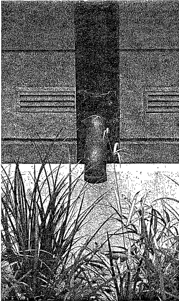
A disconnected roof downspout spills into a bioretention planter. Photo: Krystal Zamora
