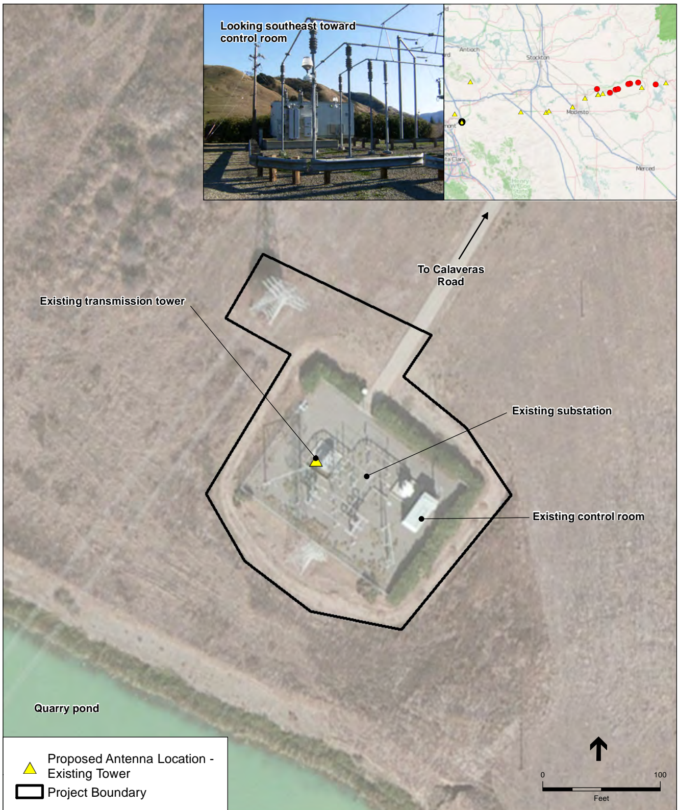
SOURCE: ESRI, 2011 San Joaquin Valley Communication System Upgrade Project Figure 2-20 Calaveras Substation (Site 20)
