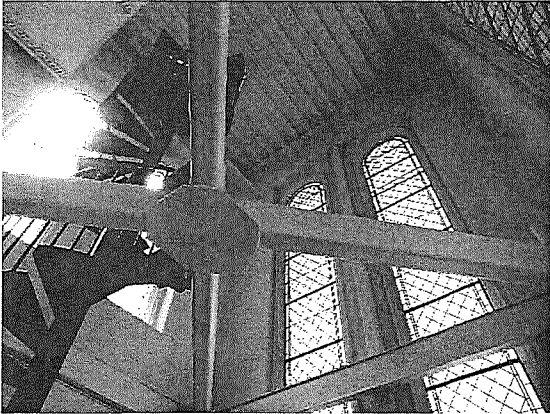
Figure 28. West tower, featuring seismic bracing and a spiral staircase. Source: Page & Turnbull, April 2019.
