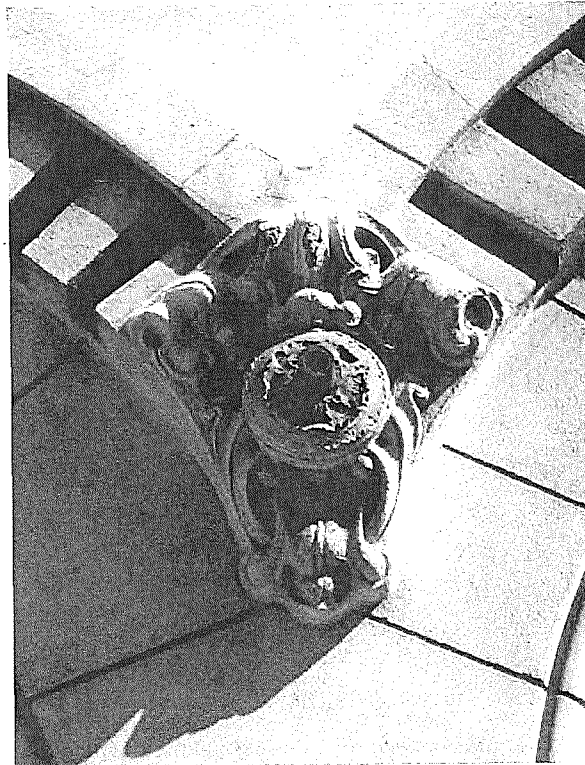
Figure 35b. Detail, original mounting hardware is all that remains in place.
