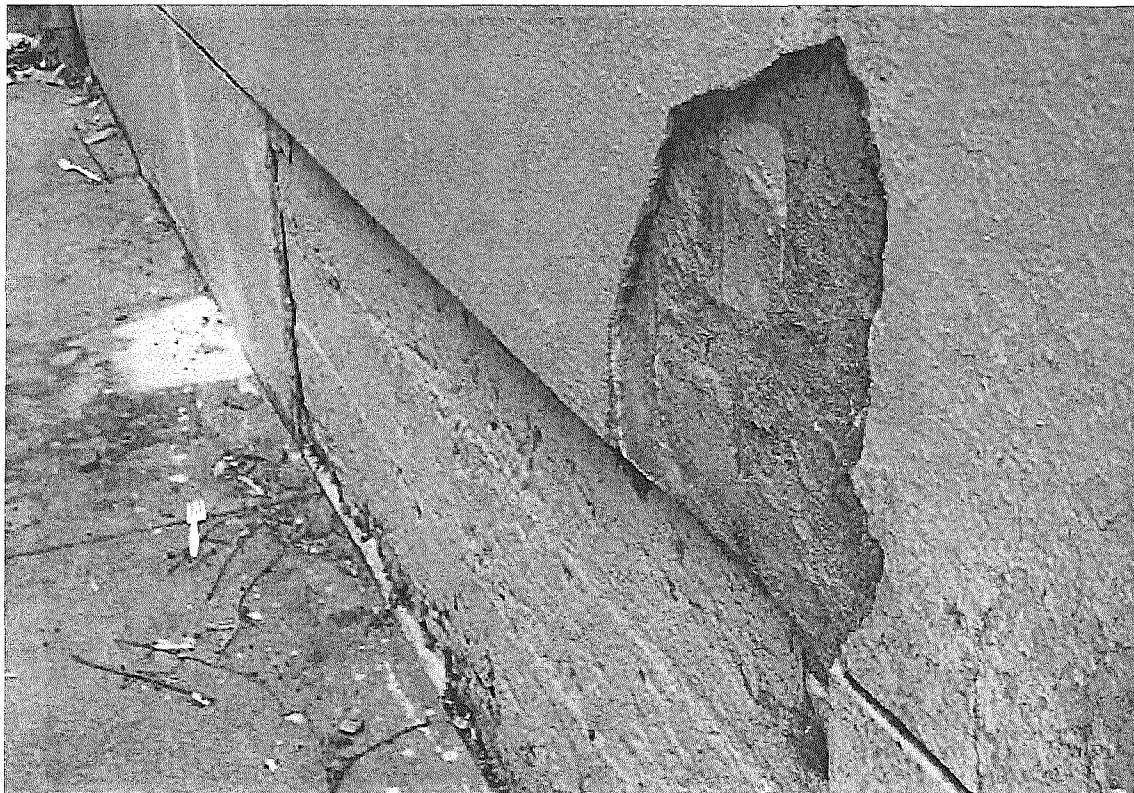
Figure 34b. East tower, north façade, showing loss of stucco at ground level.
