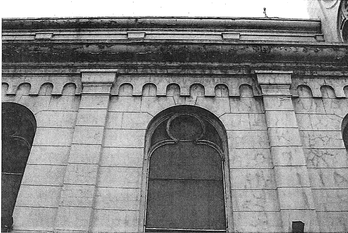
Figure 34a. East nave façade, showing soiling, water staining and hairline cracking of stucco.
