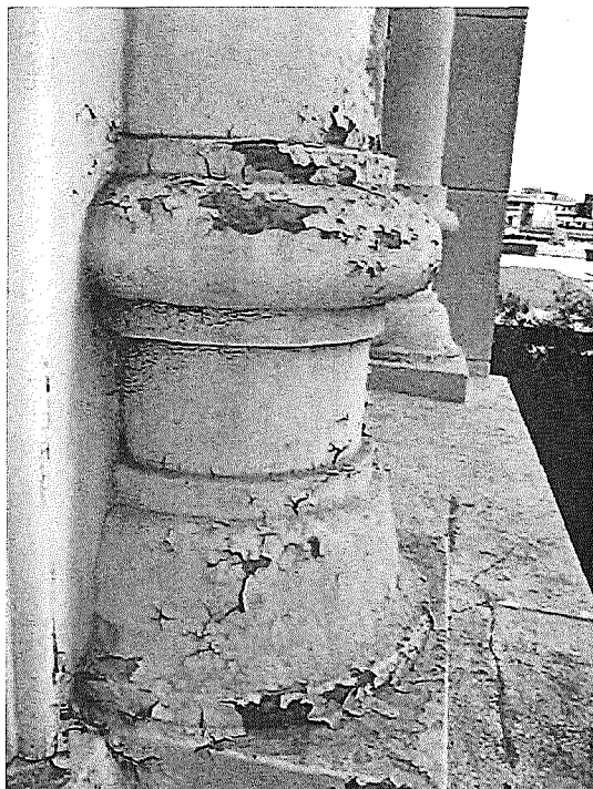
Figure 37a. Column base, south side of east tower, showing flaking and loss of protective paint layer.
