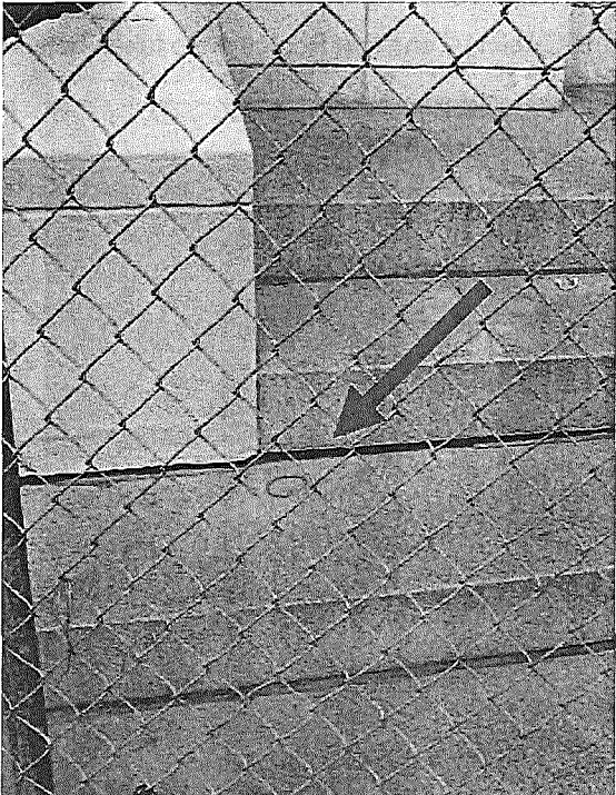
Figure 33b. Detail, east side of main portal steps, showing gap between blocks (arrow) due to uneven settling.
