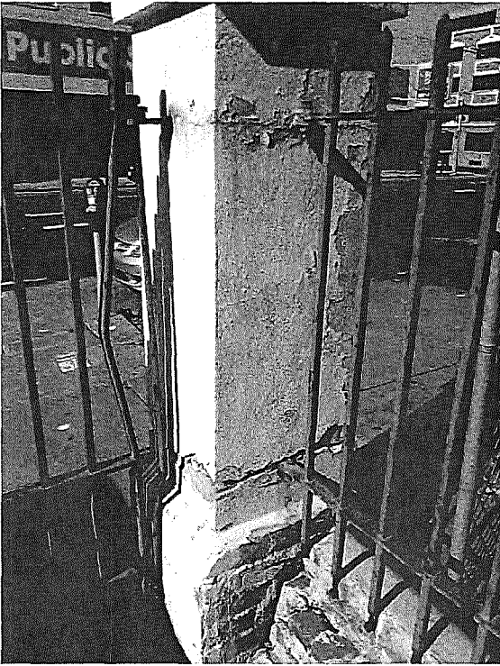
Figure 32a. Pier near west tower, showing large cracks and displaced areas of brick (arrow) and corroded metal fence.
