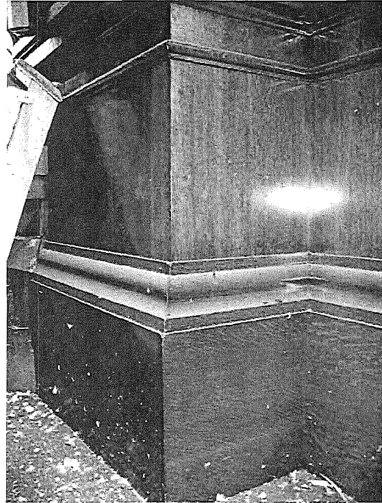
Figure 41b. Dust (on molding) and paint/guano spatters can cause permanent damage to wood finish.
