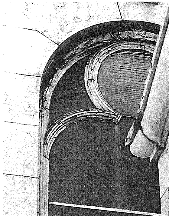
Figure 38b. East façade, transept window, showing soiling, paint loss and rotting/loss of tracery elements.
