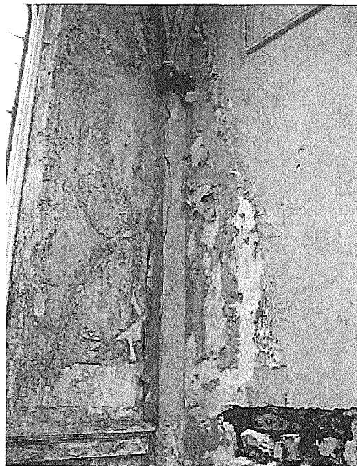
Figure 40d. Structural cracking and separation of plaster details from masonry substrate caused by moisture from blocked drains.
