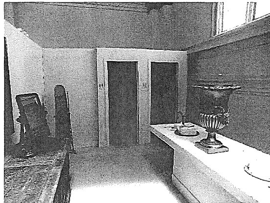
Figure 27. Restrooms, including a marble alter converted to sinks, on the mezzanine level of the east transept. Source: Page & Turnbull, April 2019.
