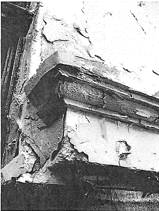
Figure 40c. Softening and deterioration of decorative plaster elements caused by moisture from faulty roofing.
