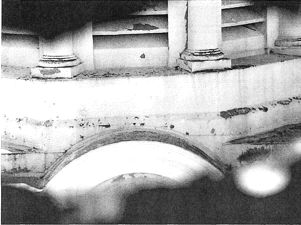
Figure 36a. Detail, rust-through at painted sheet metal cupolas.
