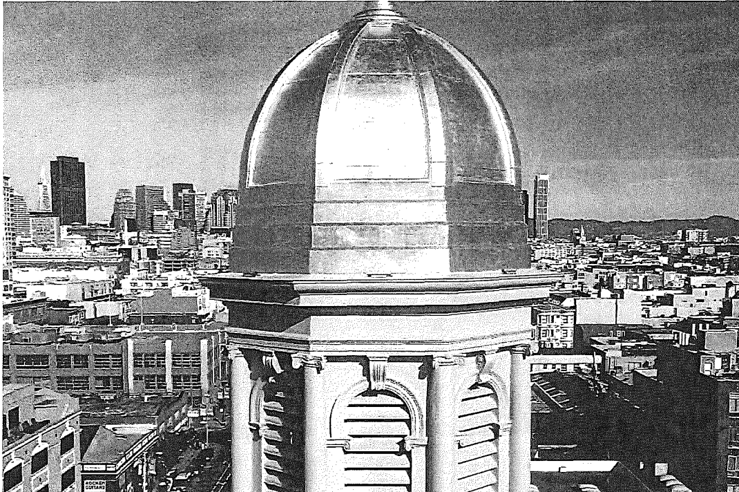
Figure 55. Gilded sheet metal dome and top of sheet metal cupola. (Palisade Builders, 05/20/2018)
