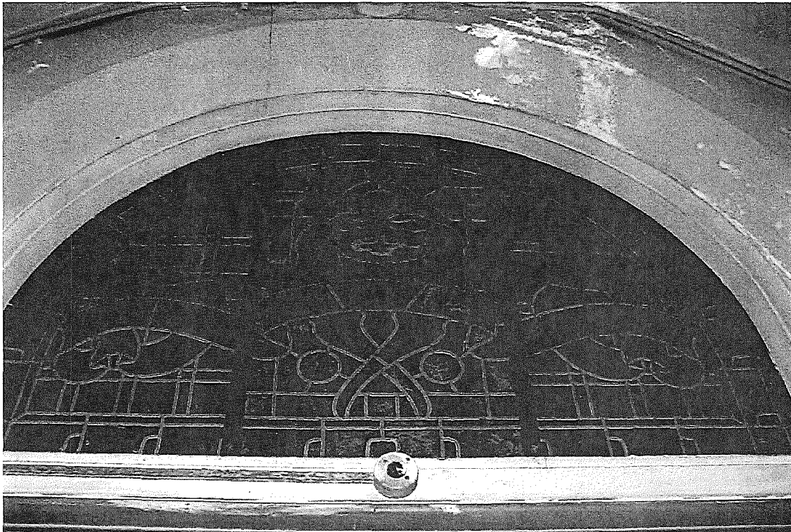
Figure 42a. North-east transept portal, showing blocked figurative stained glass window with heavy soiling and corrosion of steel frame
