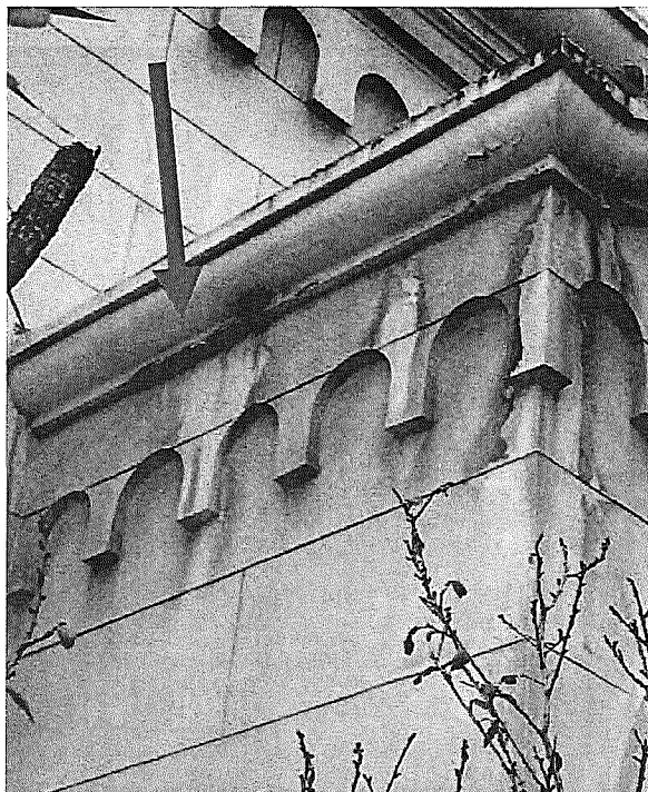
Figure 37b. Cornice above north portal, east transept, showing perforation (arrow) of the metal due to corrosion.
