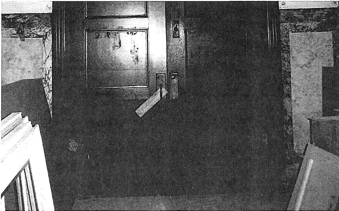
Figure 39a. Marble wainscoting of the narthex, showing soiling of the baseboard, wear of polished surface, and adhered tape. Original marble floor was covered with vinyl tile.
