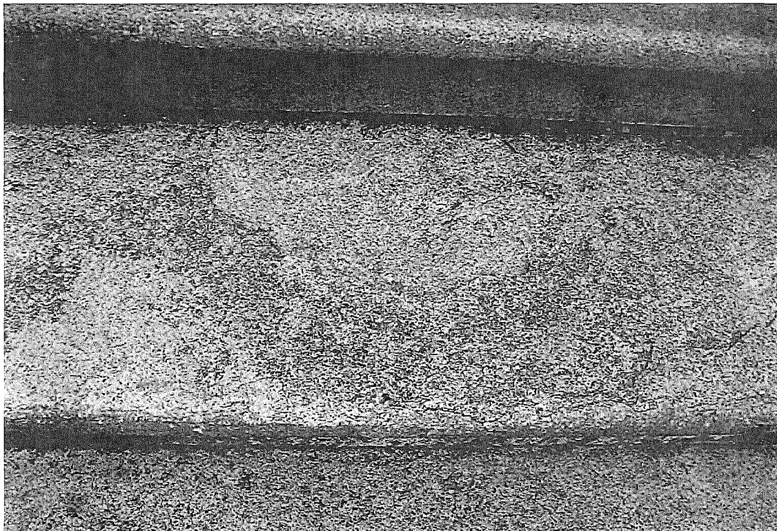
Figure 33e. Detail, south portal steps, spalled surface of granite tread.
