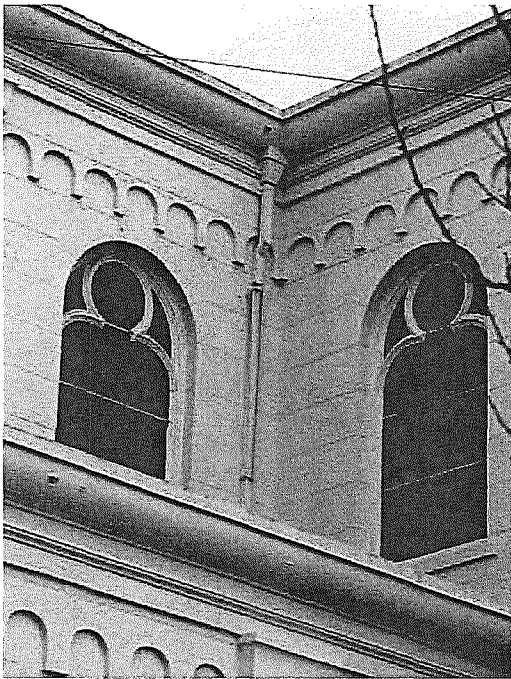
Figure 40a. West façade, showing blocked or perforated drainage which is causing damage to interior plaster.
