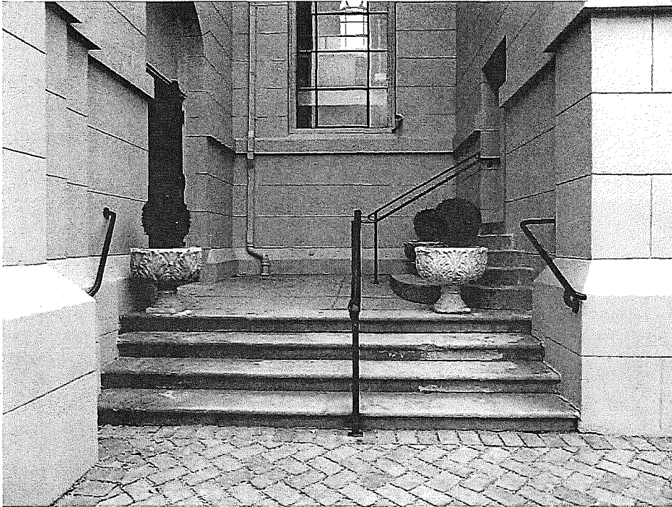
Figure 49. Exterior landing on west façade between west transept and sacristy. (Page & Turnbull, 05/25/2018)
