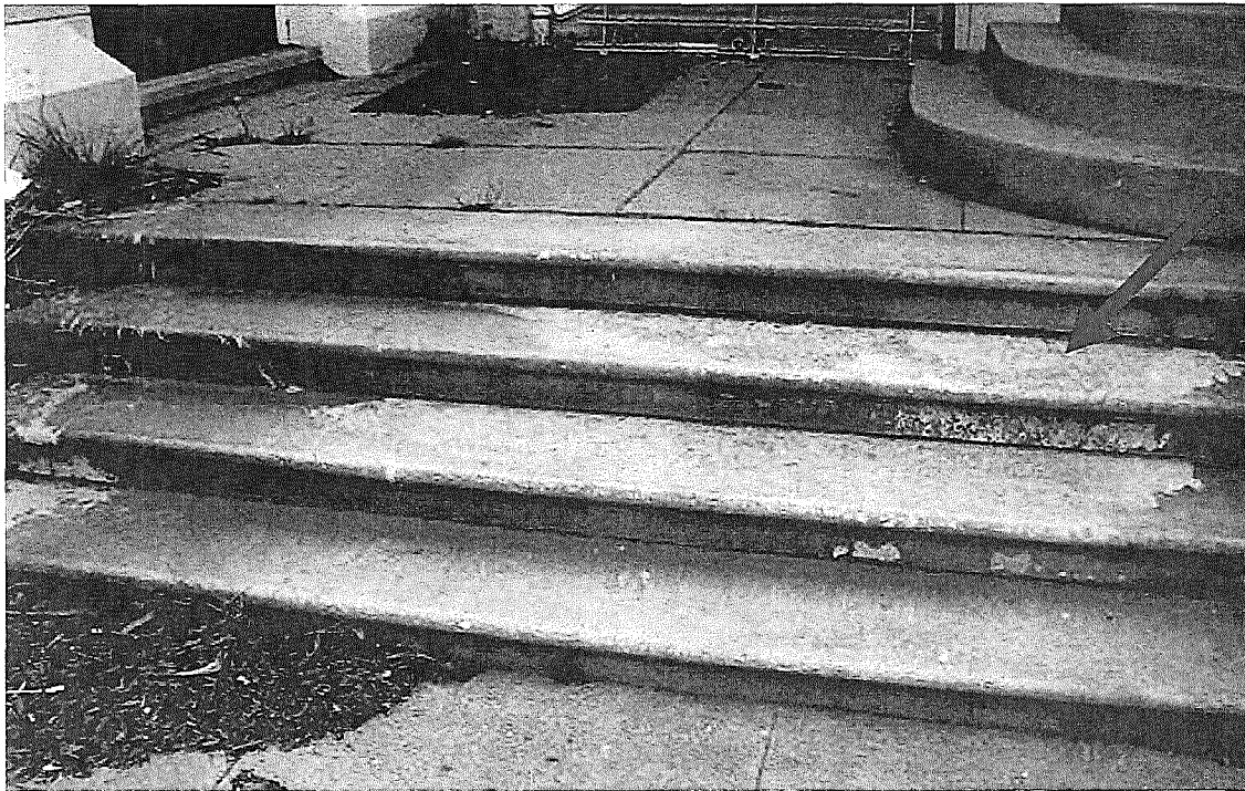
Figure 33d. West transept, south portal steps, showing paint stains (left), soiling and spalling surface (arrow).
