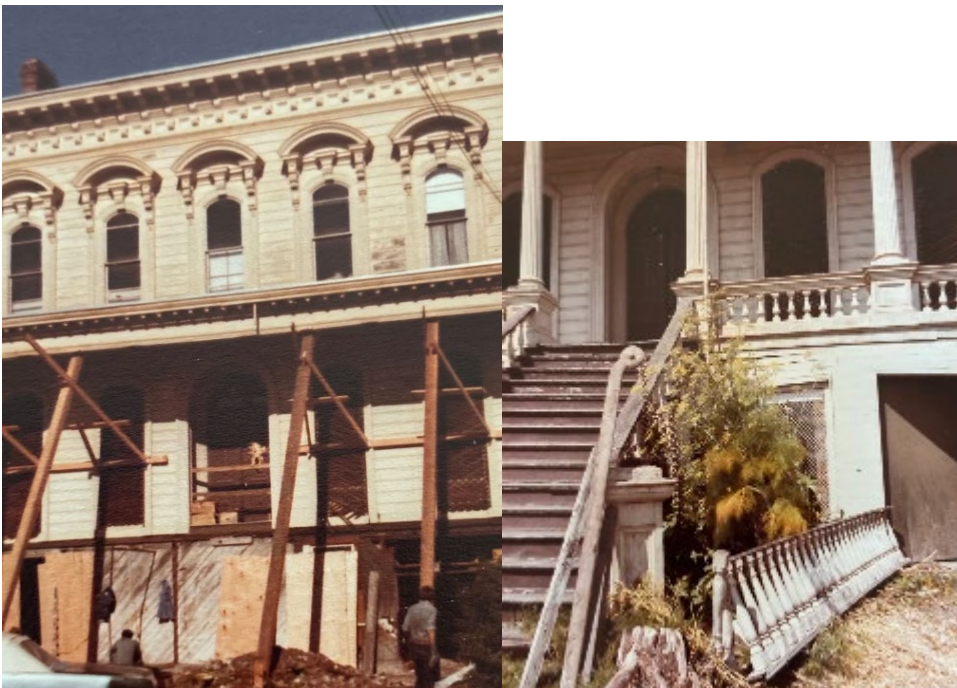
Blacketer-Sylvester House, 1556 Revere Avenue, deteriorated front façade features and with front porch removed, c. 1978.
