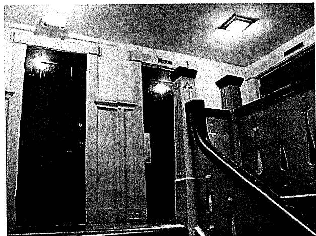
Second floor landing. From left to right a closet, men’s room and double doors leading to the Freja Hall ante room. Both the closet and men’s room were removed in 2014 to install an ADA compliant elevator.
