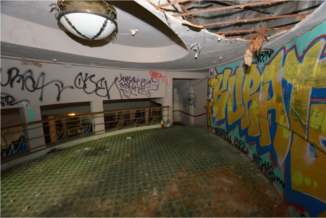
Upper lobby. Note decorative metal and wood handrail at left and ceiling mounted light fixture top left.
