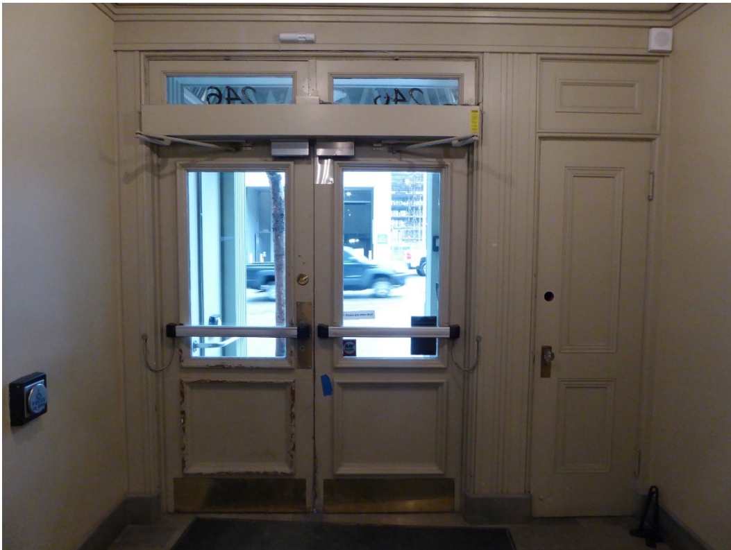
A17. View of vestibule and closet inside south entry, looking east (ARG, February 2017).
