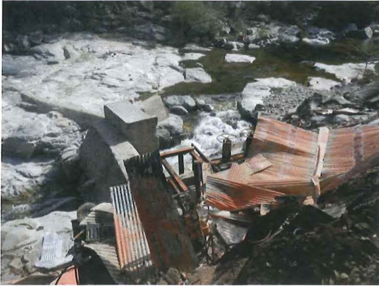
Destroyed Buildings at Head Gates
