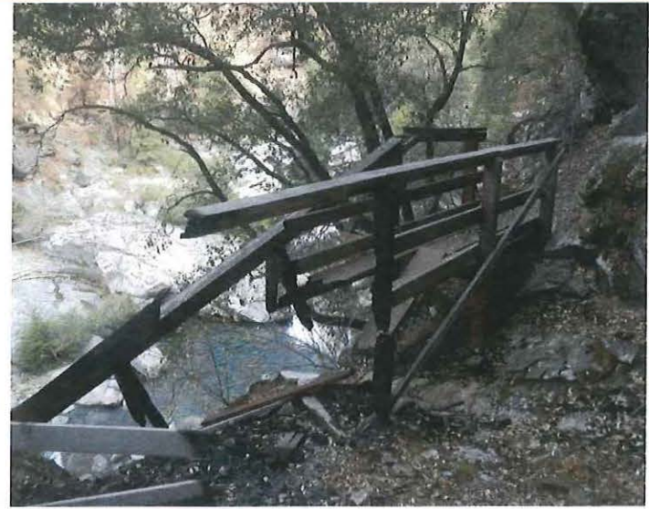
Damaged Pedestrian Bridge
