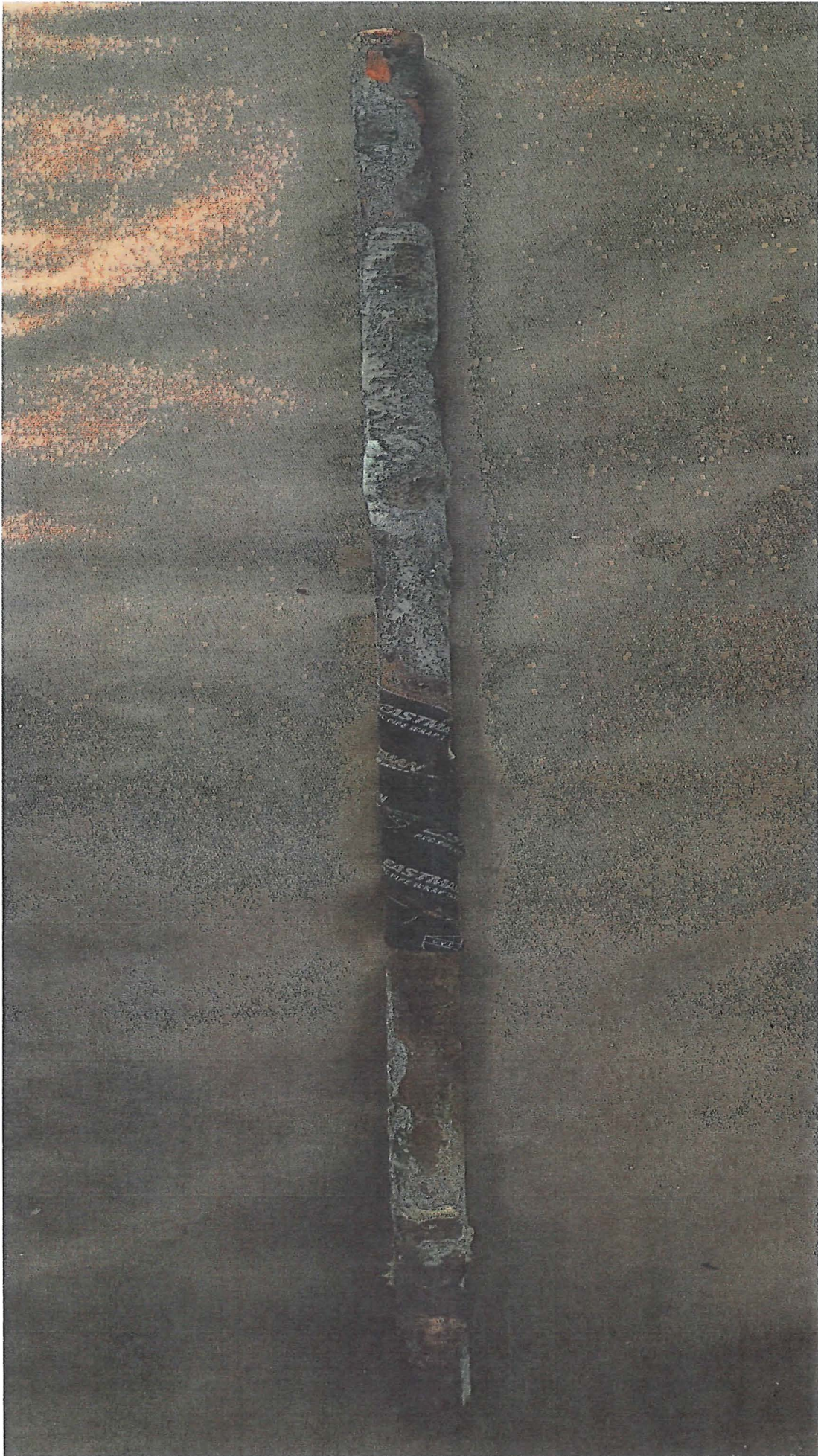
A copper water pipe from the subject area Influenced by salt water and lead contamination
