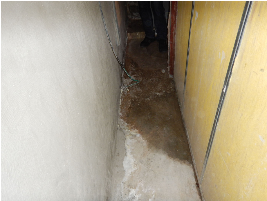
Photo 6: Efflorescence on wall base and water on floor adjacent to equipment (left side).
