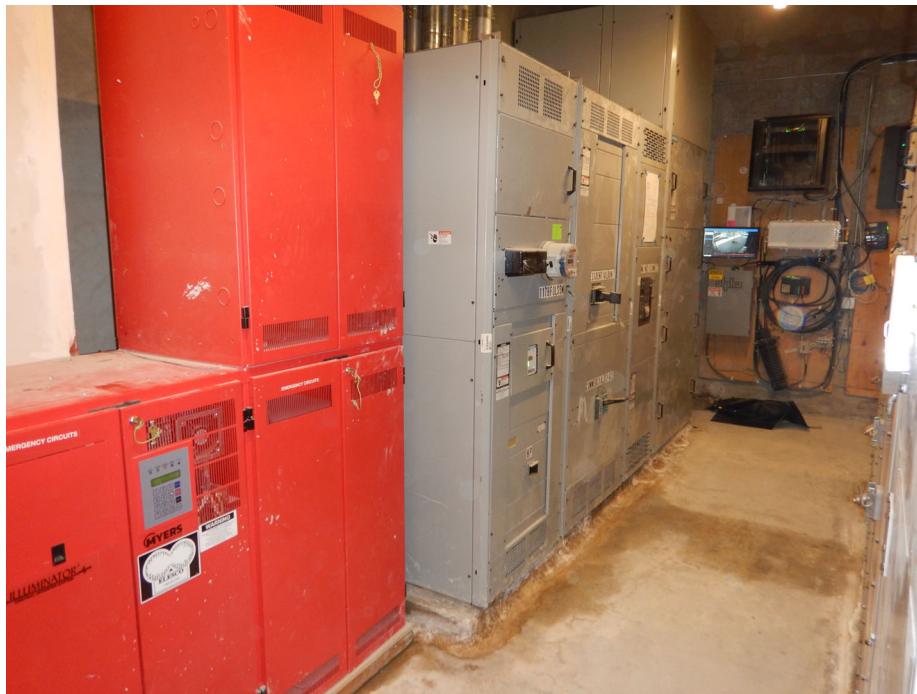
Photo 1: General view of electrical equipment. Note water on floor.
