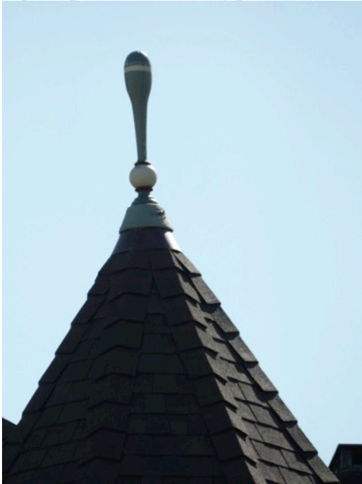
Figure 14. Detail of turret roof and spindle. (Photograph by Garavaglia Architecture, Inc., April 2015.)
