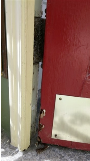
Figure 24. Rotted wood at entrance portico door. (Photograph provided by Côme Lague, April 2015.)
