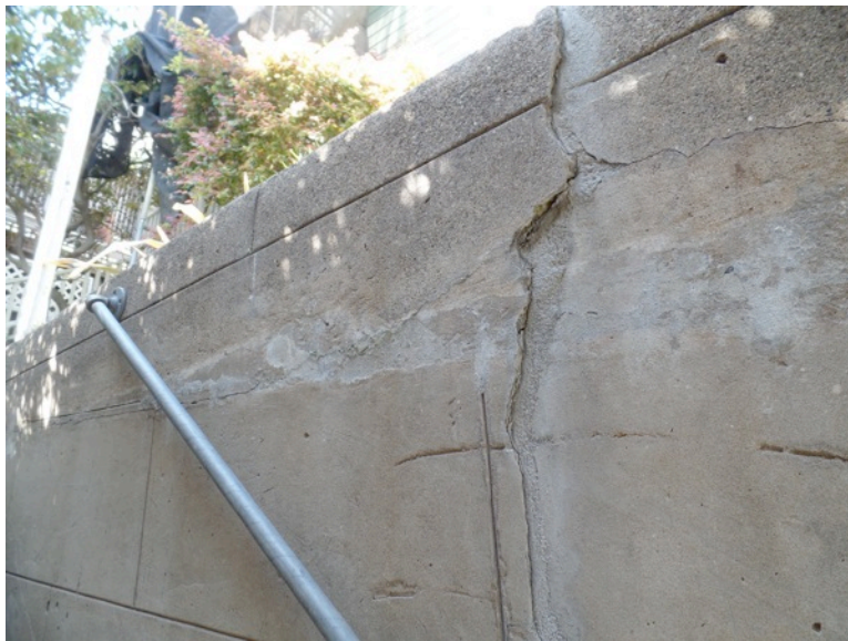
Figure 16. Cracked retaining wall along east property line. (Photograph by Garavaglia Architecture, Inc., April 2015.)
