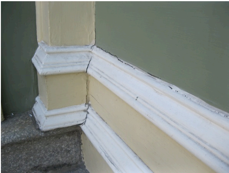
Figure 20. Peeling paint and splitting wood at west elevation. (Photograph by Garavaglia Architecture, Inc., April 2015.)
