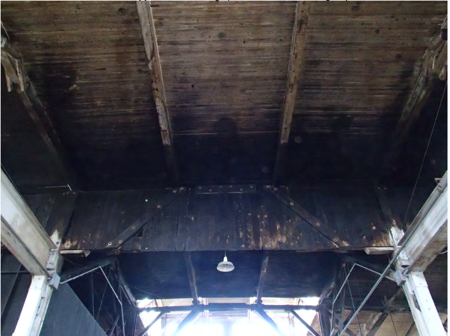
Photo 4. View of a portion of the roof displaying fire damage at the north end of the building
