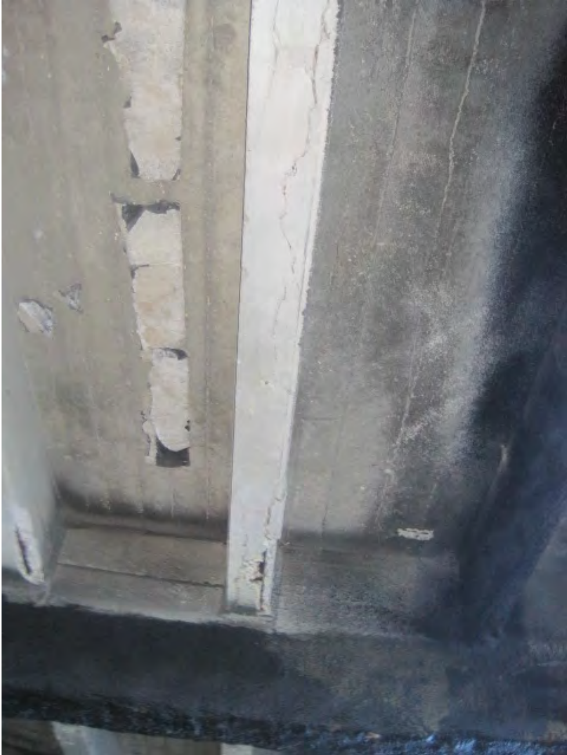
Photo 6. Concrete spalling at slab
