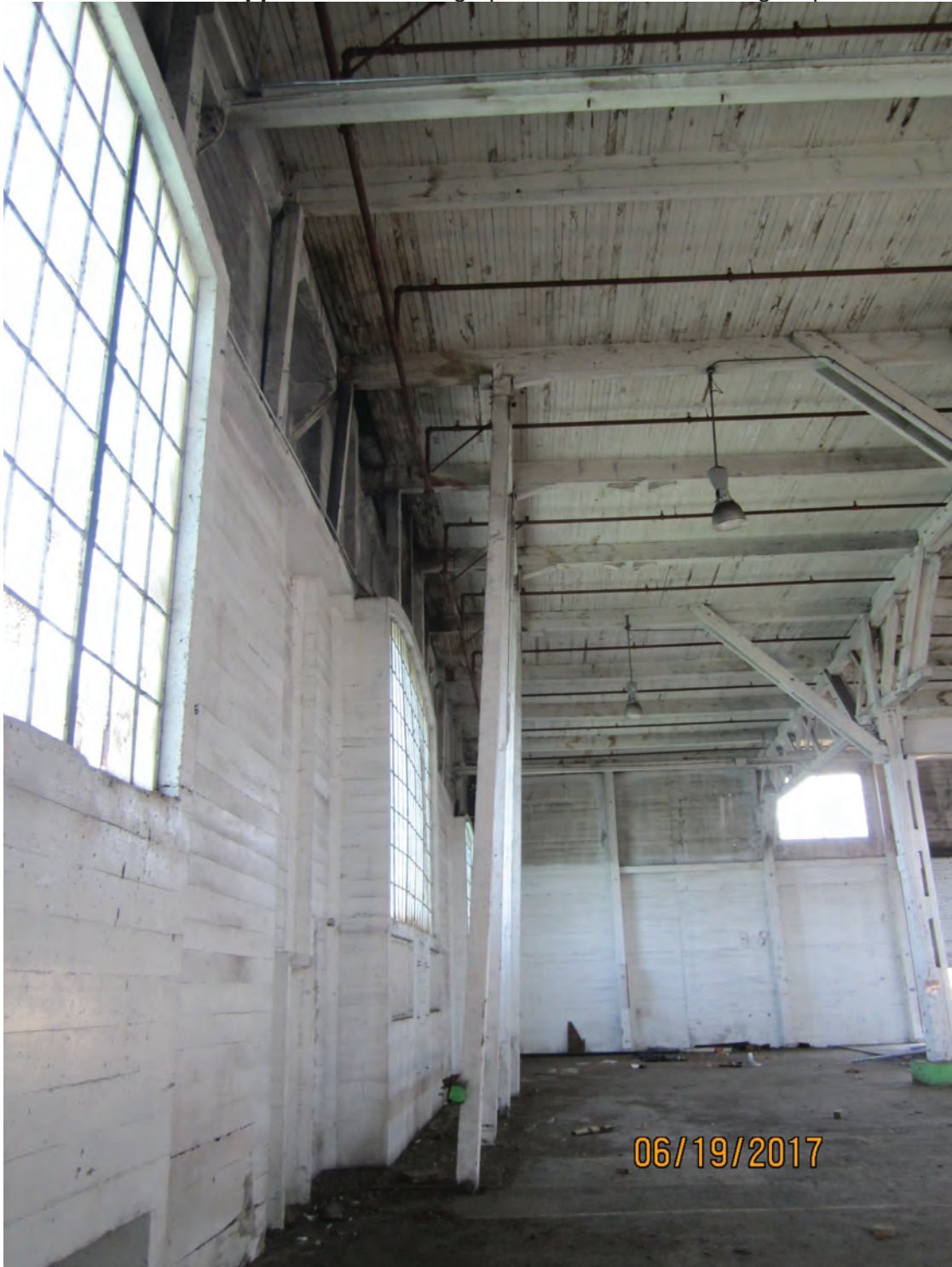
Photo 13. Shoring posts under roof beams near rear wall. Posts are keyed into substructure concrete slab.
