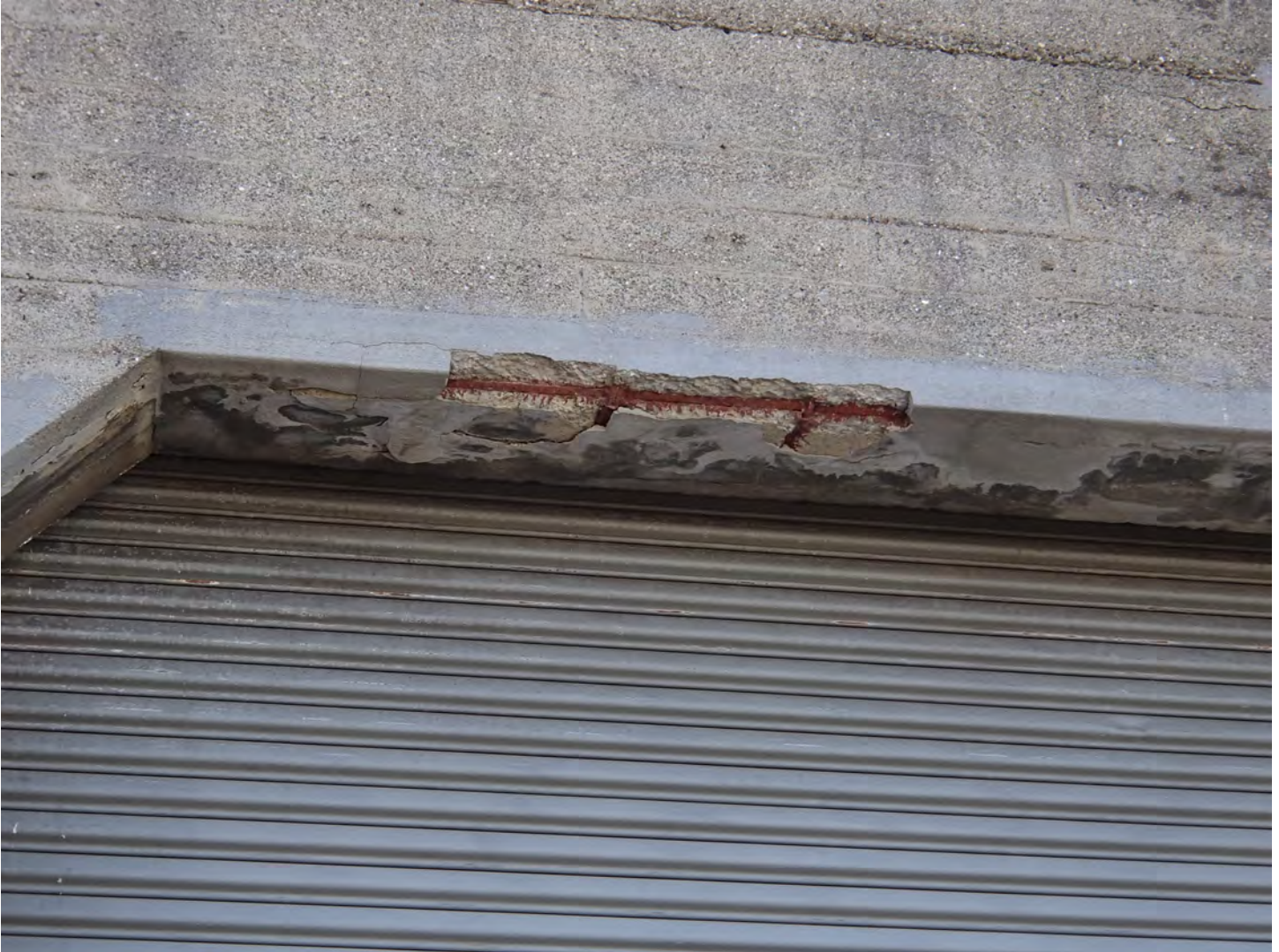
Photo 3. View of the concrete spalling at door openings at east elevation
