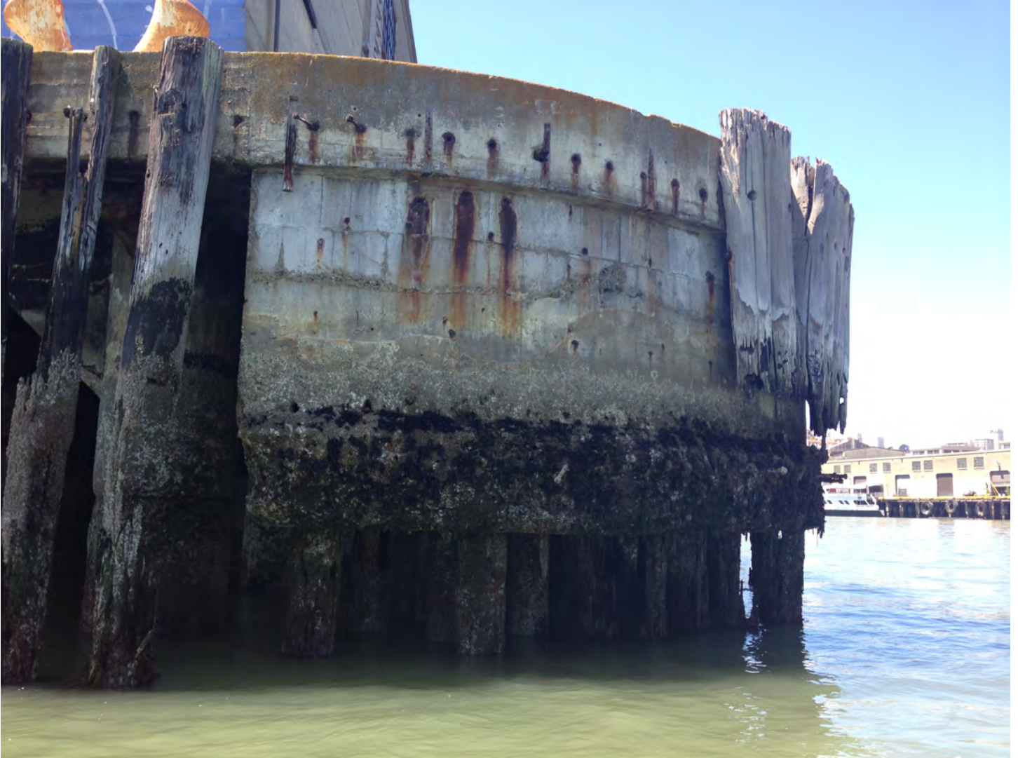
Photo 3. Deteriorated wood piles at pier corner
