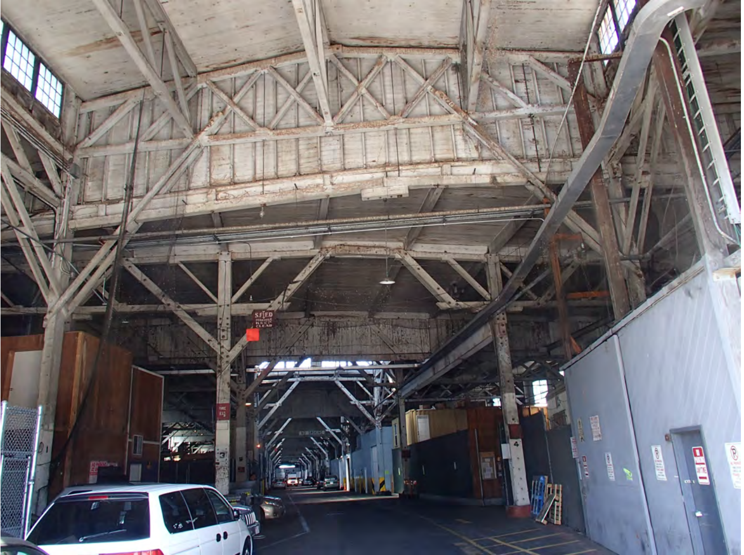
Photo 9. View of the structural framing near the interior entrance of the shed
