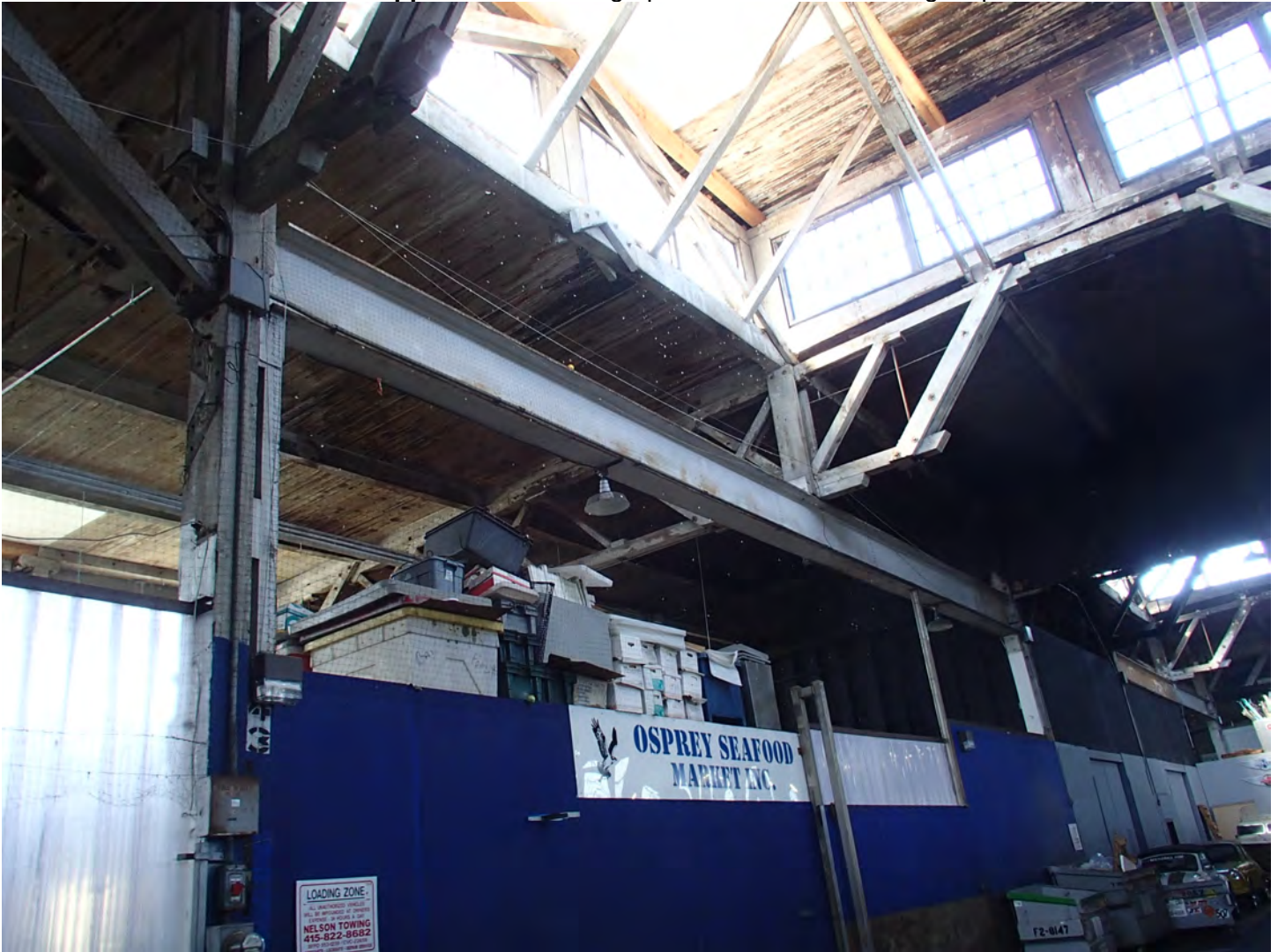
Photo 5. View of roof repair work at the fire damaged area. Note: A steel beam replaces a removed wood post due to fire
