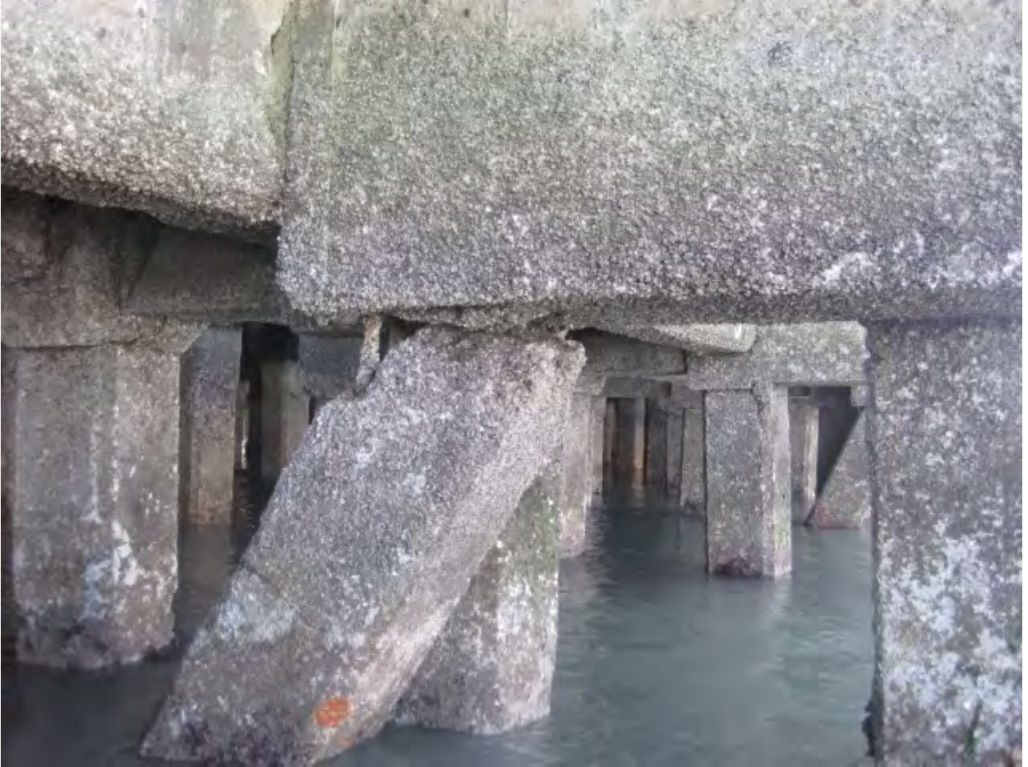
Photo 7. Broken batter pile
