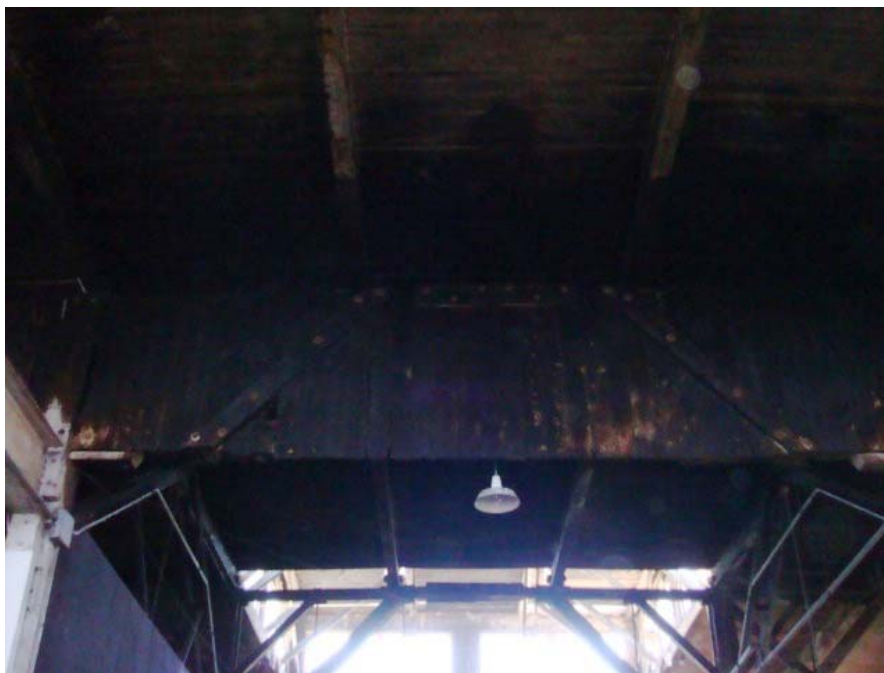
Photo 6. Fire damage at north end
