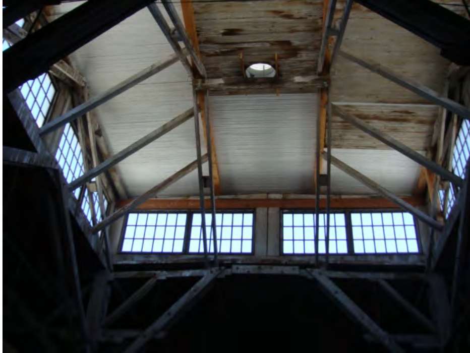
Photo 3. Roof repair work and water staining
