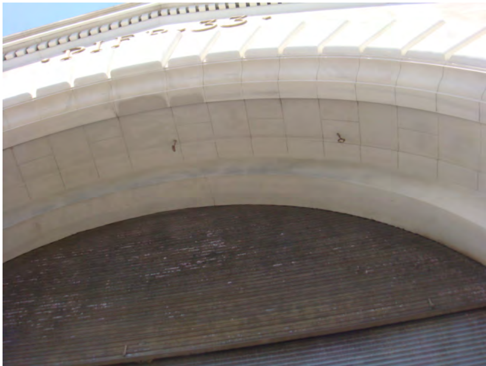
Photo 2. Rusting eye bolts
