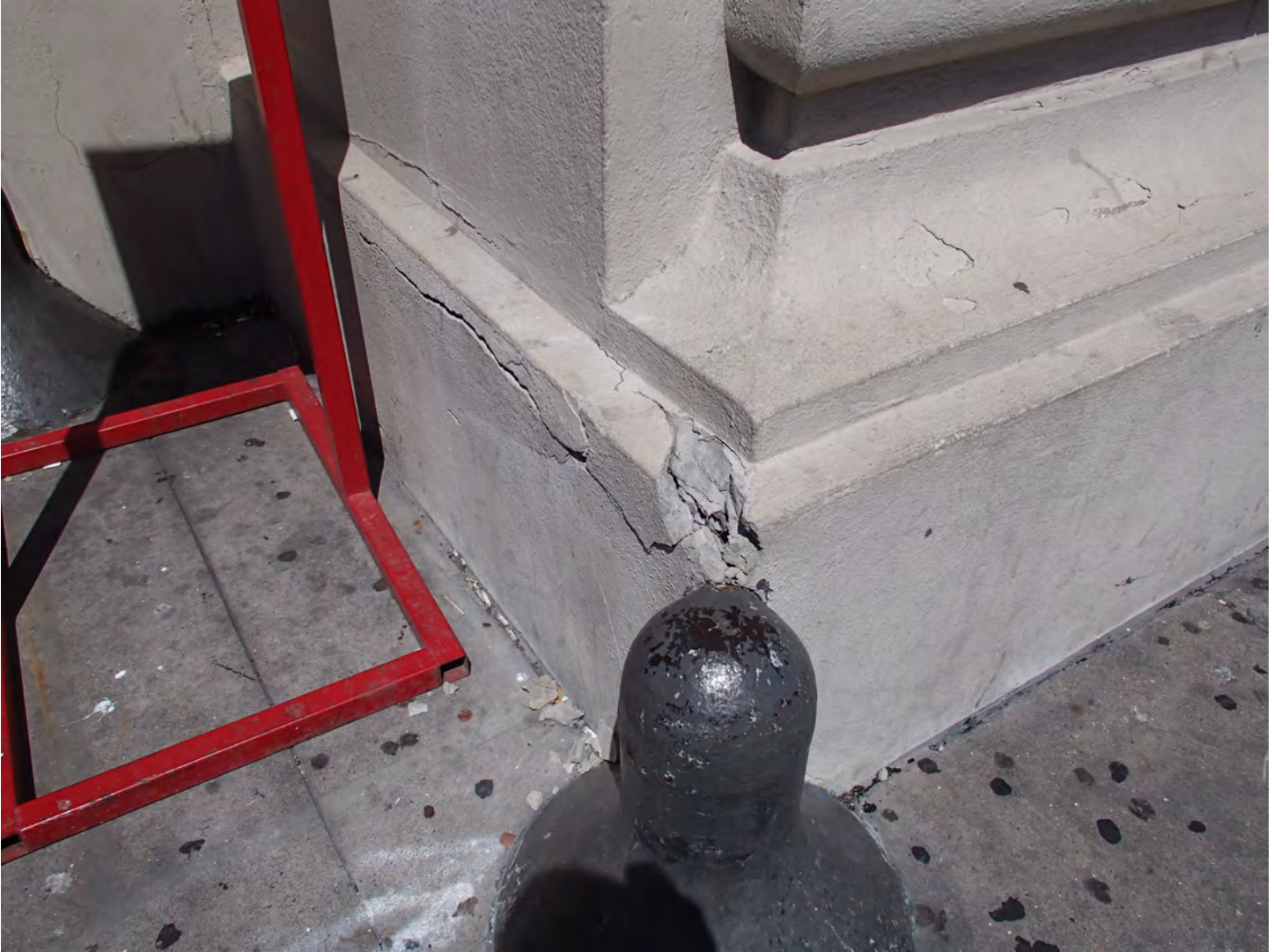
Photo 10. View of the stucco spalling in the wall base near the entrance
