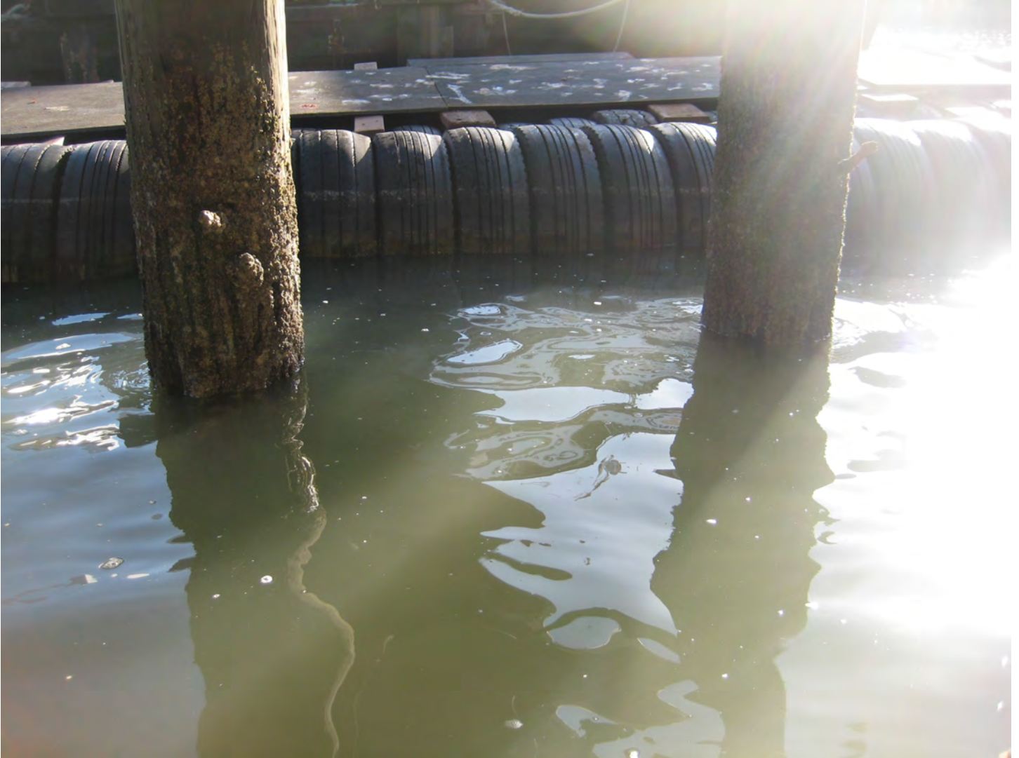
Photo 4. Deteriorated wood piles near metal deck
