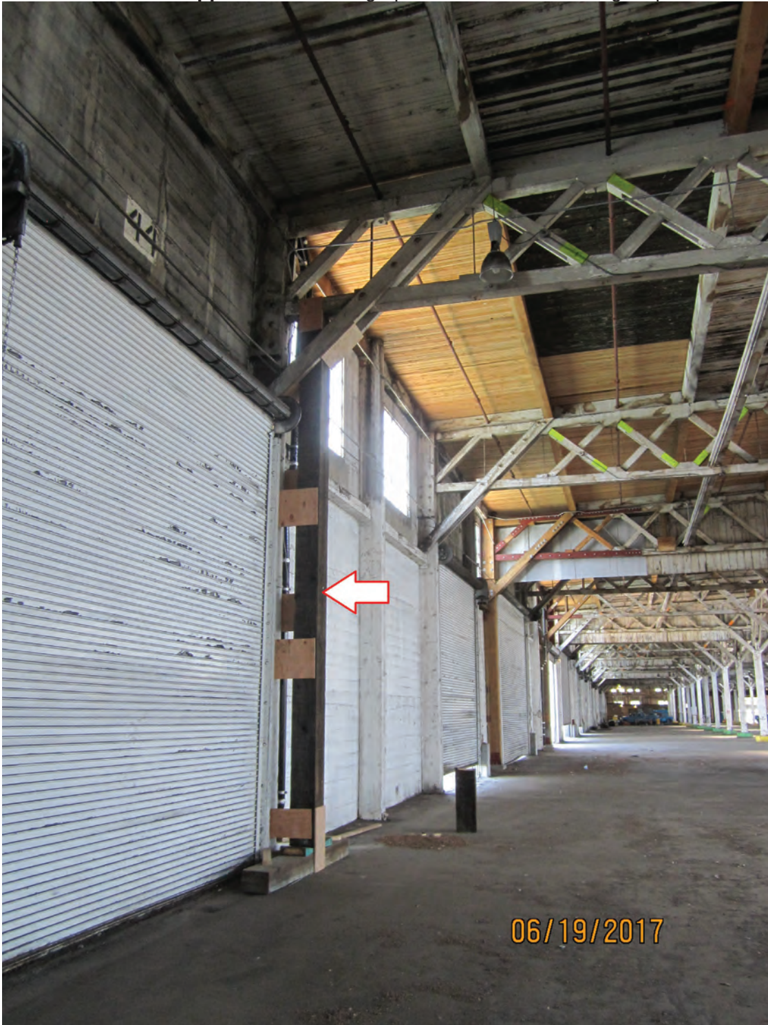
Photo 16. Shoring post installed at column grid H26 due to additional dry rot discovery. Permanent repairs are already planned. Similar shoring at B14 and B42. Roof area supported by these posts are shown yellow tagged until permanent repairs are complete.
