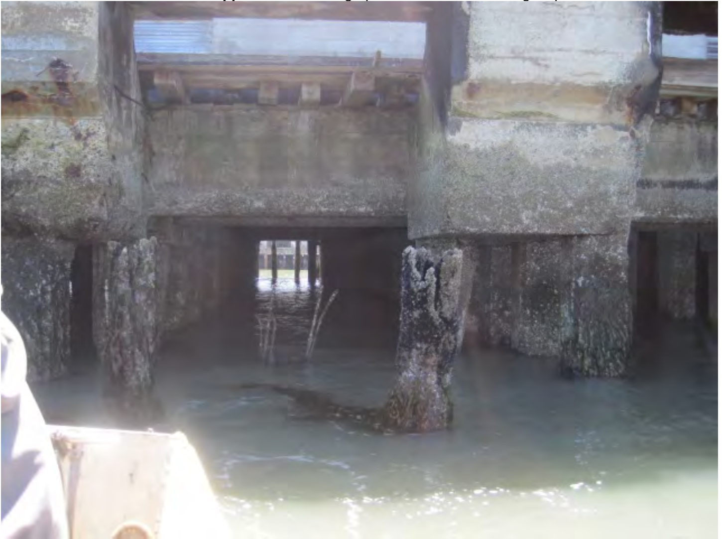
Photo 5. Deteriorated fender piles
