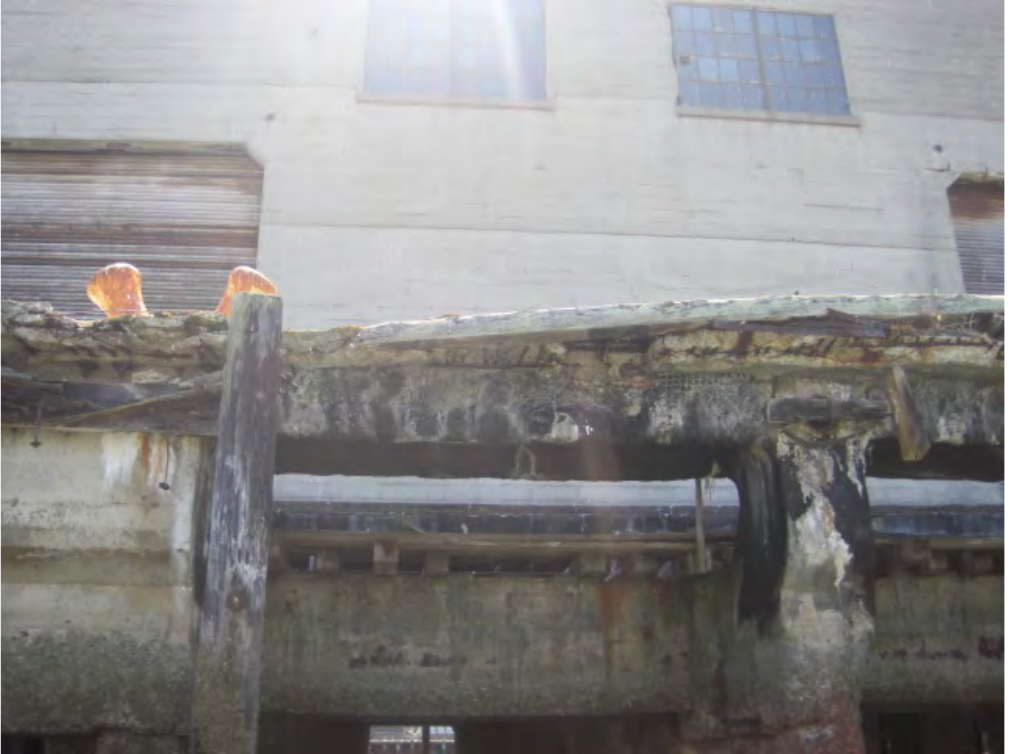
Photo 10. Spalling deck and corroded/exposed rebar
