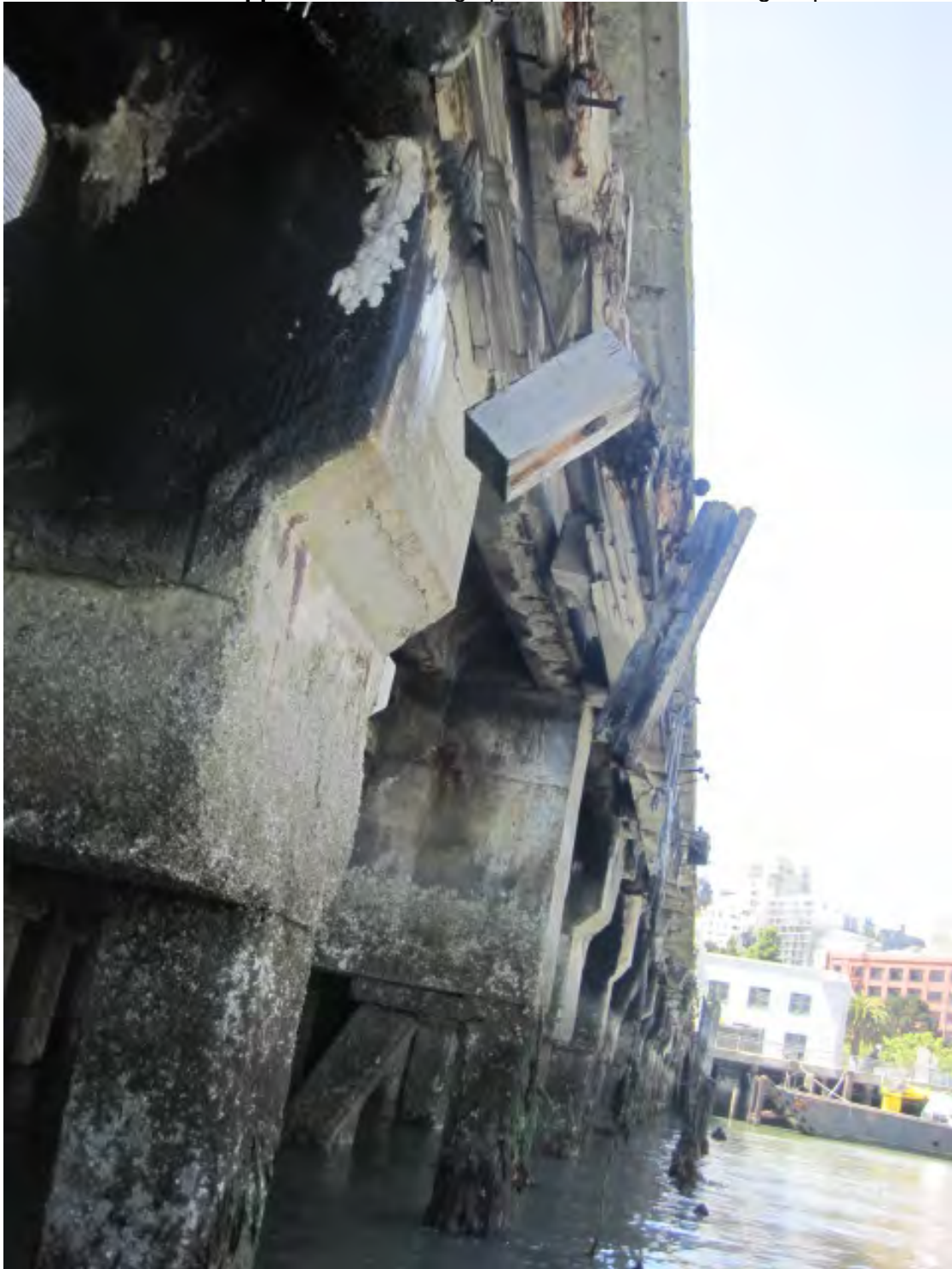
Photo 6. Hanging wood members
