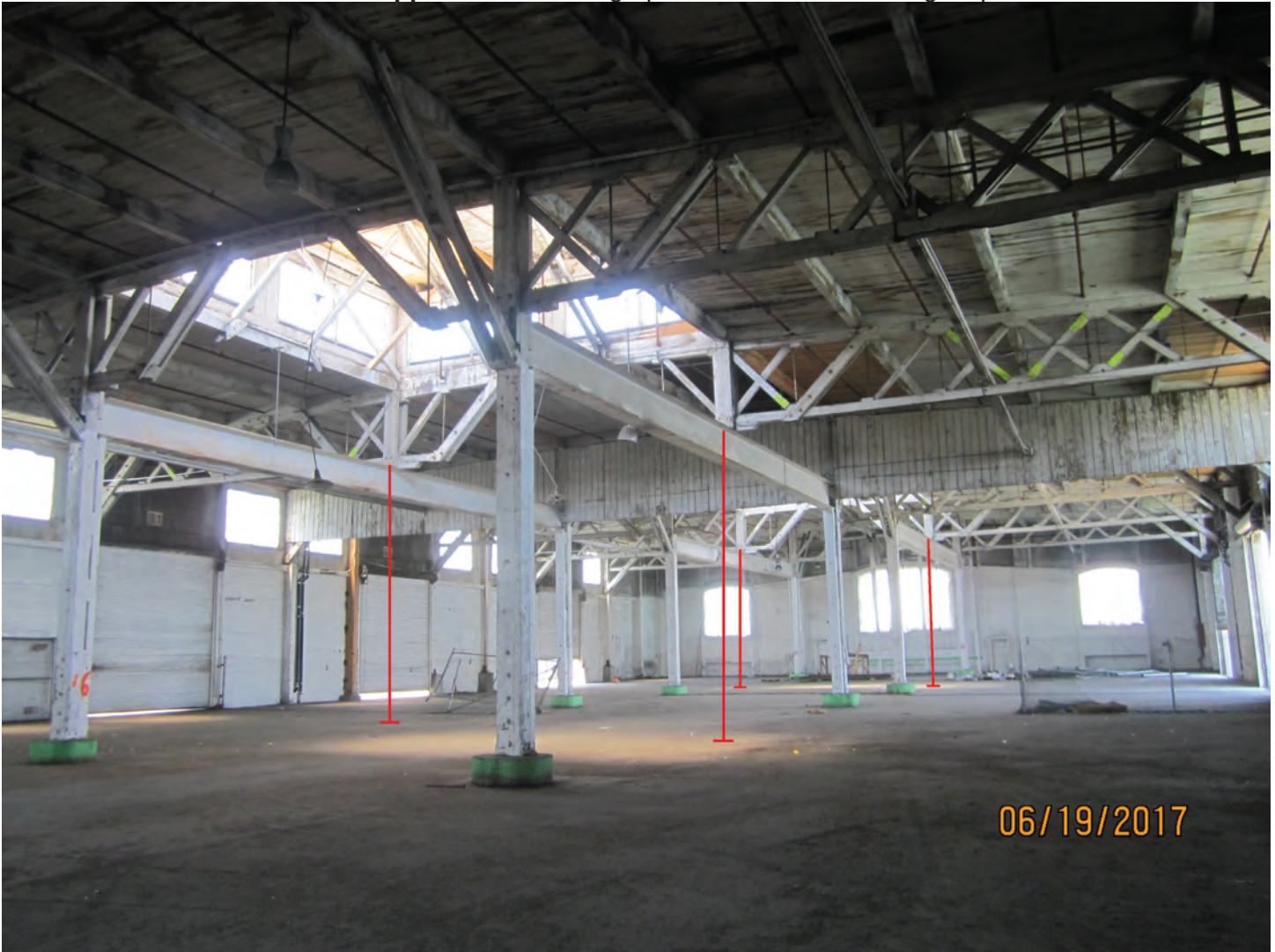
Photo 12. Steel beams and supplemental wood posts added in the past in order to remove original columns.
