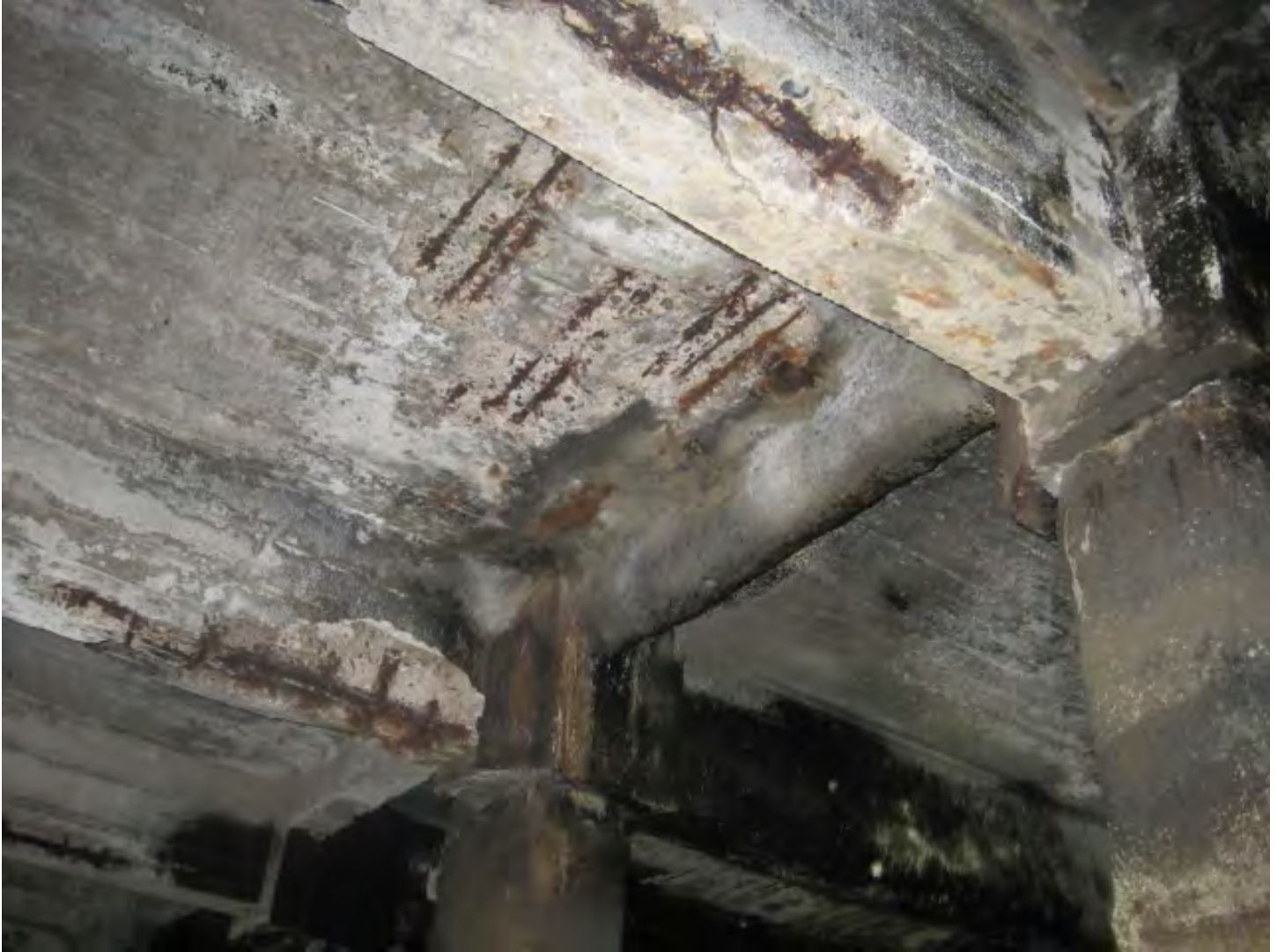
Photo 9. Spalling of concrete beams and slab
