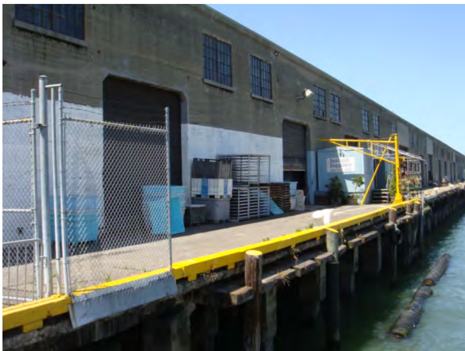
Photo 4. Concrete spalling around windows at east wall
