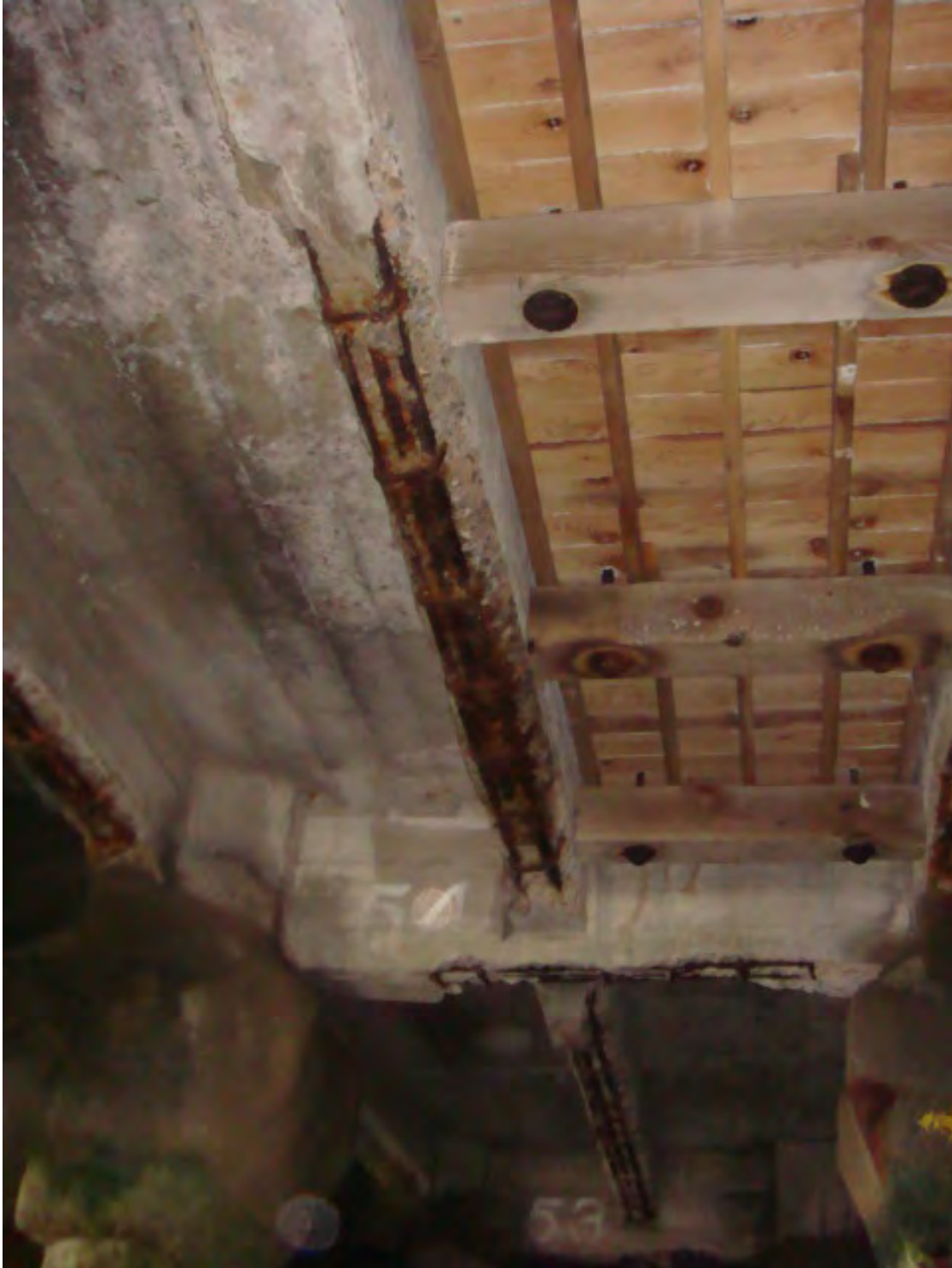
Photo 3. Concrete spalling, typical
