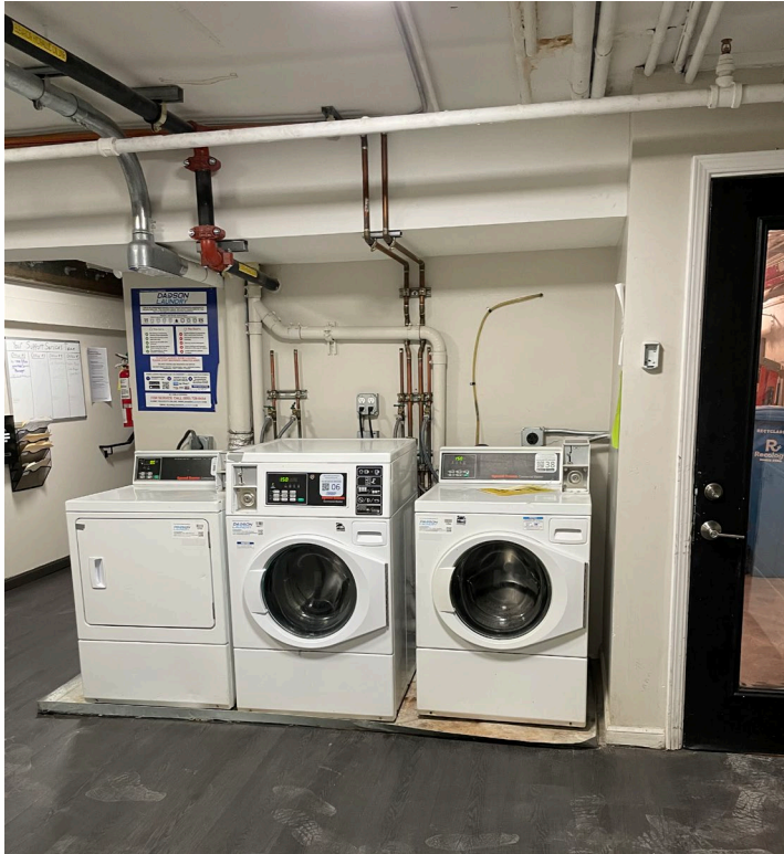
Photo: Garland Hotel, laundry
