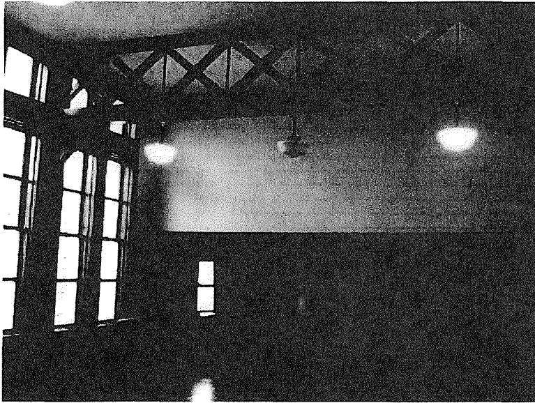
Balder Room showing trusses that will likely be replaced within 10 years.
