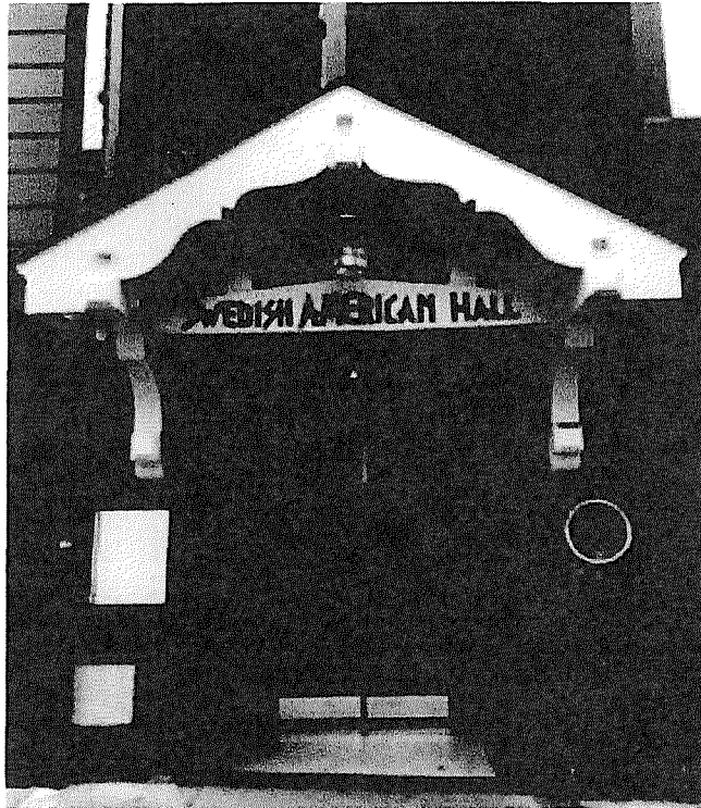
Main entry showing doors to be replaced.
