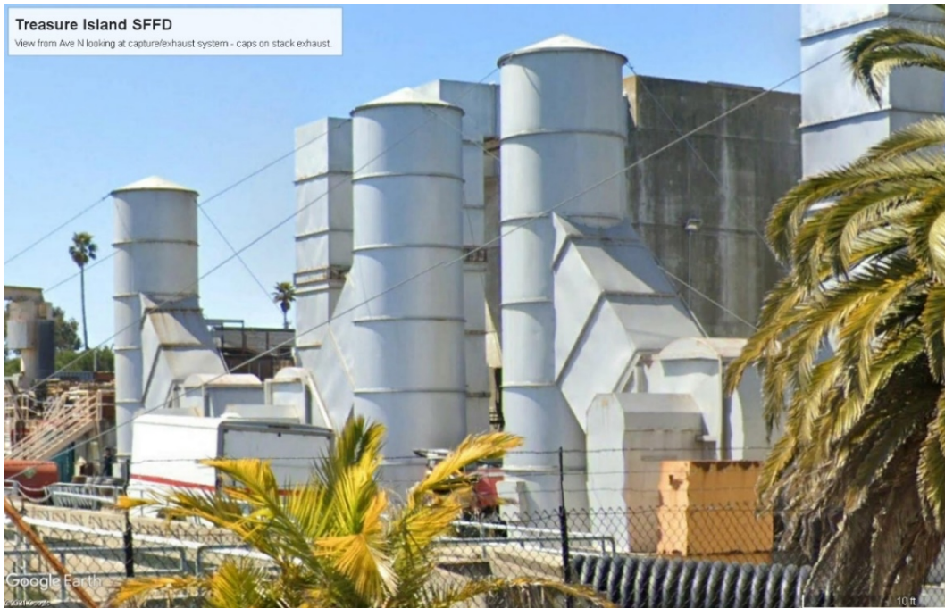
Figure 7. Existing Live-Fire Training Exhaust Capture System at Treasure Island Facility
