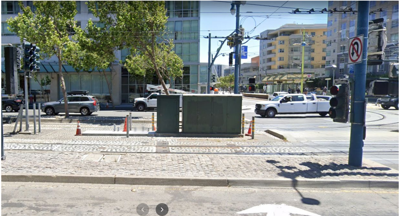
Figure 1. Example of Interlocking cabinet (left) at 4th & King streets.
