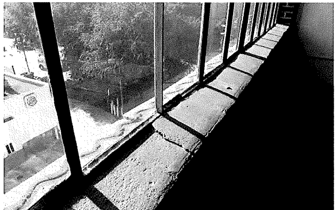
Figure 2: Concrete parge at south window sills, typical. Note level of localized cracking.
