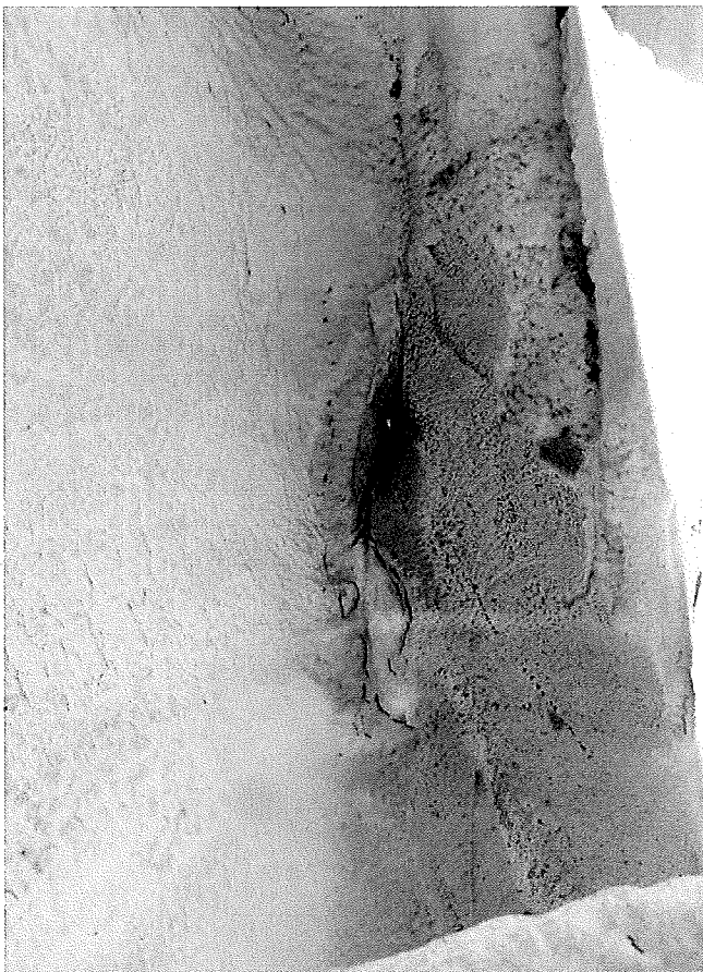
Figure 4. Detail of roofing membrane and localized damage; assess conditions throughout.
