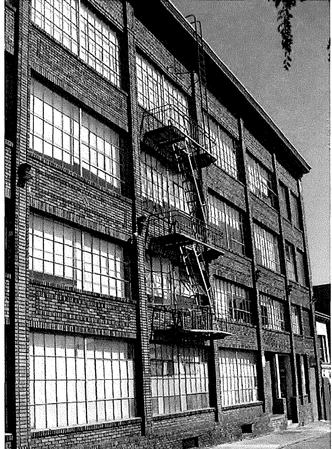
Figure 1. Metal fire escape at south elevation.
