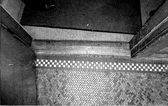
Figure 2. Threshold at wood entry door.
