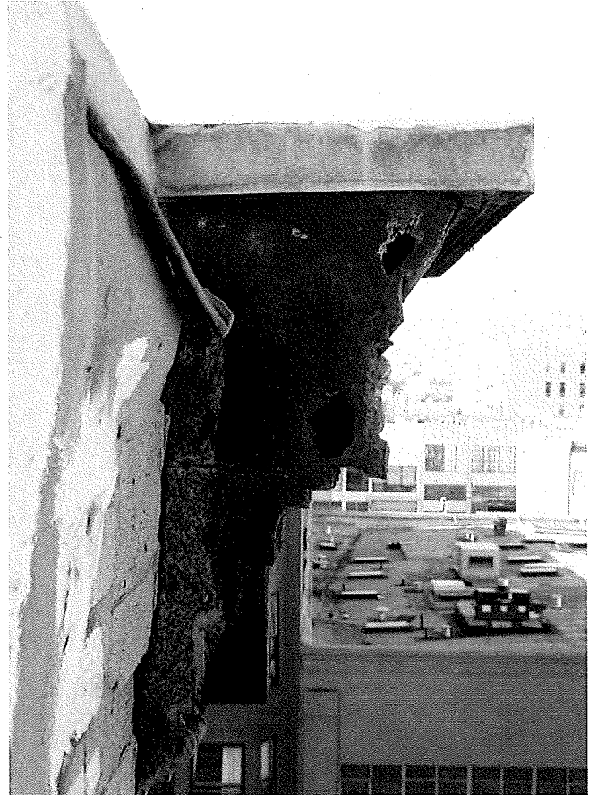
Figure 1. Cornice at northwest corner; note level of corrosion, this is worst condition observed and atypical of overall cornice.
