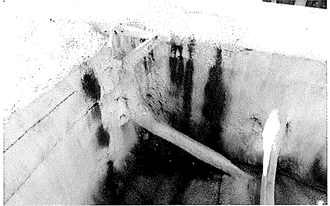
Figure 5. Bio-growth and water stains at roof. Investigate to if determine localized water damage exists.
