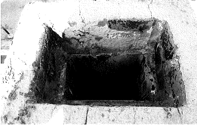
Figure 2. Open ventilation stack on north wall; cover with sheet metal as needed.
