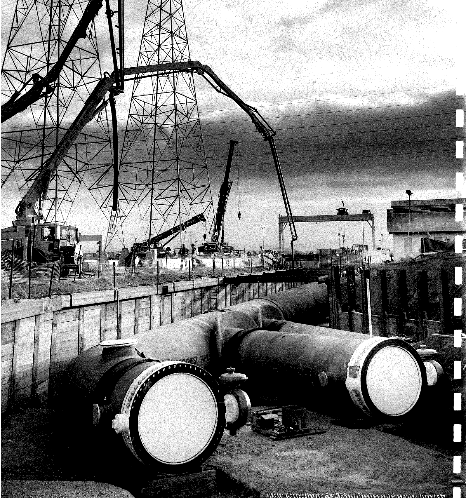
Photo: Connecting the Bay Division Pipelines at the new Bay Tunnel site.
