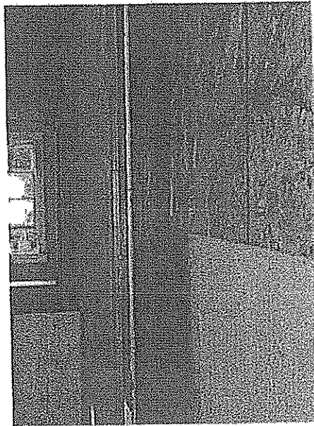
Image 20. Detailed view of former window at west wall of upper floor. Photo Frederic Knapp, 2007.
