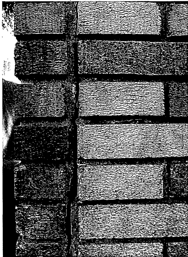
Figure 4. Southwest pier; note cracking and mortar conditions for re-pointing.
