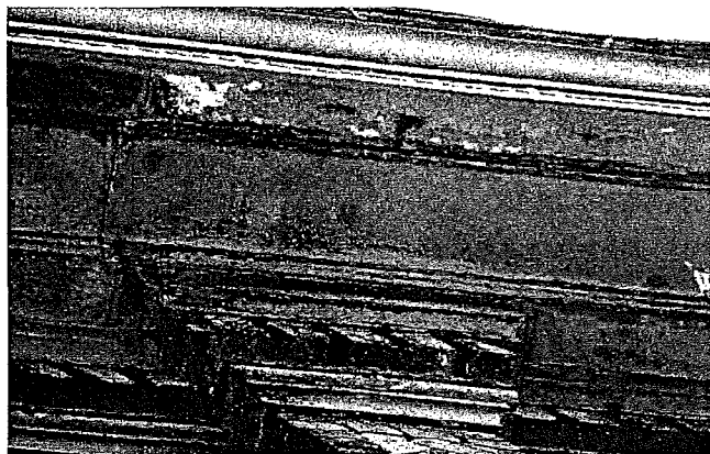
Figure 4. Cornice; conditions noted as typical.
