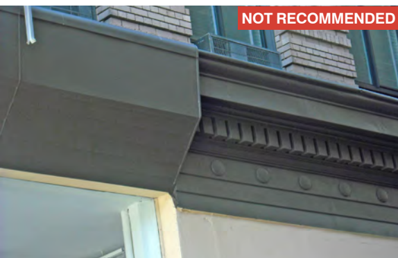
Removing, obscuring, or damaging historic features through installation of new features is discouraged, such as this historic beltcourse partially concealed with an aluminum panel.
