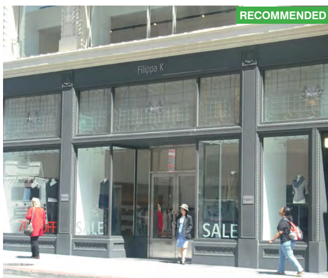
These contemporary entry doors have been located within the historic storefront. Original cast iron elements such as columns, bulkheads and the prism glass transoms have been restored. This treatment is recommended.
