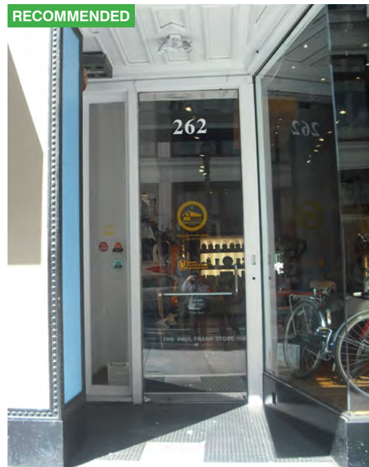
The historic wood panel ceiling in this recessed entry is historic and should be retained.
