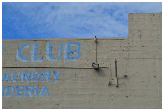
Figure 7. Flat parapet roof projection with painted sign advertisement, located at the south façade, facing north
