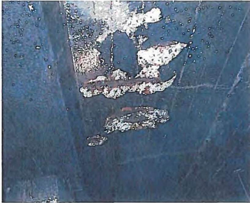
Photo 5--Deterioration in concrete slab under sheds
