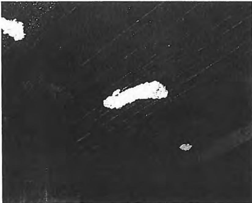
Photo 2--Substructure Deck under sheds (A and B)--areas repaired in past for minor spalls
