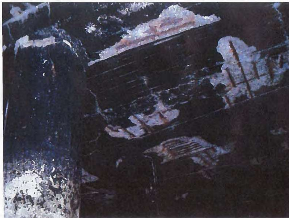
Figure 20: Spalling at deck
