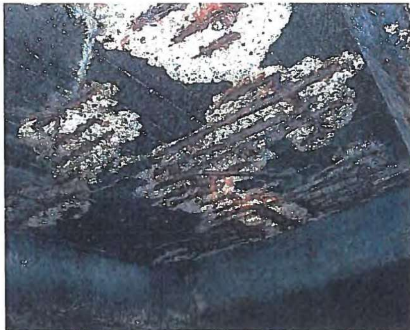
Photo 5--Deterioration in concrete slab-substructure between sheds A and B-- (typical throughout)
