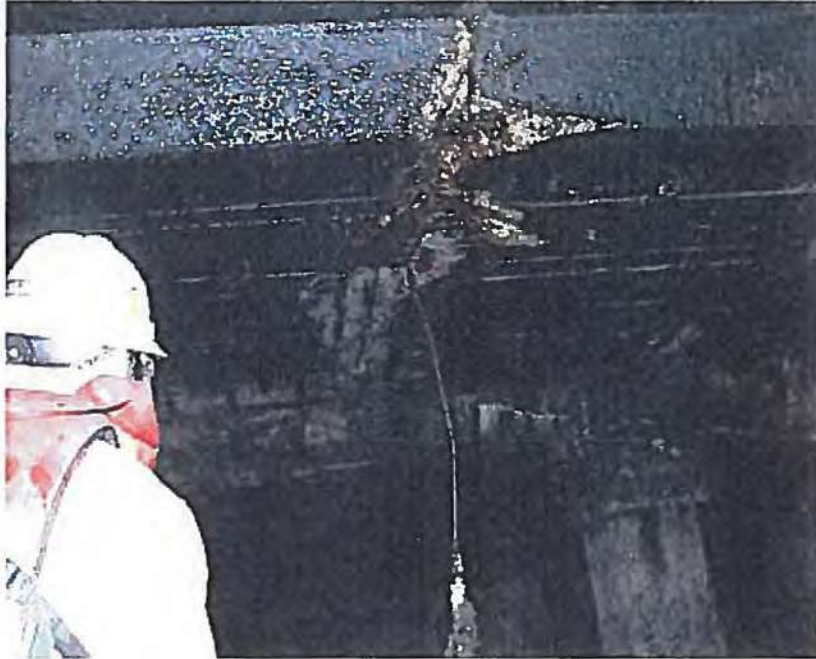
Photo 6--Cracked concrete beams and slab--substructure between sheds A and B and between RR tracks--Severe deterioration
