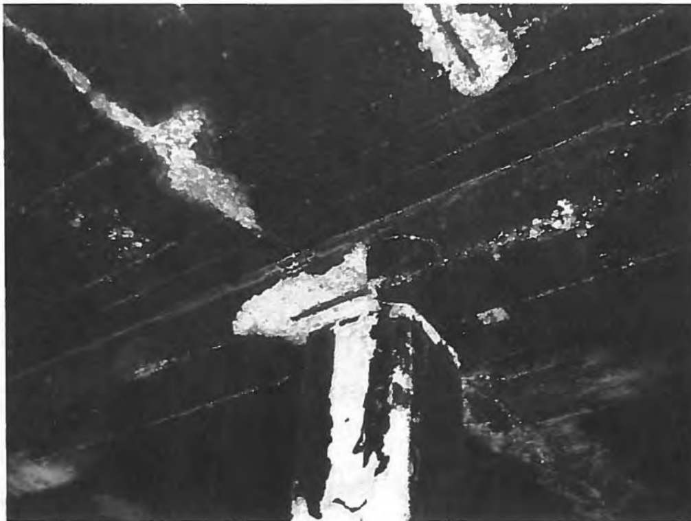
Figure 4: Spalling at deck
