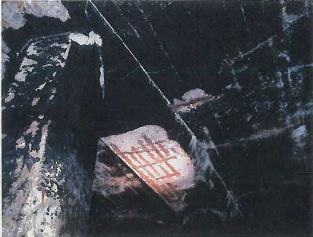
Figure 22: Spalling at deck
