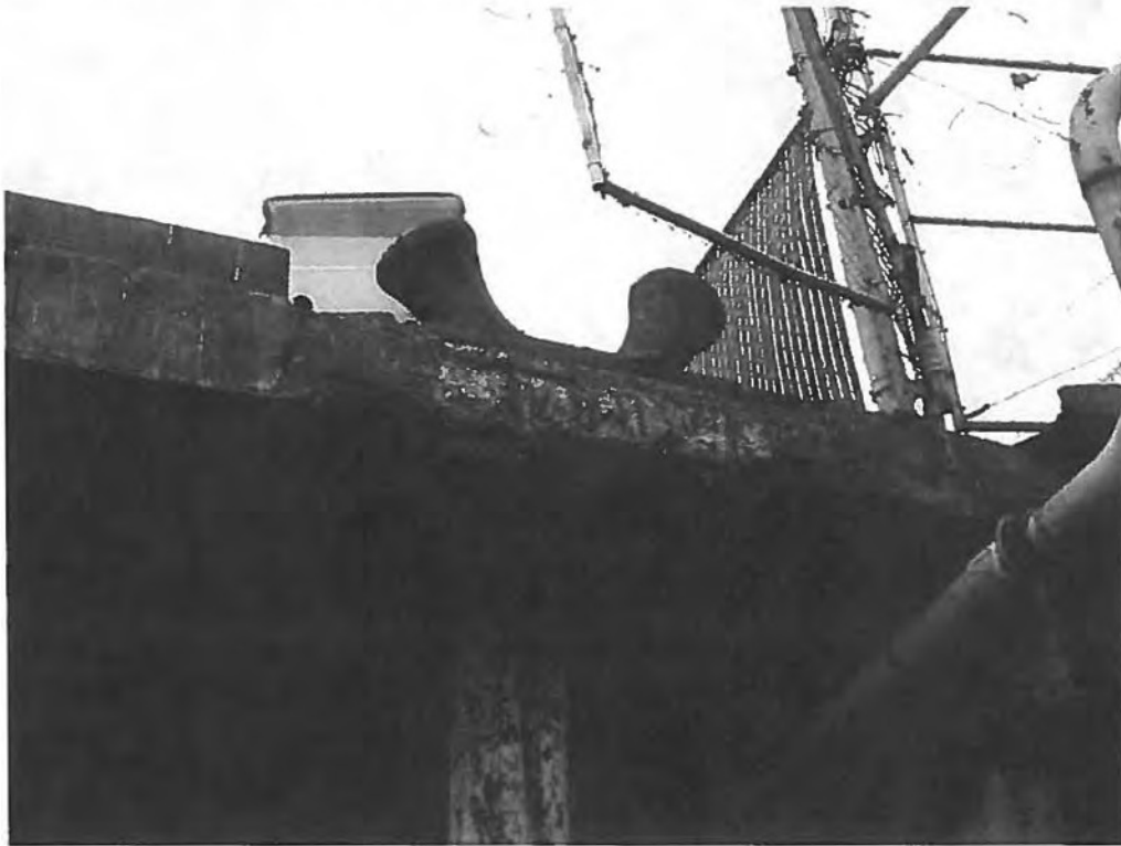
Figure 23: Edge of deck, north end
