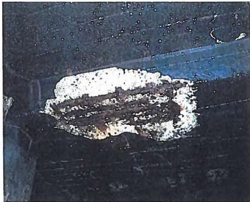
Photo 4--Deterioration in concrete beam under sheds
