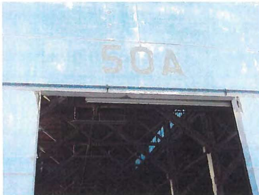
Photo 2. Spalling and exposed rebar at east elevation
