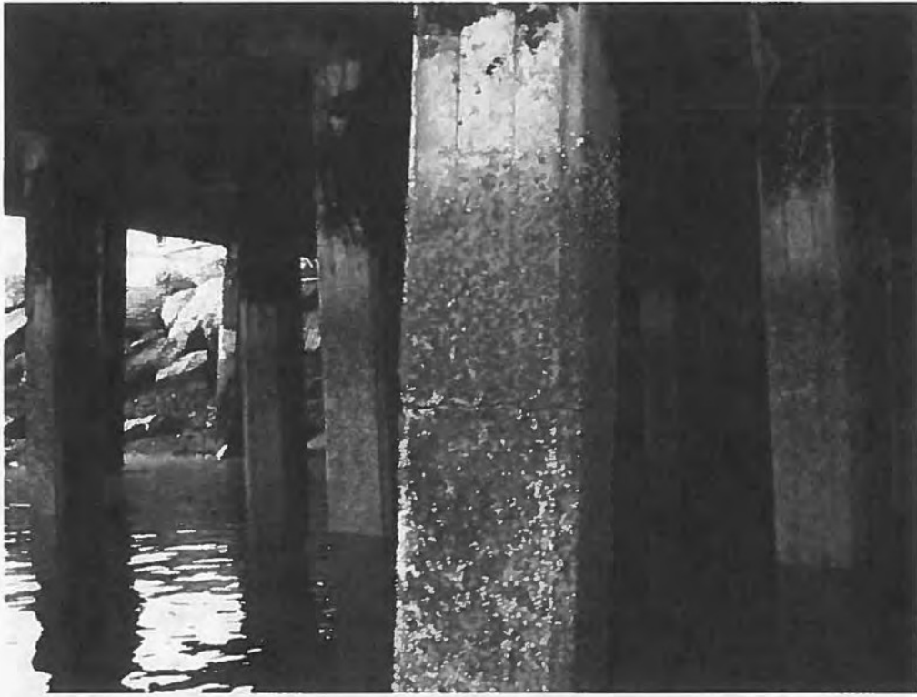
Figure 17: Crack in pile, pile out-of-plumb
