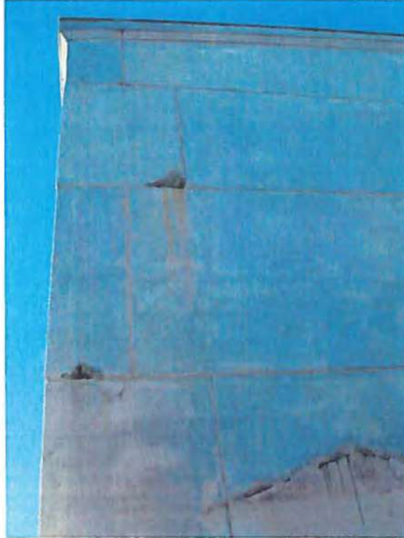
Photo 1. Concrete spalling at southeast end
