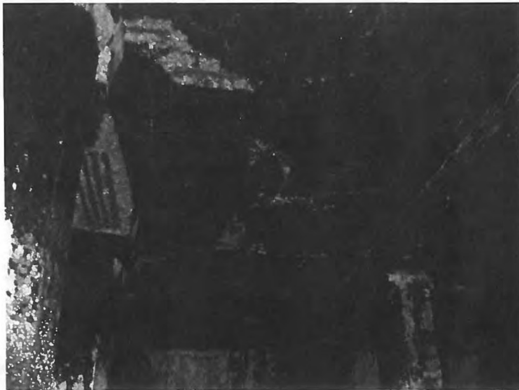
Figure 16: Spalling at deck, girder
