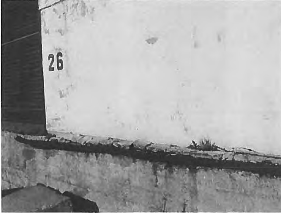
Photo 3. Concrete spalling and corroded metal edge at south elevation
