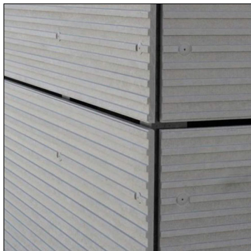
CEMENTITIOUS PANEL OR STUCCO WITH REVEALS - EAST AND WEST PROPERTY LINE WALLS
