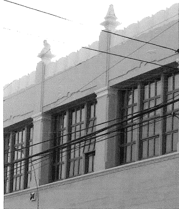
Figure 19. Typical condition at second floor level of east classroom wing facing Bryant Street.
