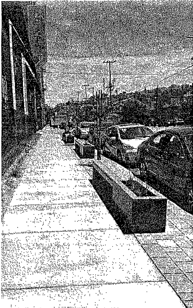
Local San Francisco manufacturer, Heath Ceramics, was awarded an Urban Watershed Stewardship Grant from the SFPUC to install permeable paving in the sidewalk along their storefront. Photo: Heath Ceramic
