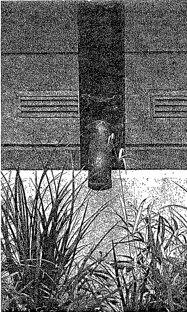
A disconnected roof downspout spills into a bioretention planter. Photo: Krystal Zamora
