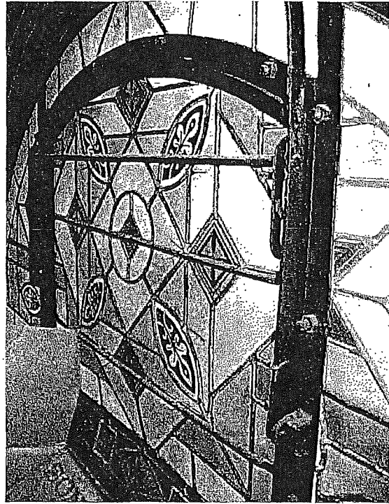
Figure 42 e. Upper portion of window showing corroded hopper-type opening assembly.
