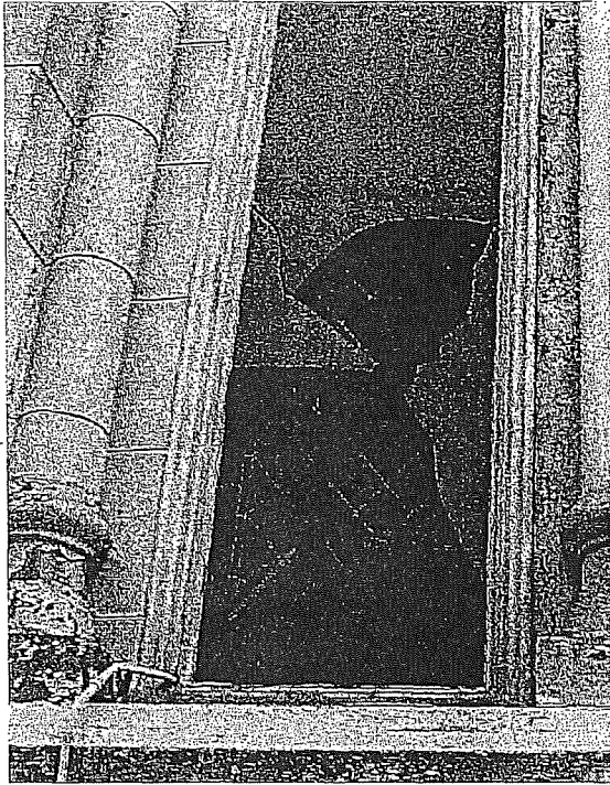
Figure 38a. West tower, north window, showing broken protective glazing.
