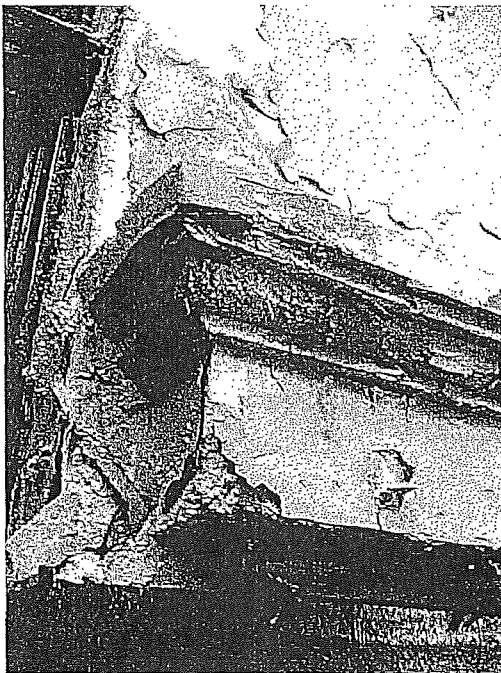
Figure 40c. Softening and deterioration of decorative plaster elements caused by moisture from faulty roofing.
