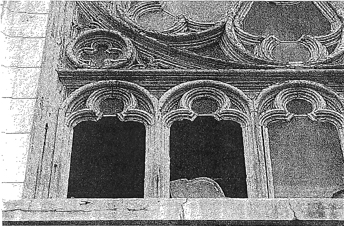
Figure 38c. West transept rose window, showing paint loss and missing glazing.
