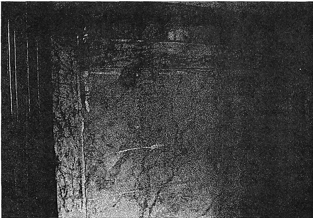
Figure 39b. Detail, showing tape and adhesive residue.
