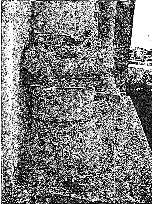
Figure 37a. Column base, south side of east tower, showing flaking and loss of protective paint layer.
