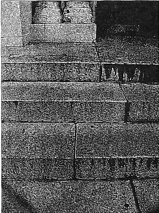
Figure 33a. Main portal steps, showing soiling, paint stains and vertical joints without mortar.
