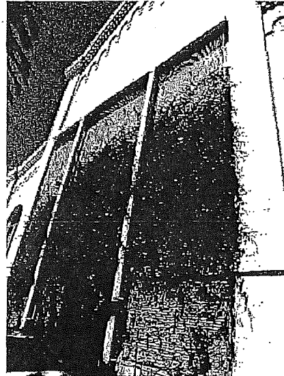
Figure 16. Structural metal frame with mesh screen and climbing vines on rear (south) façade. Source: Page & Turnbull, April 2019.
