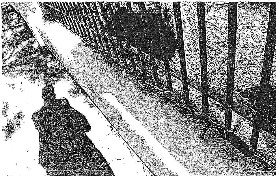
Figure 32c. Low brick wall along Howard Street, showing gaps and voids, corroded metal fence, and graffiti (painted over with mismatched paint).
