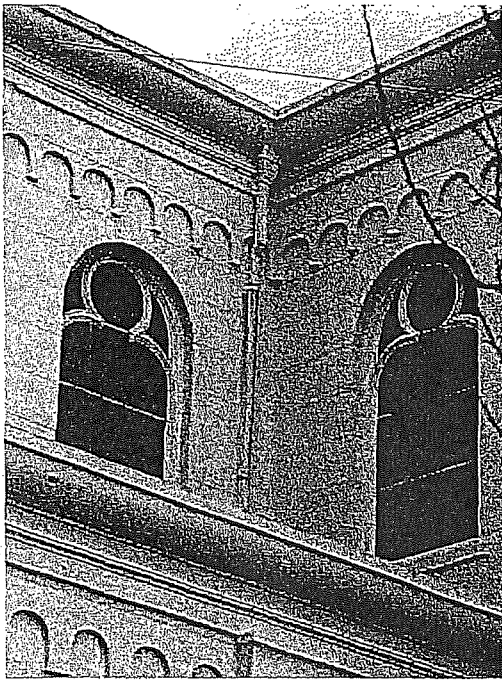
Figure 40a. West façade, showing blocked or perforated drainage which is causing damage to interior plaster.
