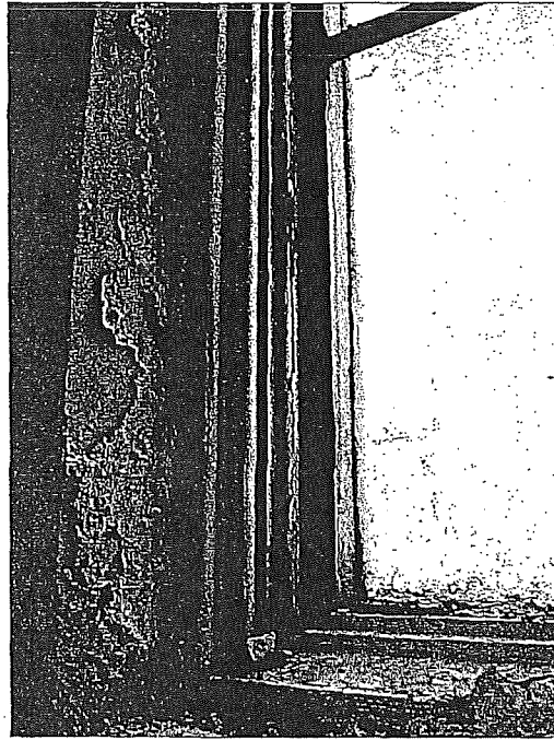
Figure 40b. Deterioration of plaster caused by moisture from poorly sealed window.
