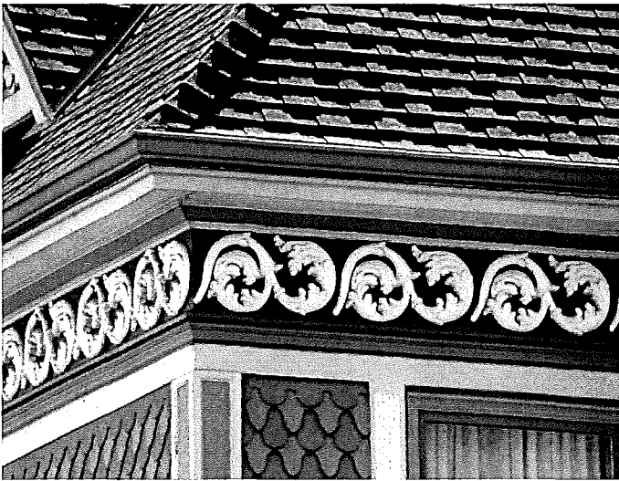
Figure 7. Detail of northwest corner of house at second floor: Note the fishscale shingles and fascia featuring vine motif and articulated eaves. (Photograph by Garavaglia Architecture, Inc., April 2015.)
