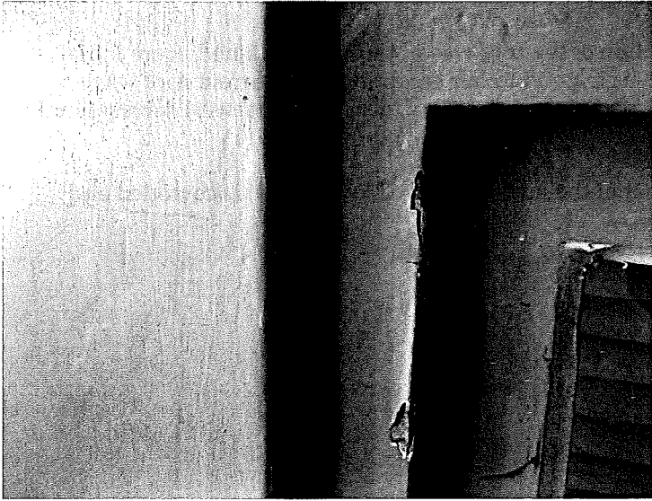
Figure 19. Peeling paint at basement level. (Photograph by Garavaglia Architecture, Inc., April 2015.)
