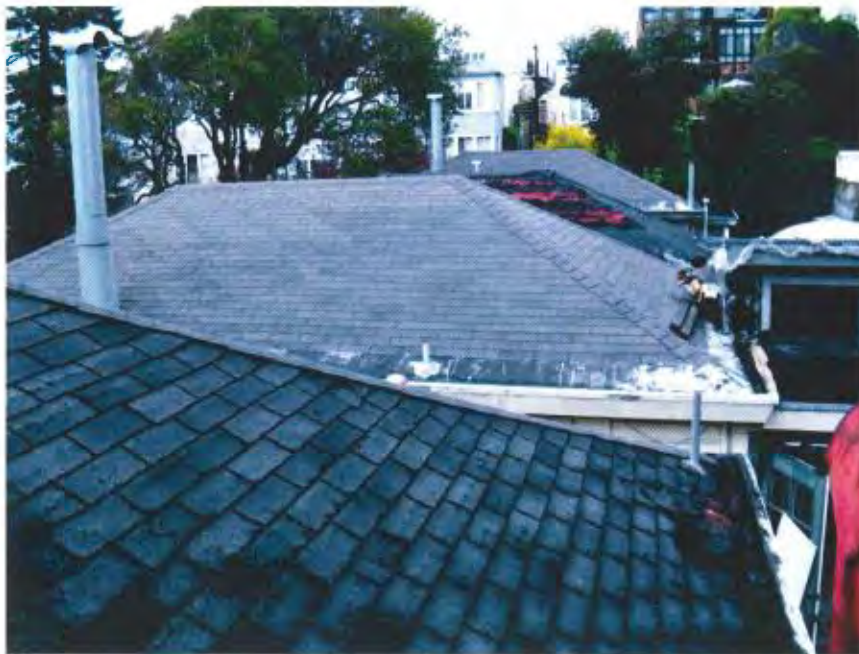
Figure 5. Detail of cottage roofs. Note the round metal flues on the cottages.
