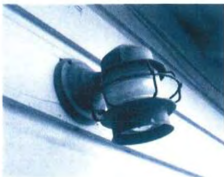
Figure 28: Wall mounted industrial entry porch light.
