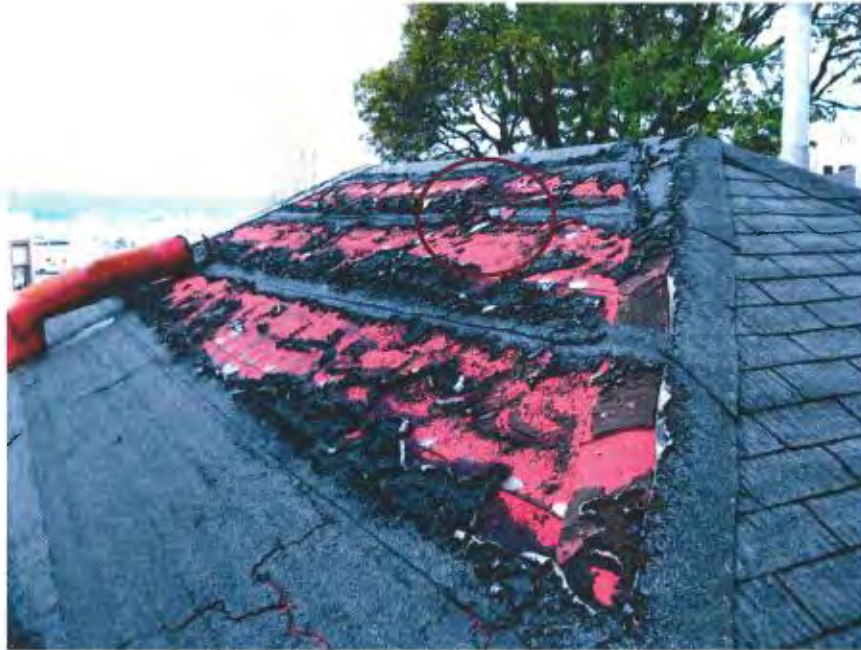
Figure 8. Location of Sample 3 at the ridge of Cottage C. Sample area is circled in red.
