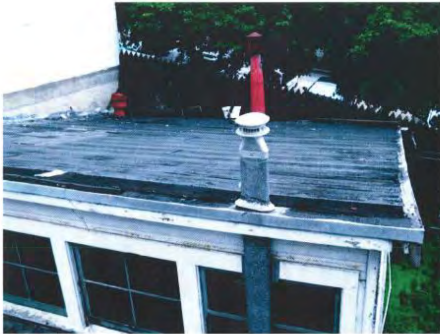
Figure 6. Detail of Studio roof. Note the round metal flue in the background.
