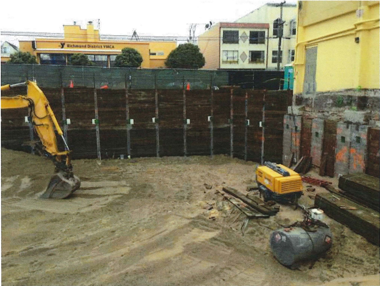
Figure 8 1810 8th Ave - 30,000 CY of sand. All compaction done with water and excavator. No vibratory rollers. Note hand dug pits.
