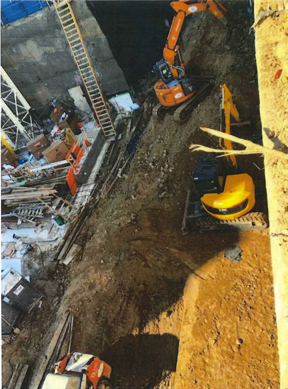
Figure 5. 390 1st Street Excavation of sandstone with no hoe-rams. All equipment shown is <63hp (Demolition, Excavation and shoring 28,000 CY)
