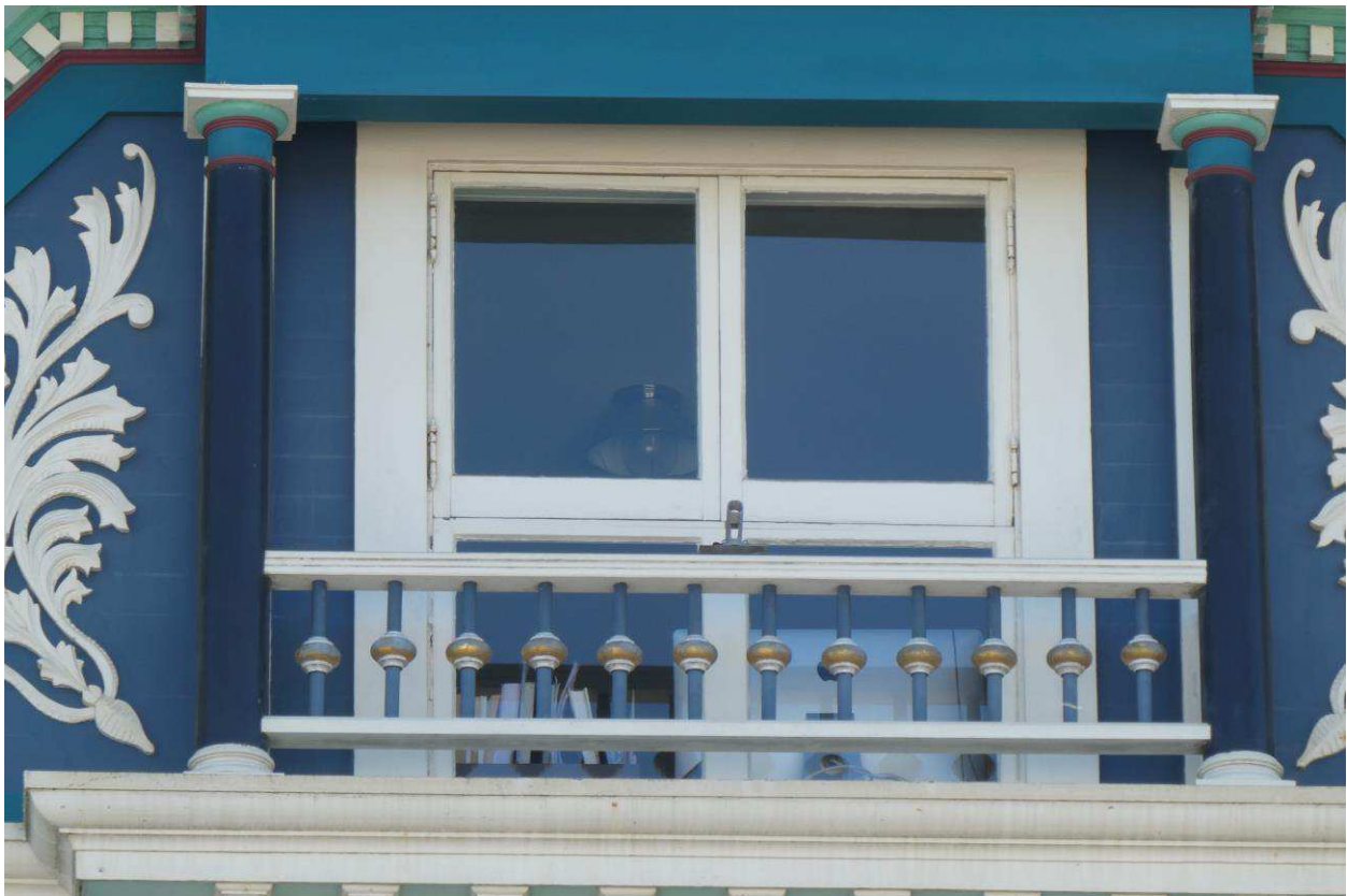
Figure 38: Exterior detail of the attic window at the Waller Street gable end.
