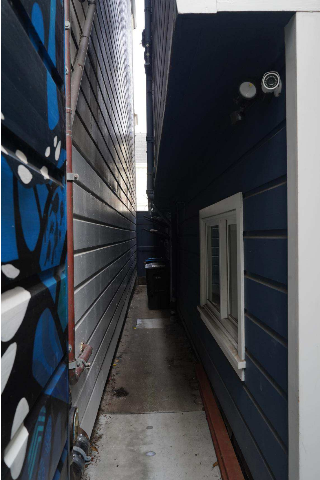
Figure 46: Overall view of the walkway at the southwest side of the building. Note the mechanical and plumbing flues/piping at the upper portion of the wall in the distance. See also (Figure 48).
