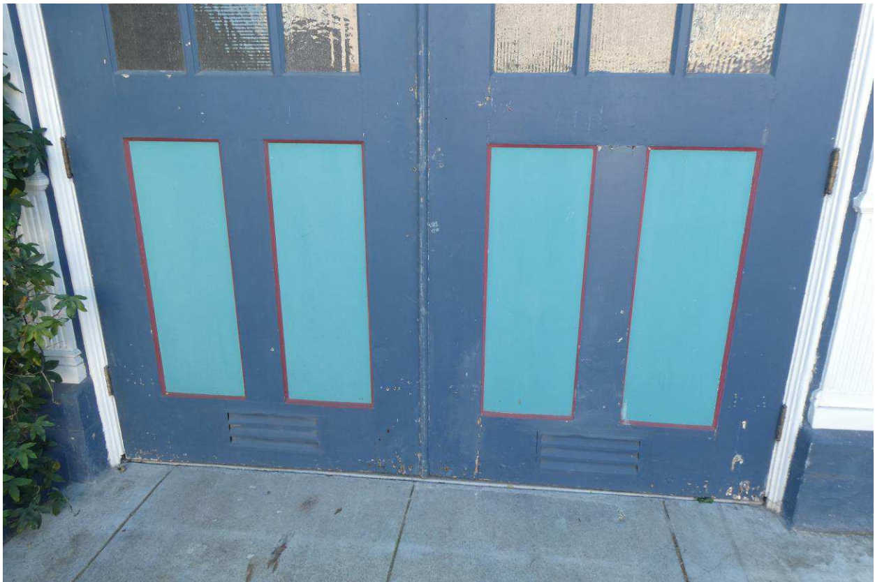
Figure 30: Detail showing deteriorated wood at the bottoms of both garage doors.
