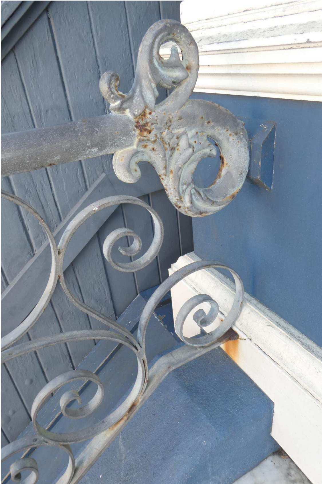
Figure 33: Detail of typical corrosion at the wrought and cast iron stair rail.
