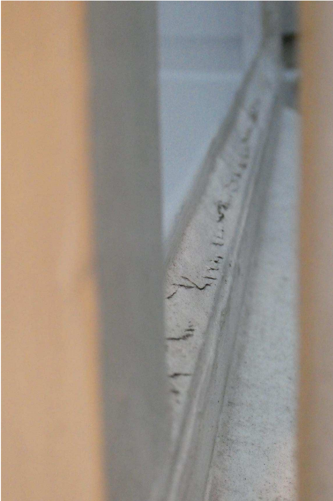
Figure 50: Detail showing deteriorated glazing sealant at the Plexiglas, second floor non-historic casement sash, northeast lightwell.
