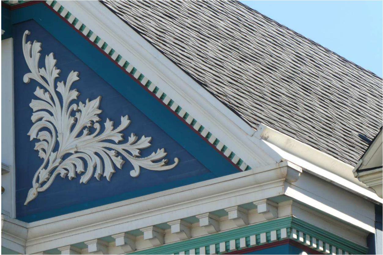
Figure 52: Detail showing the main roof's gutter/diverter at the southwest gable side from Waller Street
