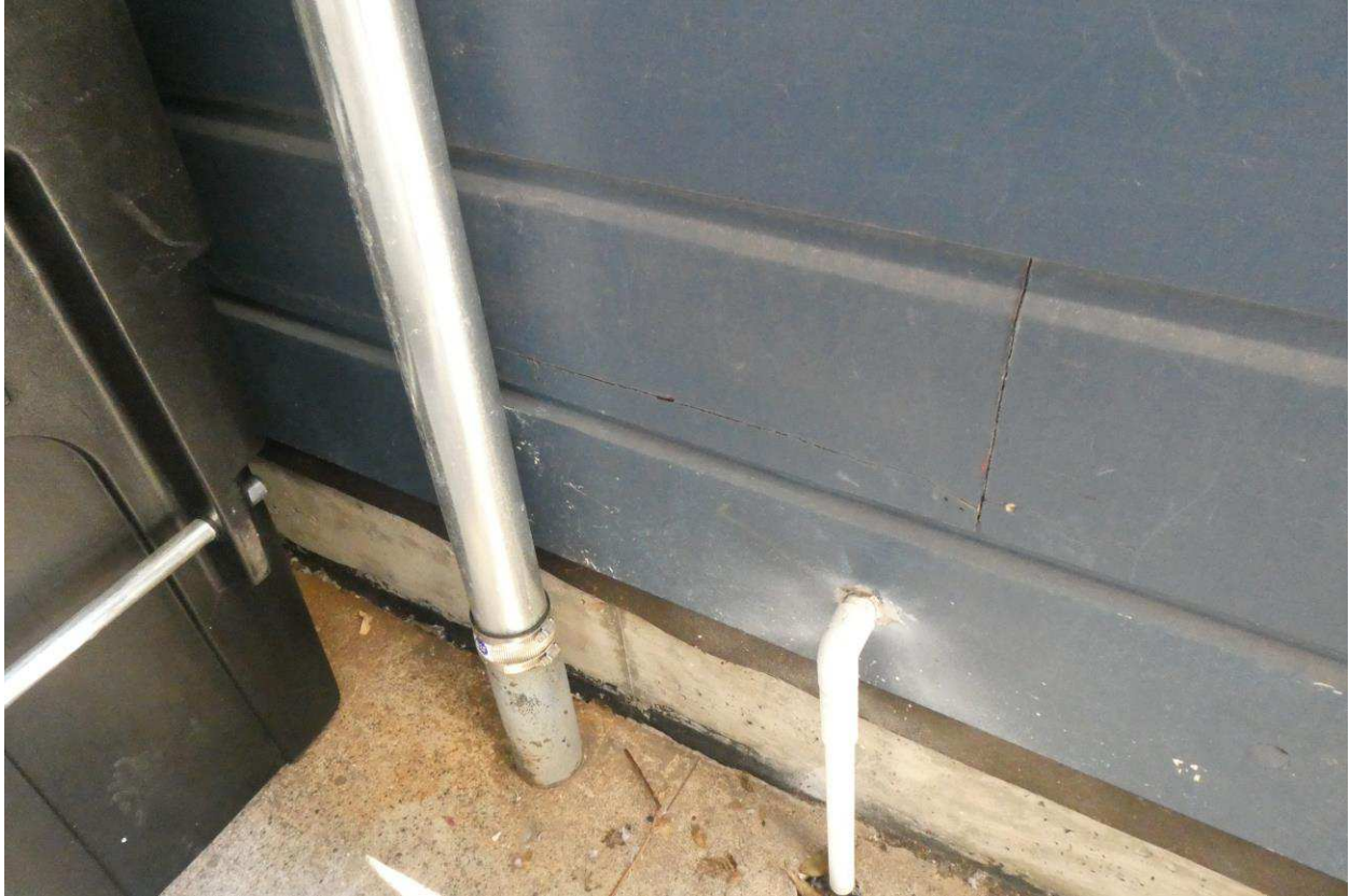
Figure 47: Detail of checked/splitting at siding on the southwest elevation.
