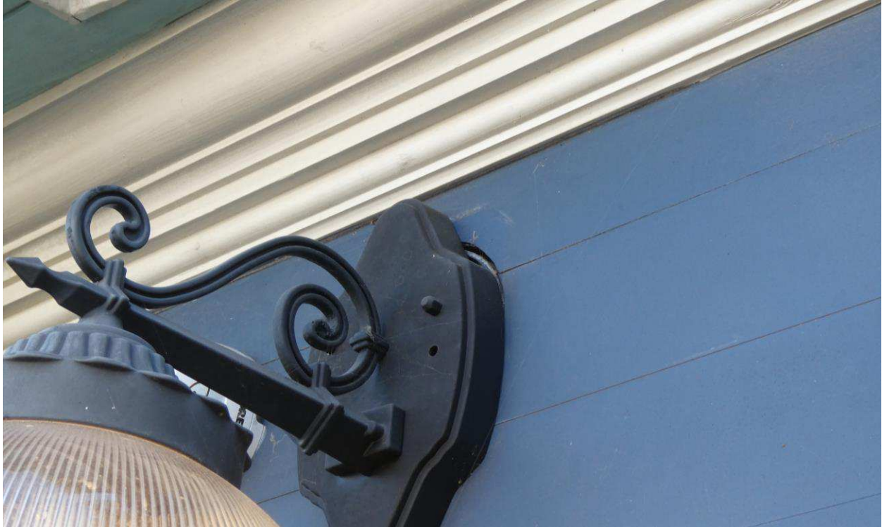
Figure 27: Detail showing gap between garage sconce escutcheon and wood siding.
