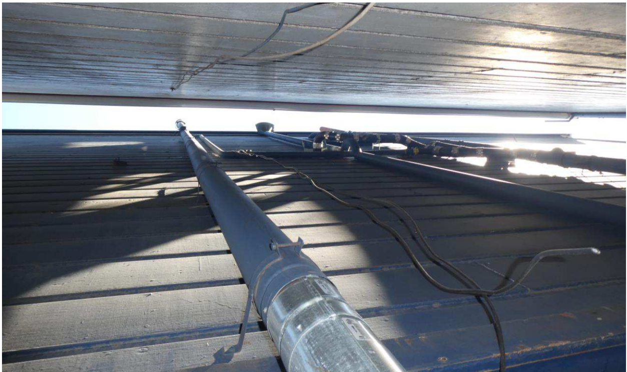
Figure 48: Detail showing the mechanical and plumbing flues/piping/conduits at the upper southwest wall.
