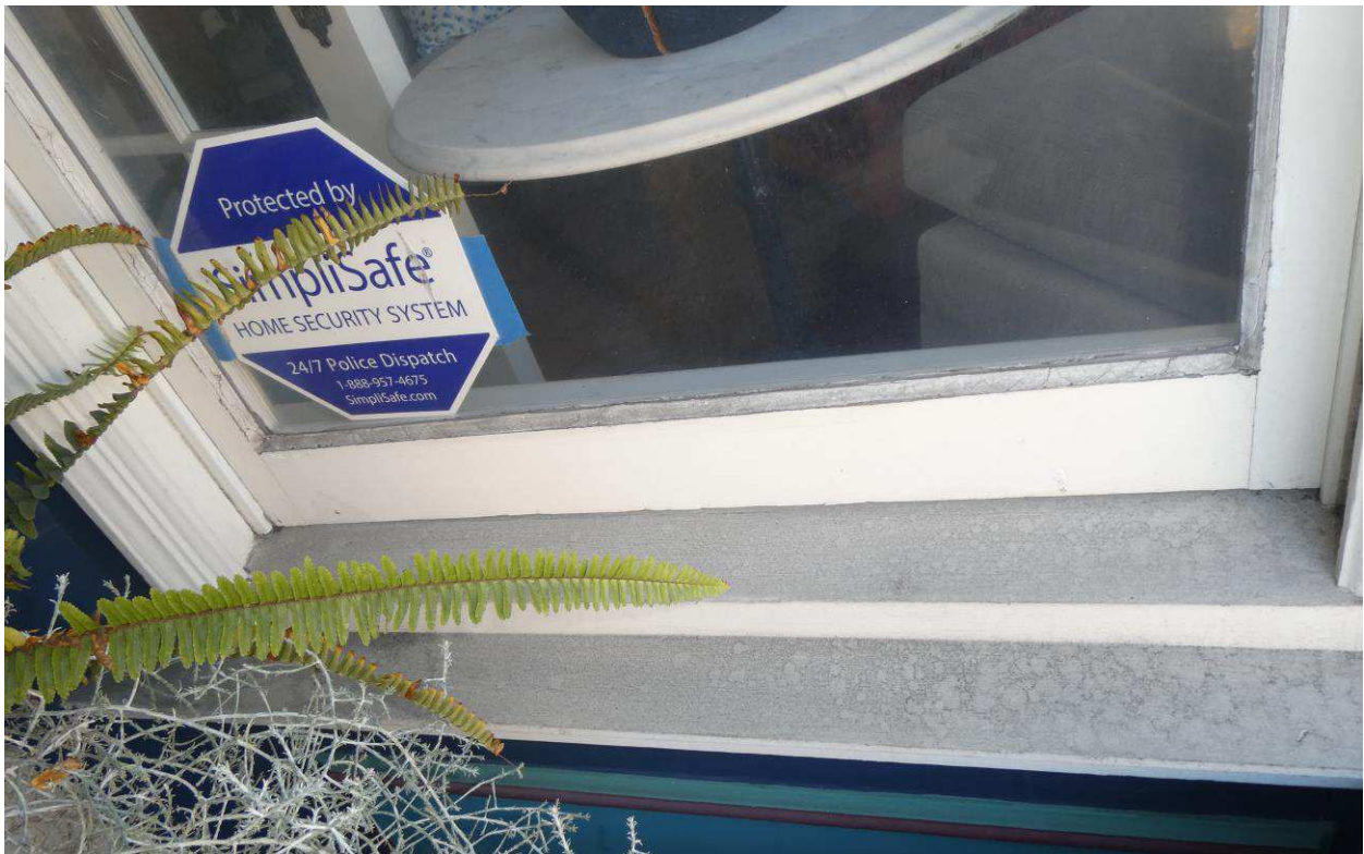
Figure 35: Detail showing cracked and deteriorated glazing putty at the first story windows.
