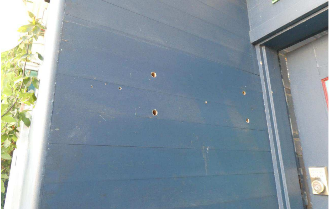
Figure 29: Detail showing holes at the ground level siding.
