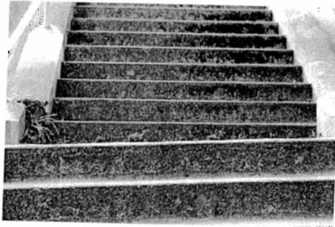
Section near top is displaced and tilted, due to a tree root. The city removed the tree about 10 years ago.
