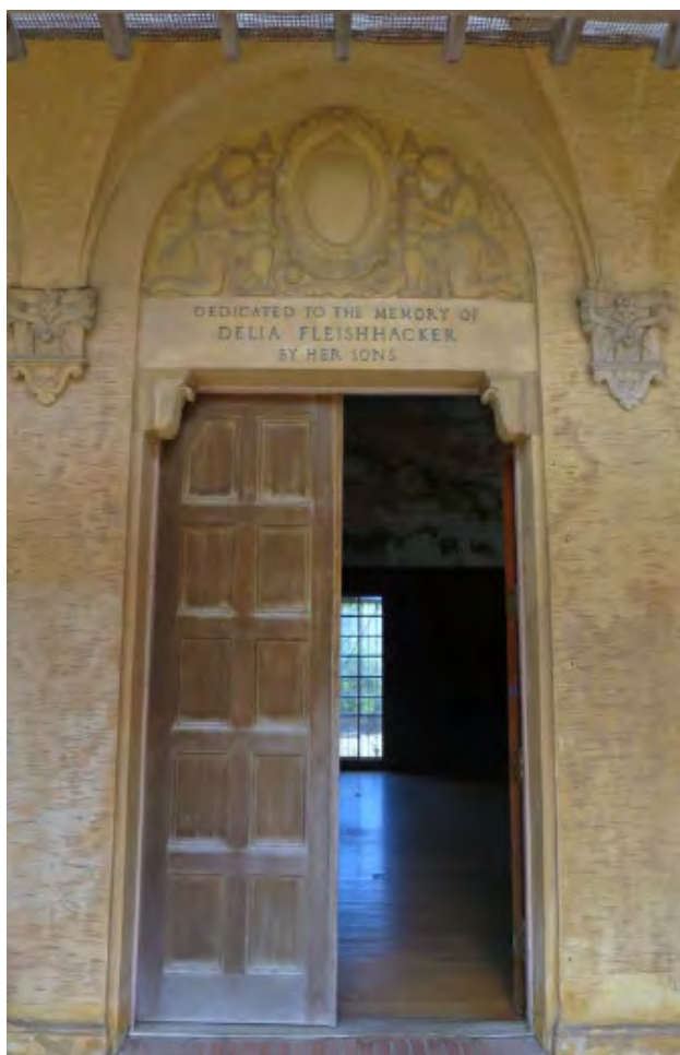
Mother's Building, main entrance, view west, 2016. Source: Architectural Resources Group, Inc., Mother's Building Conditions Assessment
