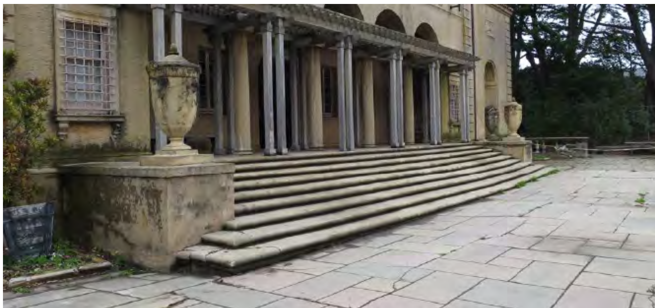
Mother's Building, terrace/plaza and entrance stairs at east elevation, view northwest, 2016. Source: Architectural Resources Group, Inc., Mother's Building Conditions Assessment
