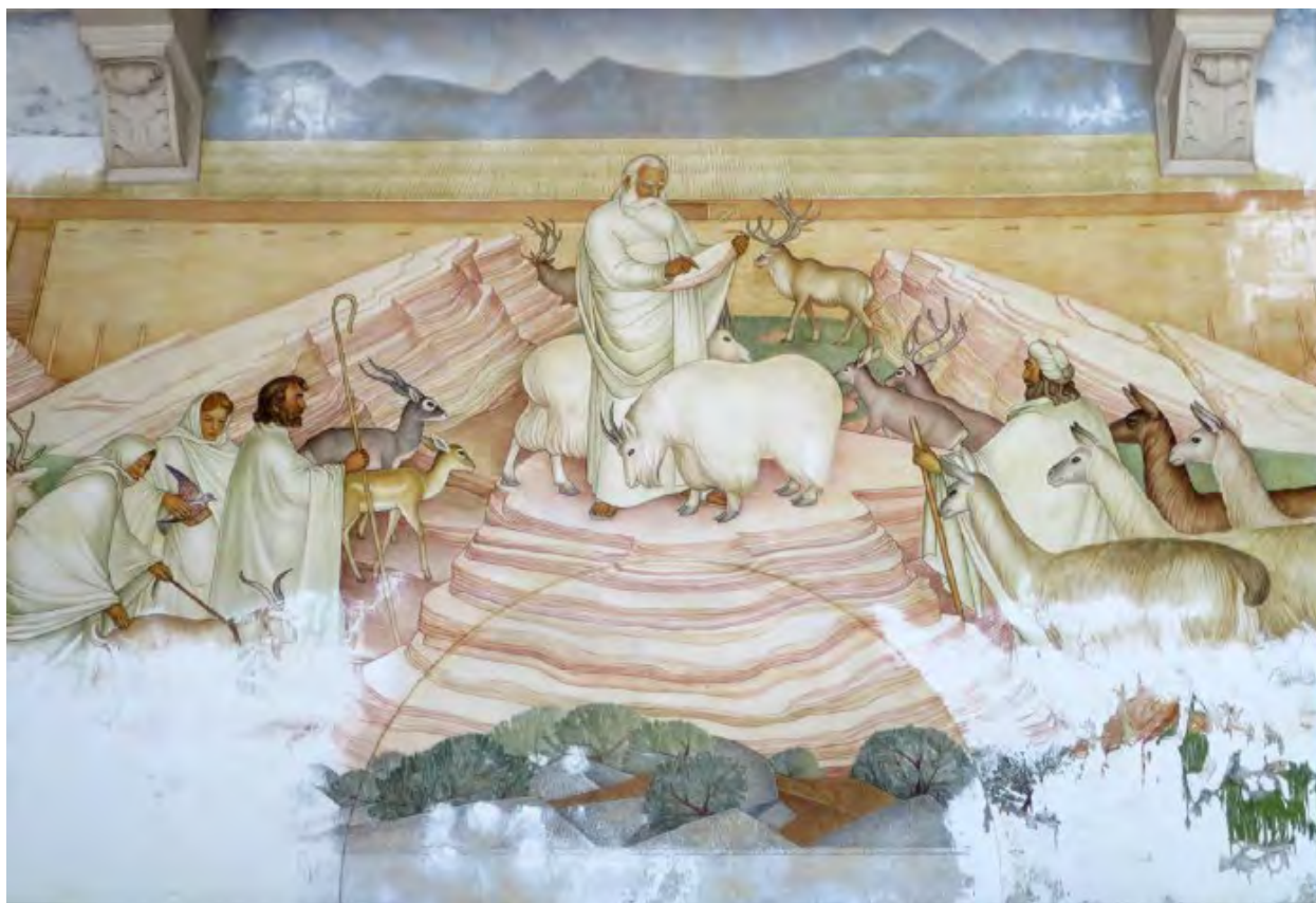
Mother's Building, west wall of main lounge, detail of Loading of the Animals , 2016. Source: Architectural Resources Group, Inc., Mother's Building Conditions Assessment
