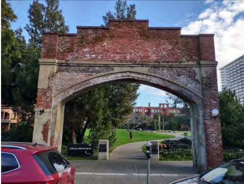
The ivy has been removed leaving faint traces of paint. Source: Richard Brandi, 2022
