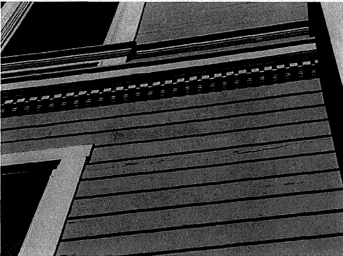
Figure 24. Peeling paint at the south facade (Garavaglia Architecture, Inc., October 2016)
