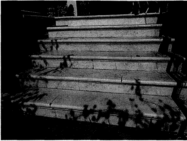
Figure 13. Marble stairs leading to the front entrance of 940 Grove Street (Garavaglia Architecture, Inc., October 2016)
