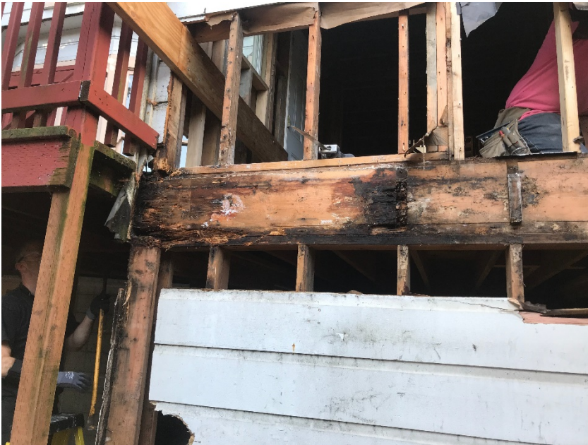
Detail photos of dry rot located at rear of building
