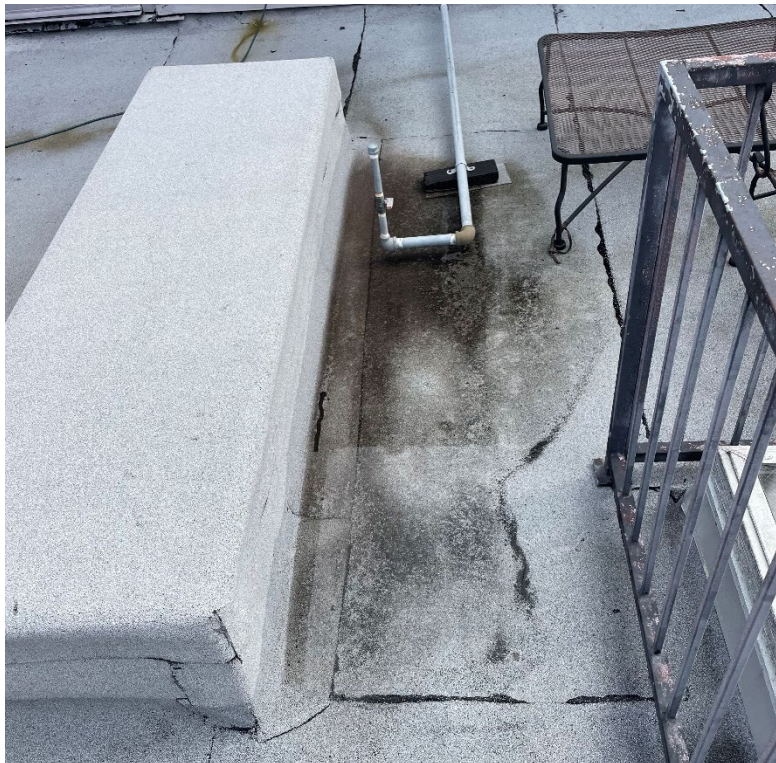
Figure 47: Active ponding on the main roof.
