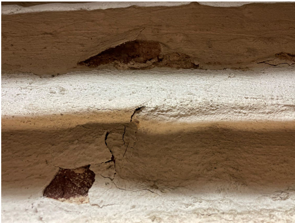
Figure 55: Paint loss at efflorescence, north wall, basement.
