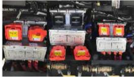
Figure 2 Service/ maintenance switch
