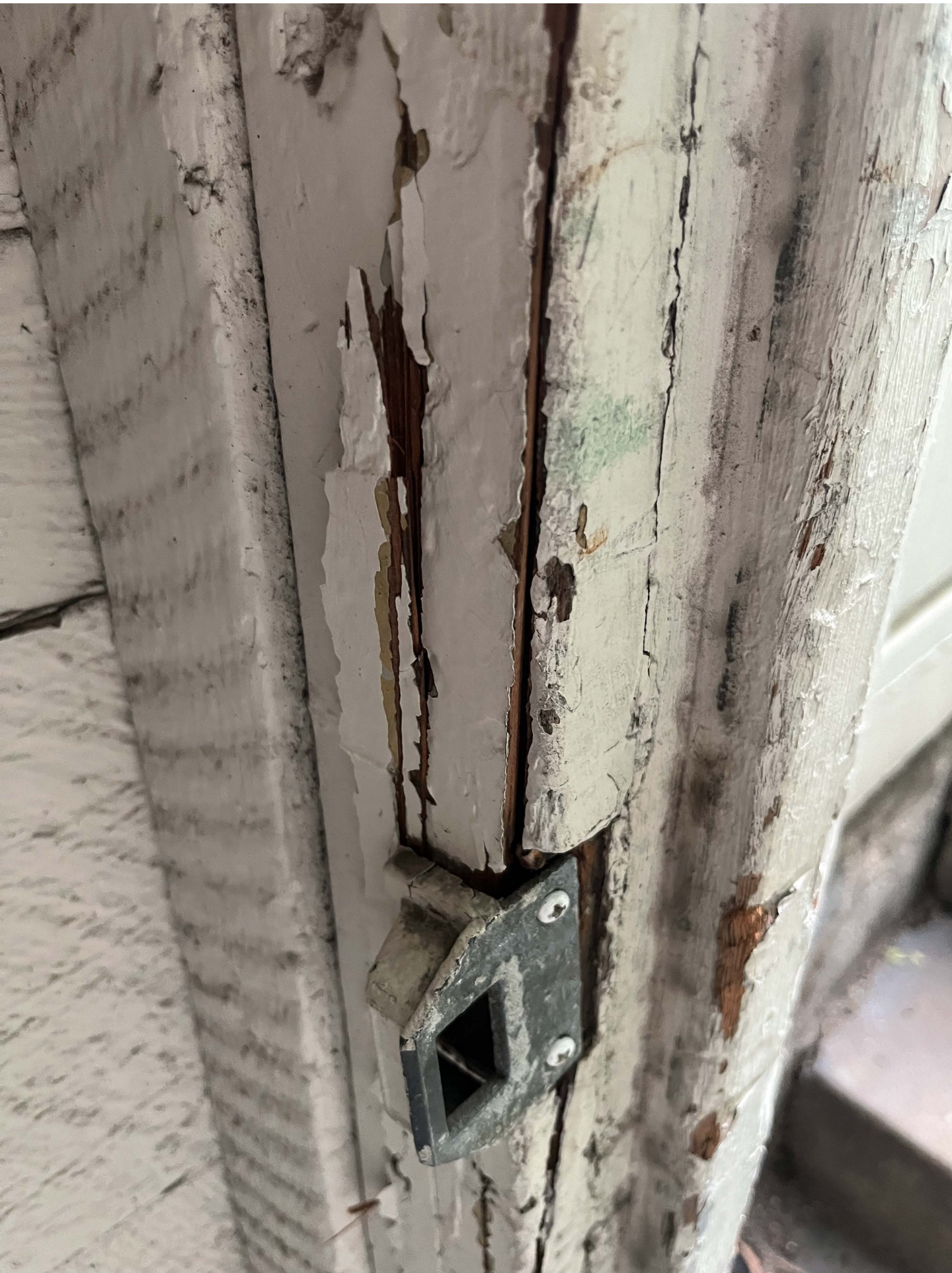
Photo: The door to the back yard on the south side of the house is in need of repair or replacement. The hardware is falling apart and is a security risk.
