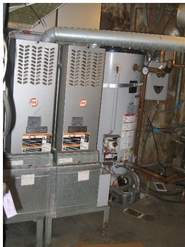
Figure 89: 2d Floor Mechanical Room
