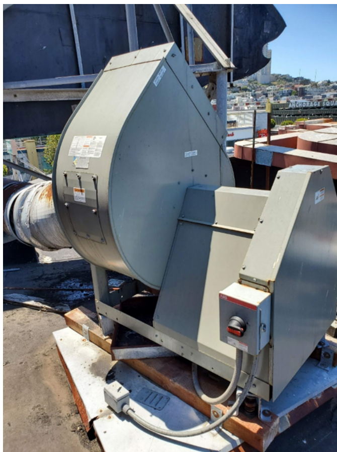
Figure 5 Newer kitchen exhaust fan
