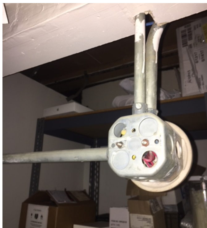
Figure 19 Missing knock outs
