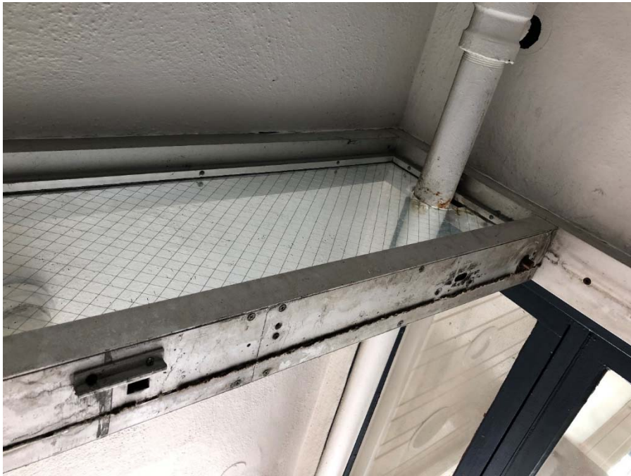
Figure 23 Breezeway double door missing one door frame damager
