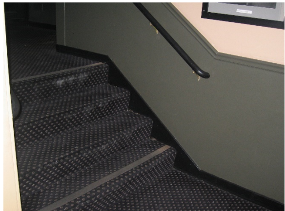
Figure 45: Stair #1 to 2 nd Floor, missing Handrail Ext.
