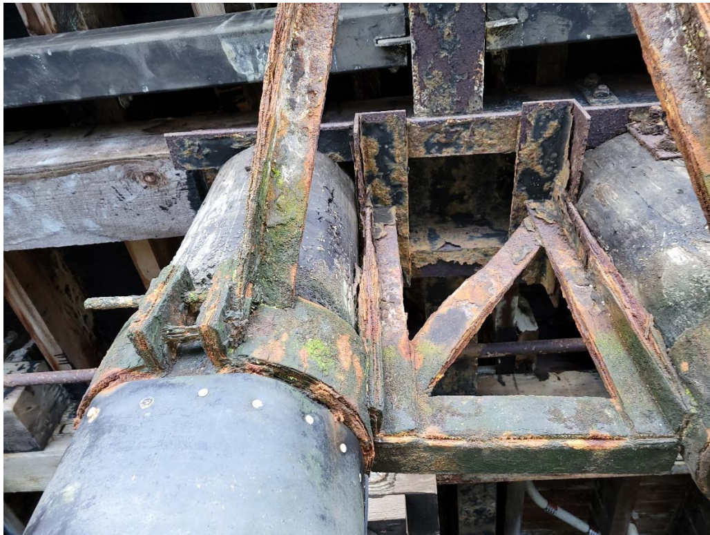
Figure 3 Structural steel framing elements show signs of corrosion
