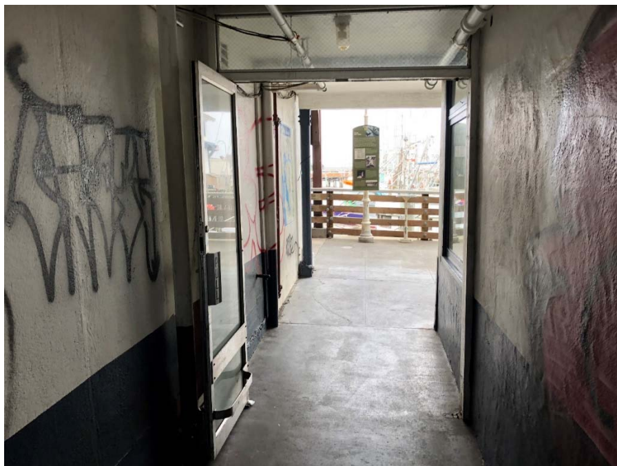
Figure 25 Breezeway double doors missing one door
