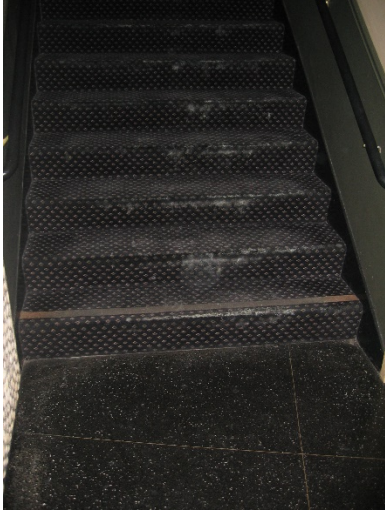
Figure 18: Staircase #1, missing Handrail Extensions
