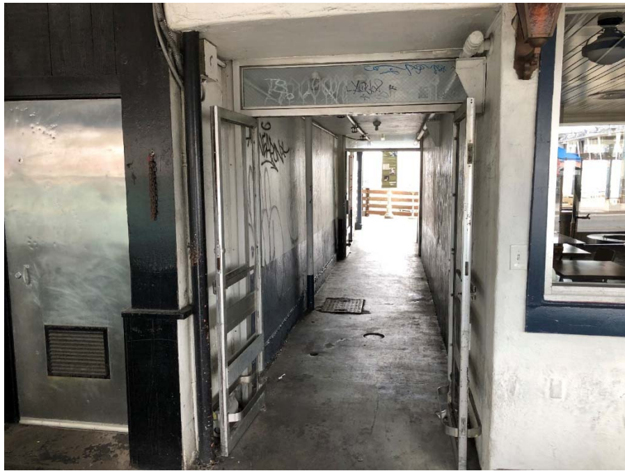
Figure 26 Double doors missing glass
