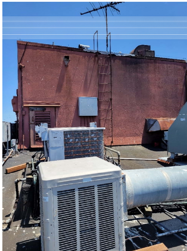
Figure 7 - Ladder – Top connection of ladder appears loose – Roof
