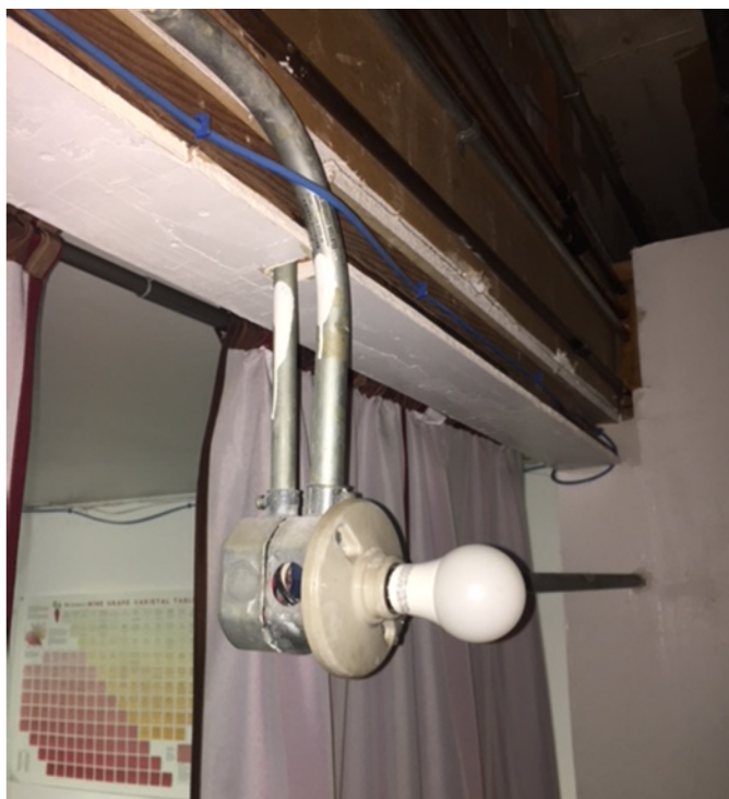
Figure 20 Missing knock outs
