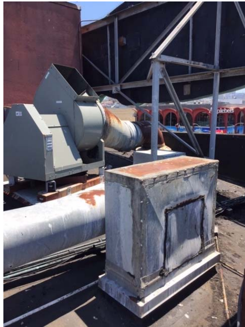
Figure 12 Roof Duct surface rust
