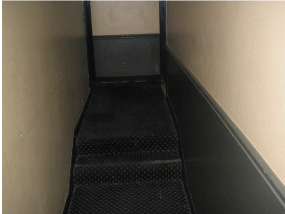
Figure 44: 2 nd Flr. Steps to Men's RR, missing handrails
