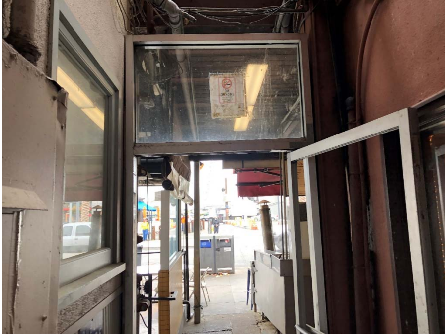
Figure 22 Single door in breezeway broken glass
