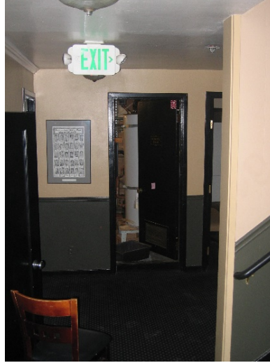
Figure 53: 2 nd Flr. Landing, missing handrail Extensions
