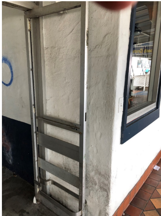
Figure 27 Double doors missing glass (Right)
