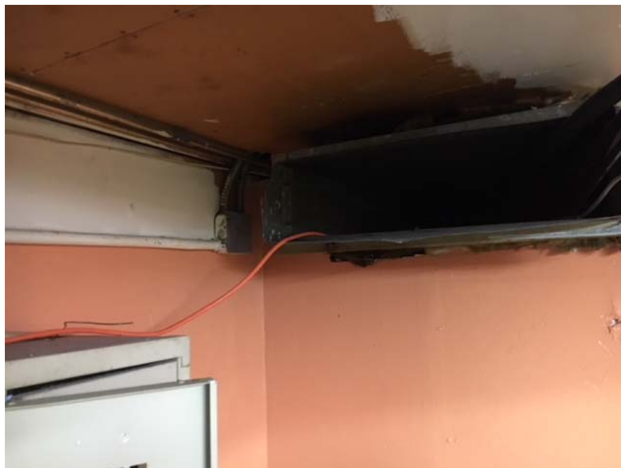
Figure 15 Extension cord inside HVAC duct
