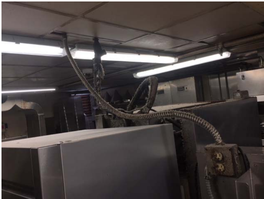
Figure 17 Unsupported flexible conduit
