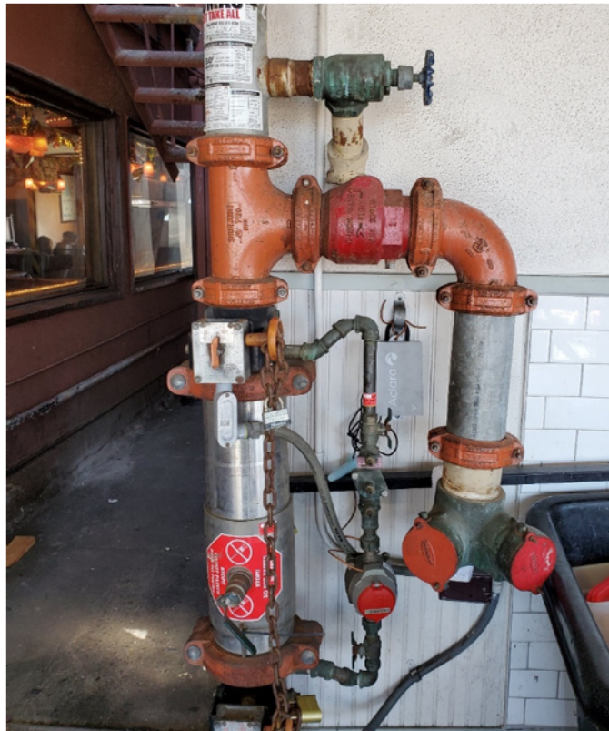
Figure 4 Fire sprinkler riser
