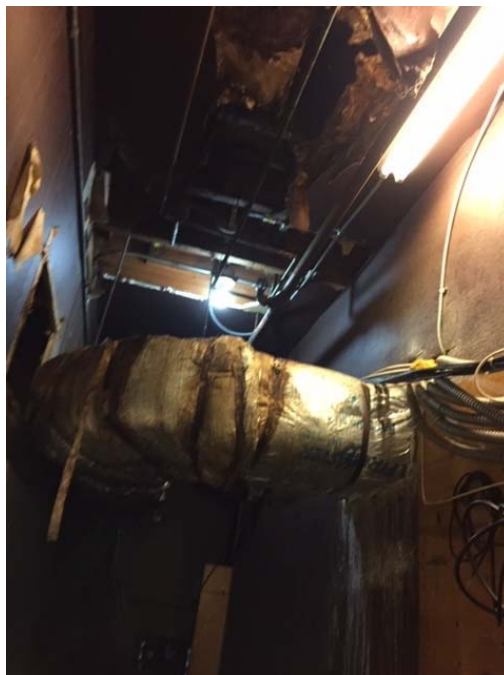
Figure 10 Employee access storage water intrusion
