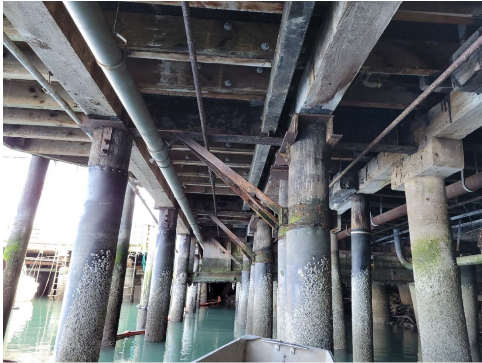
Figure 2 Structural steel framing elements show signs of corrosion
