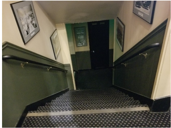
Figure 21: Staircase #1, missing Handrail Extensions
