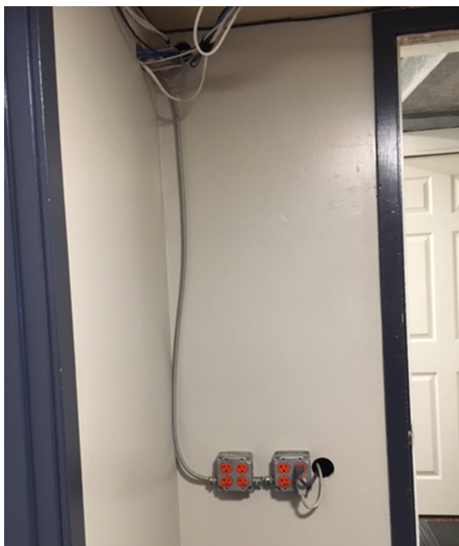
Figure 21 Open wiring, not secured
