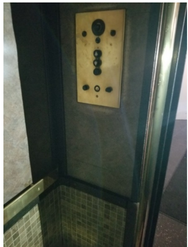
Figure 17: Passenger Elevator/Interior Control Panel
