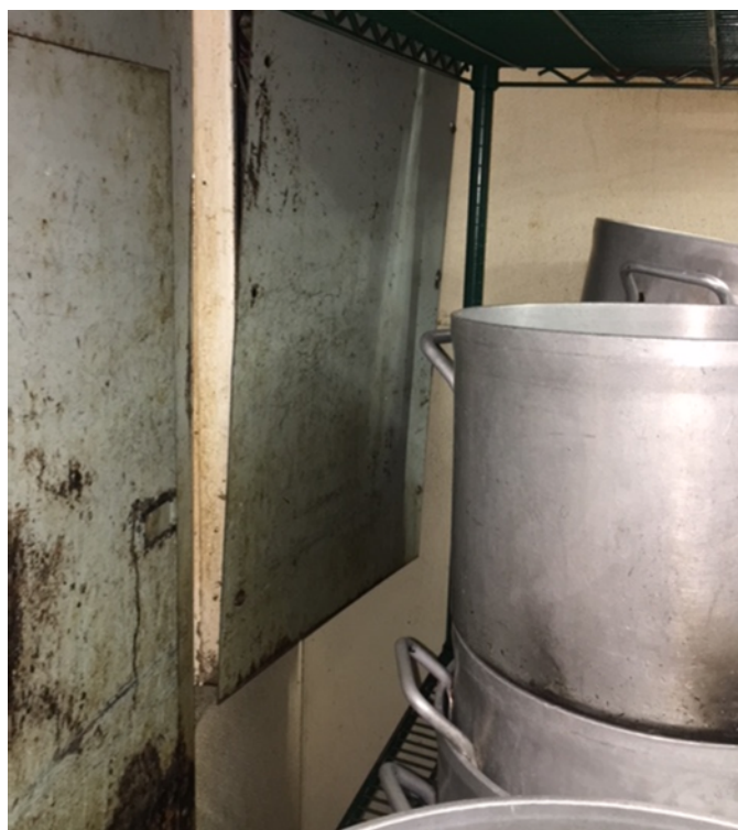
Figure 18 Panel cover not properly secured in main kitchen
