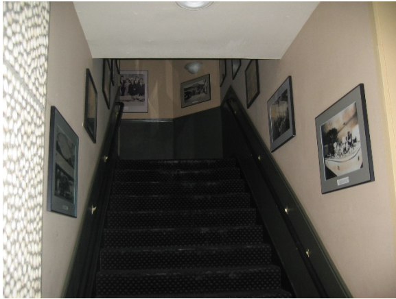
Figure 20: Staircase #1, missing Handrail Extensions
