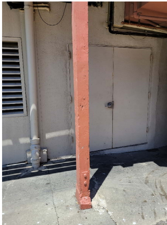
Figure 11 Exterior wood column on south side – minor deterioration at base
