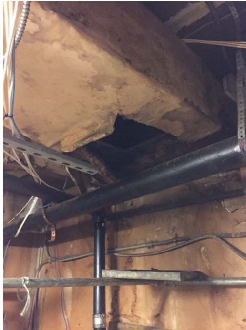
Figure 9 Utility Closet open duct work
