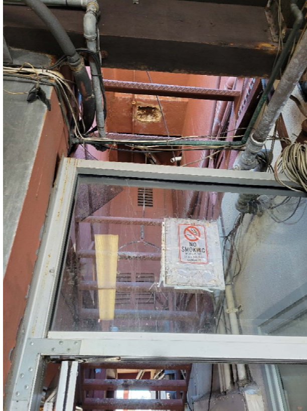
Figure 10 Stucco damage on south side
