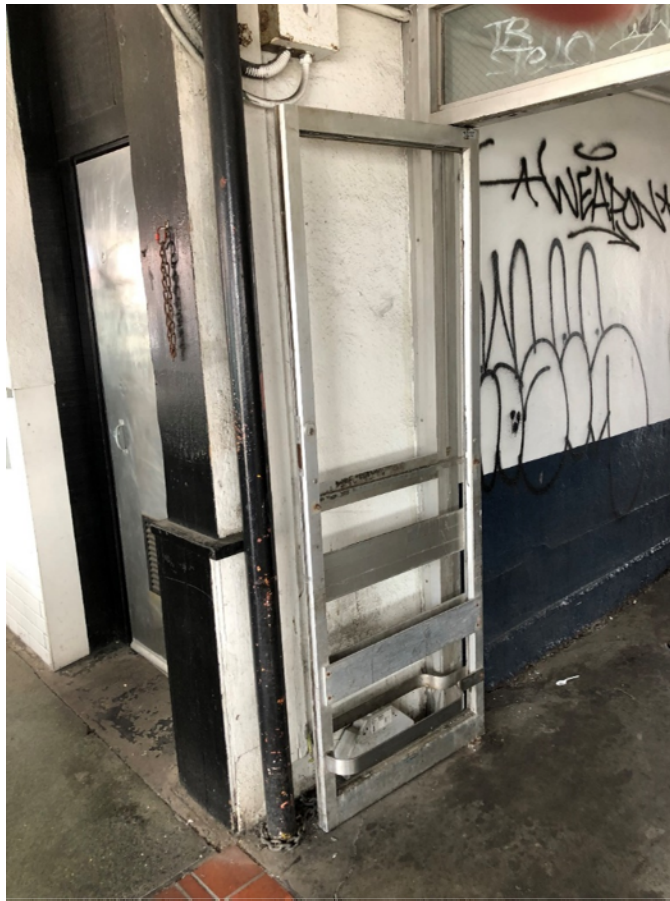
Figure 28 Double doors missing glass (Left)
