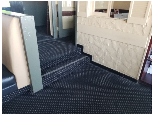
Figure 75: 3 rd Floor Steps to Mid Dining, missing Handrail.
