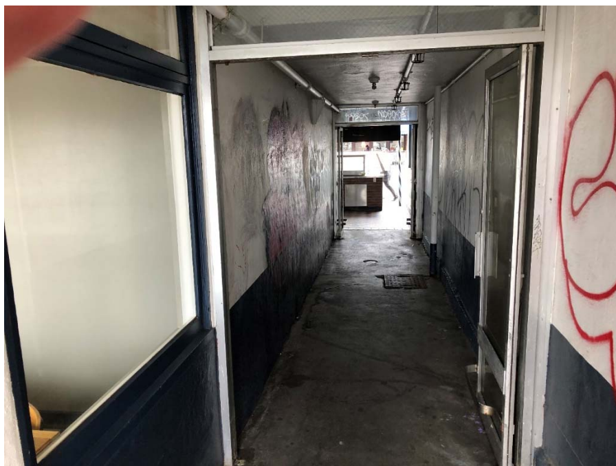
Figure 24 Breezeway double doors missing one door
