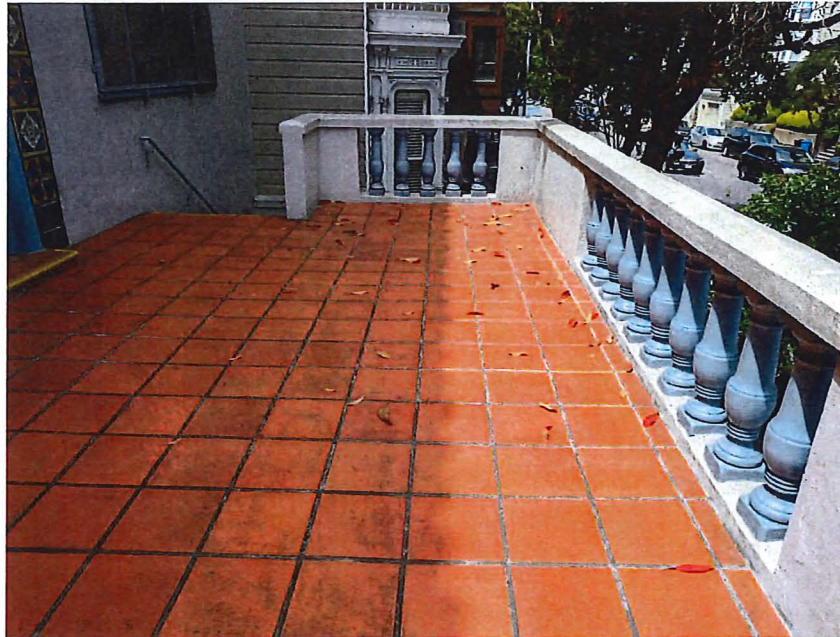
Terra cotta tile at the water table located at the second story of the entry stair, view west.
