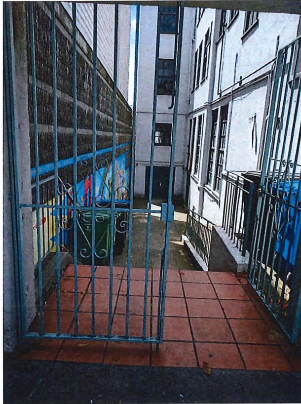
Wrought-iron entry gate leading to side yard at the eastern portion of building, view south.
