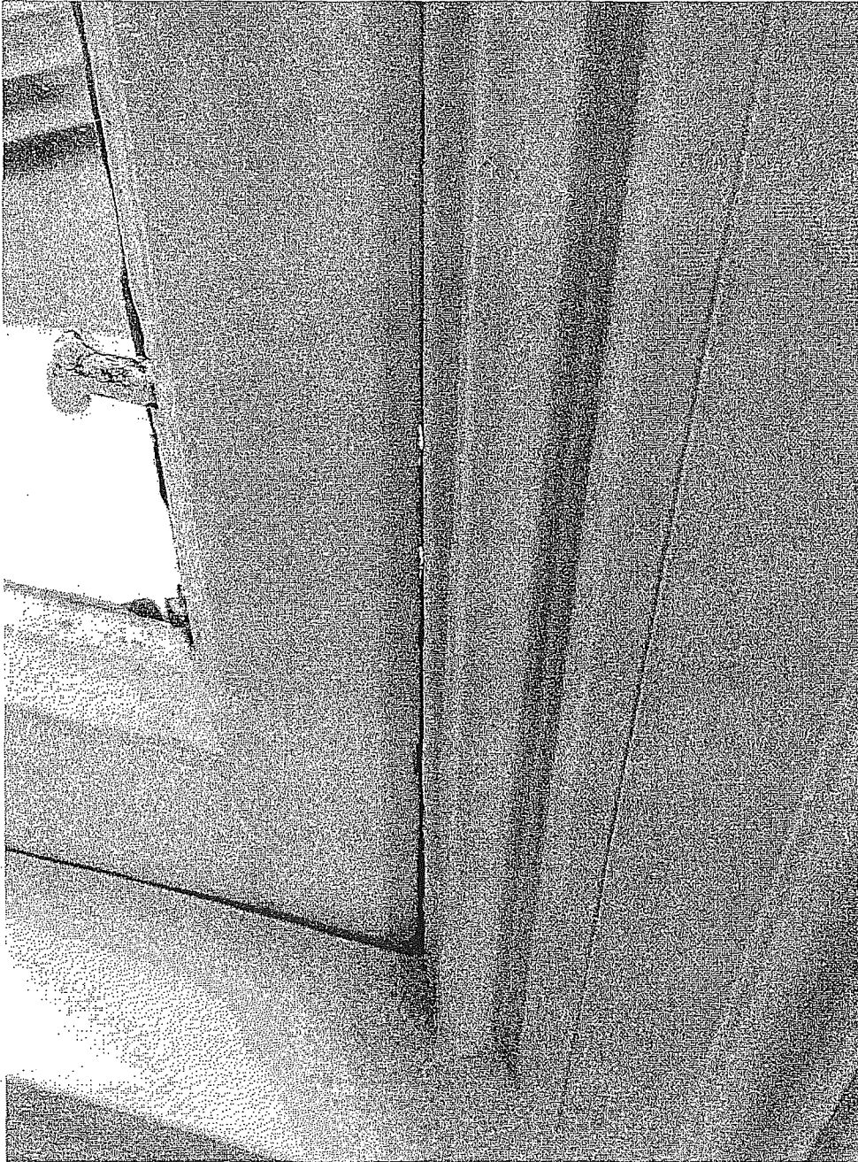
Figure 30: Detail of first floor window from interior showing gap at edge of sash where light is coming through.
