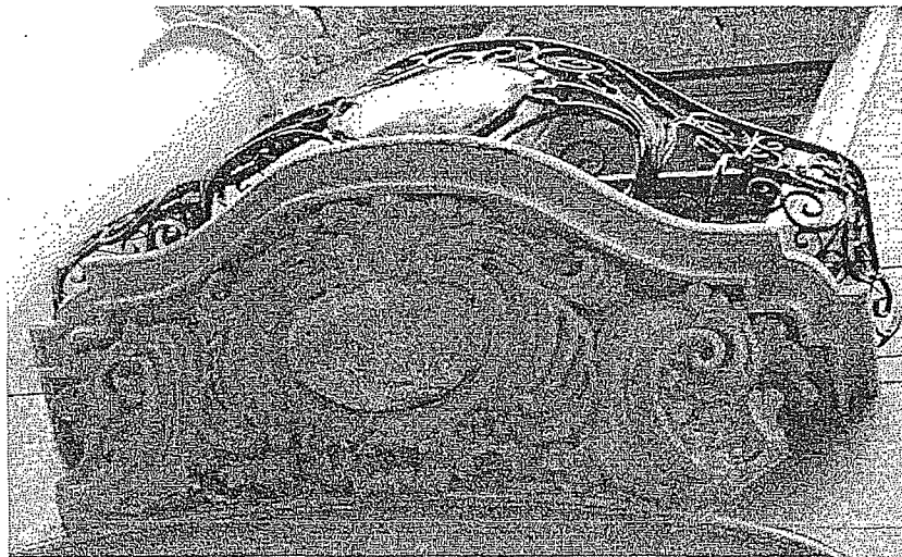
Figure 23: Detail of the molded balcony showing peeling paint at the front edge.
