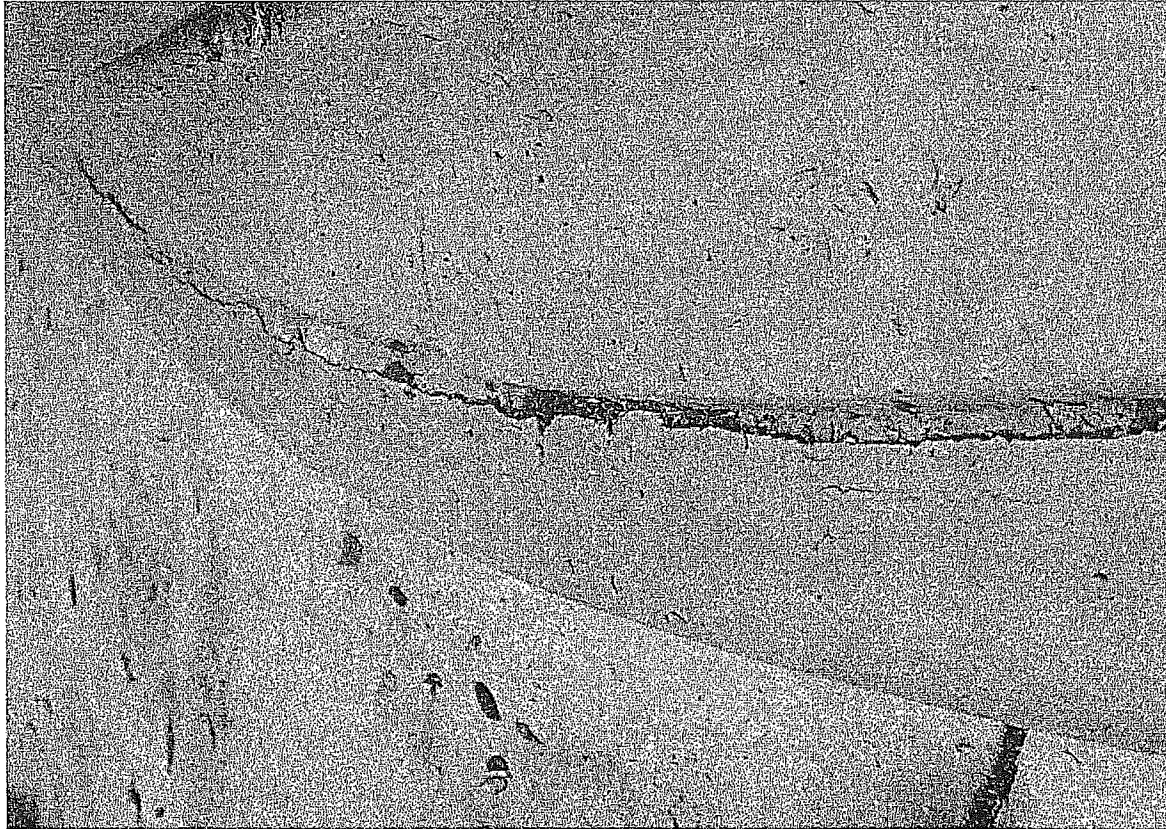
Figure 28: Detail of area where soft deteriorated wood was noted with moisture at the wood.
