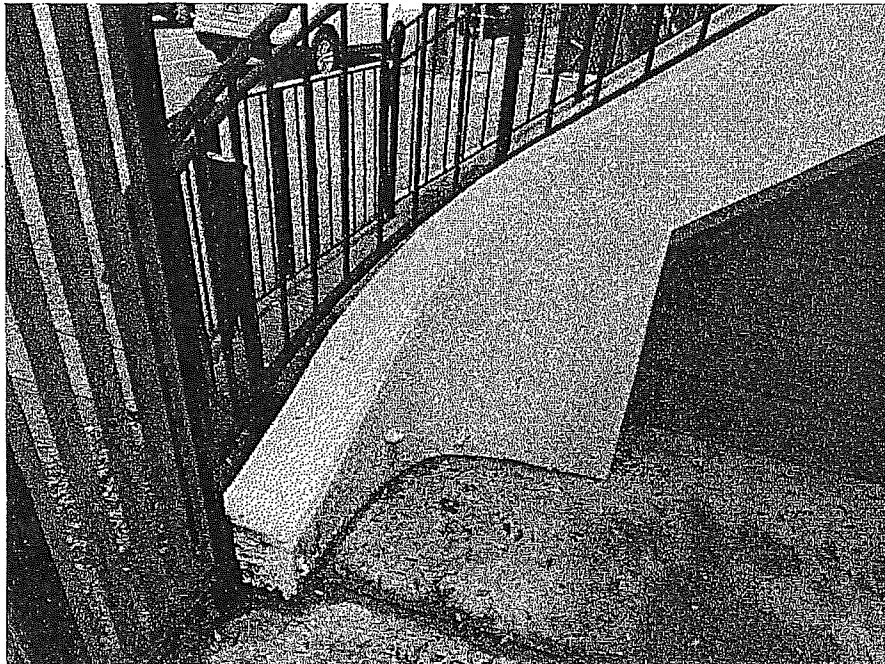
Figure 25: Detail of concrete stair curb with spall.
