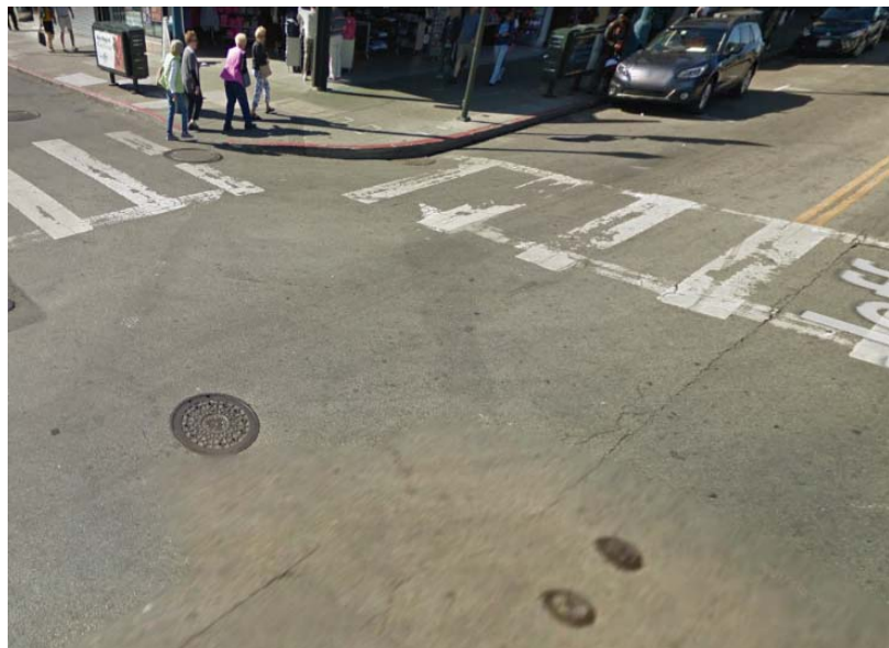
Figure 3: Faded Crosswalks and Missing Curb Ramps at Jefferson and Mason
