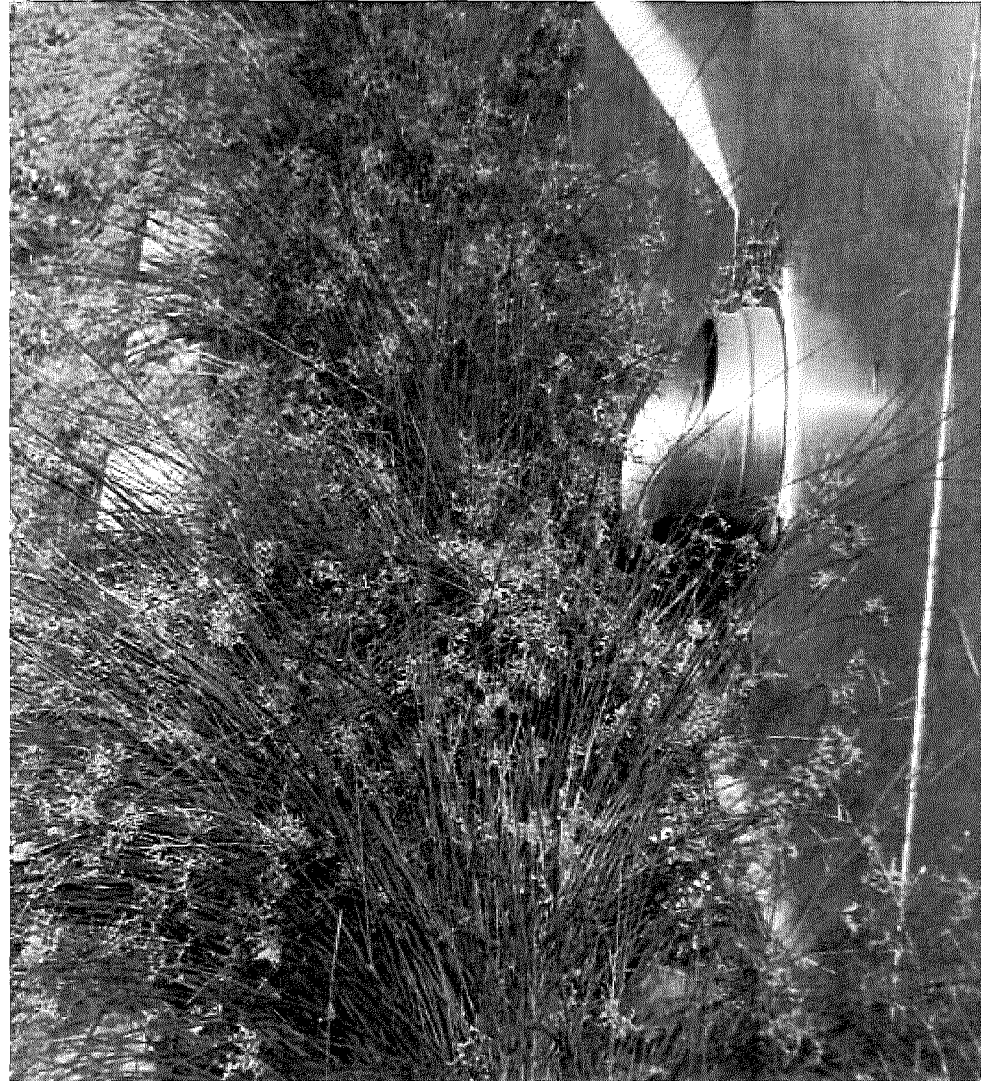
An interior roof drain discharges to a vegetated swale in Emeryville, CA. This properly designed and permitted stormwater facility is an example of an “approved alternate location” for stormwater discharge.
