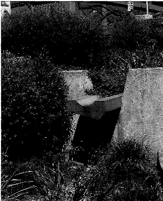
Weirs (top) and cascades (bottom) make street-side bioretention possible on steep slopes in Seattle, WA.
