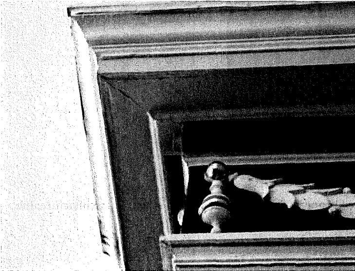
Figure 18. Peeling paint at perimeter fascia. (Photograph by Garavaglia Architecture, Inc., April 2015.)
