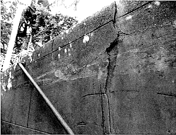
Figure 16. Cracked retaining wall along east property line. (Photograph by Garavaglia Architecture, Inc., April 2015.)
