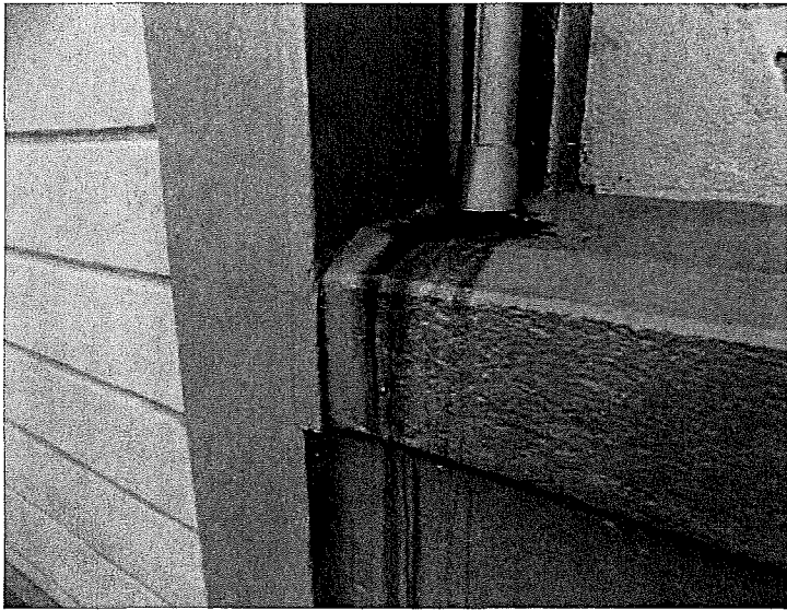
Figure 22. Corroded downspout along north elevation. (Photograph by Garavaglia Architecture, Inc., April 2015.)
