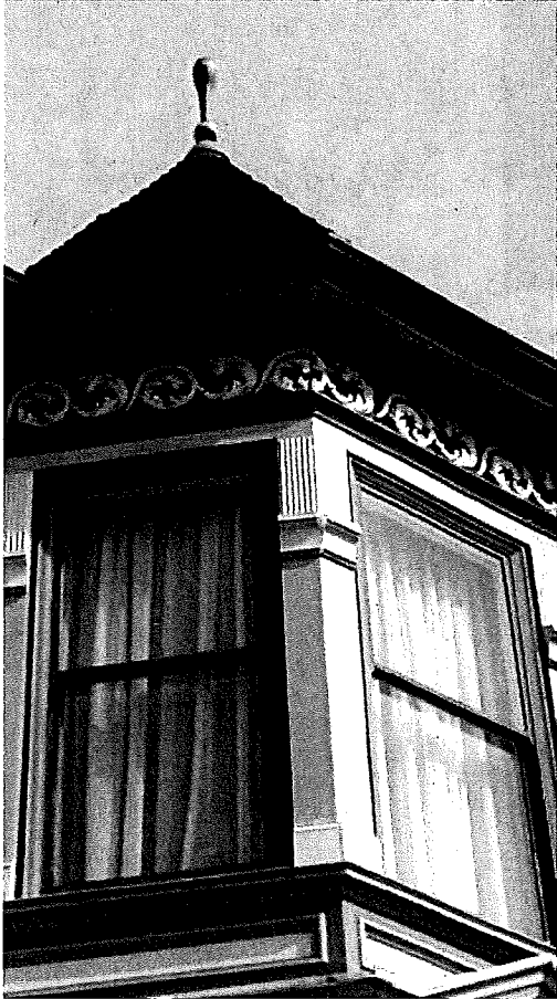
Figure 21. Peeling paint at perimeter fascia. (Photograph by Garavaglia Architecture, Inc., April 2015.)
