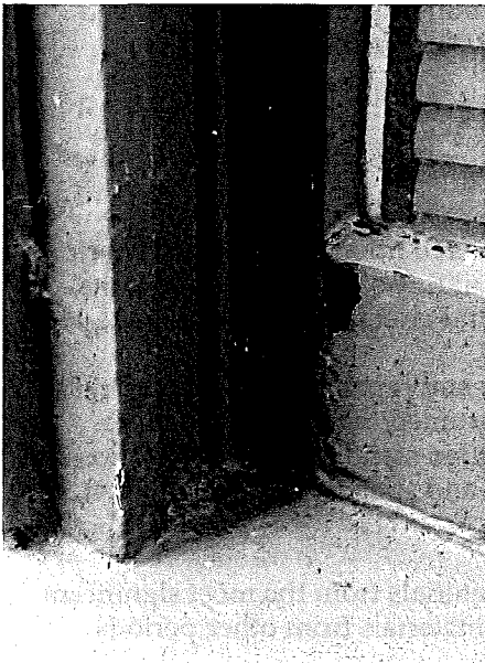
Figure 23. Rotted wood at basement window. (Photograph by Garavaglia Architecture, Inc., April 2015.)
