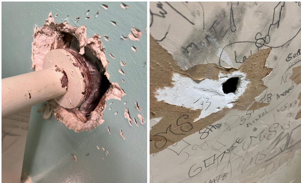
Photos of Damage in County Jail #2, provided by SFSO.
