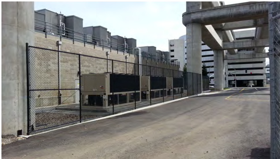
Photo 3C: Airport Data Center (Looking East)
