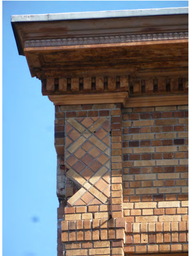
Figure 1. Northwest Corner; note missing facing and decorative brick.
