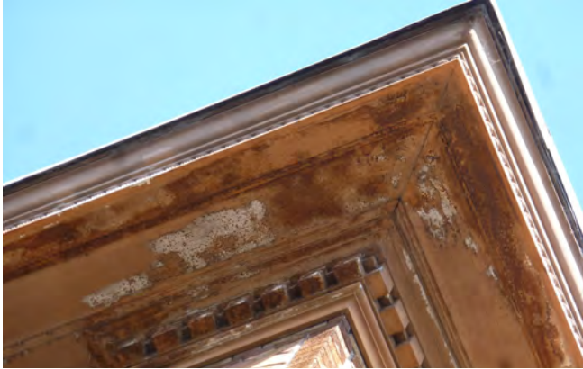
Figure 2. Cornice at southwest corner; note discoloration and localized corrosion, conditions are considered typical.
