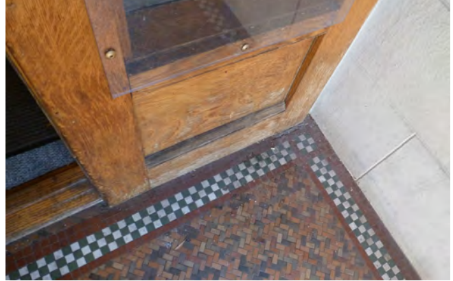
Figure 3: Sidelight at entry door; note replacement of glazing for Plexiglas in response to security concerns.
