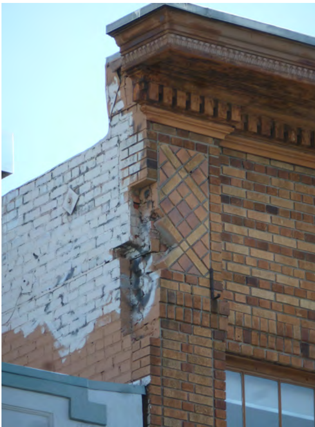
Figure 2. Northwest corner, note missing facing and decorative bricks for replacement.
