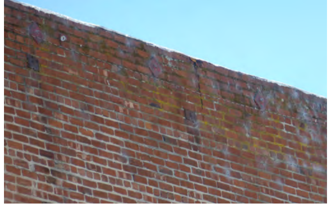
Figure 5. East elevation at roof parapet; note bio-growth and discoloration to be addressed prior to rehabilitation work.
