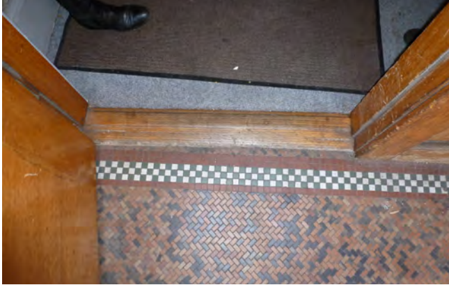
Figure 2. Threshold at wood entry door.
