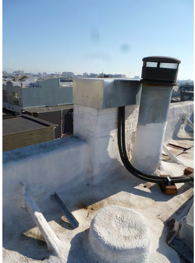
Figure 4. Capped ventilation stack and mechanical exhaust flue; note re-use of ventilation stack for services.
