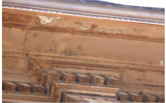
Figure 4. Cornice; conditions noted as typical.
