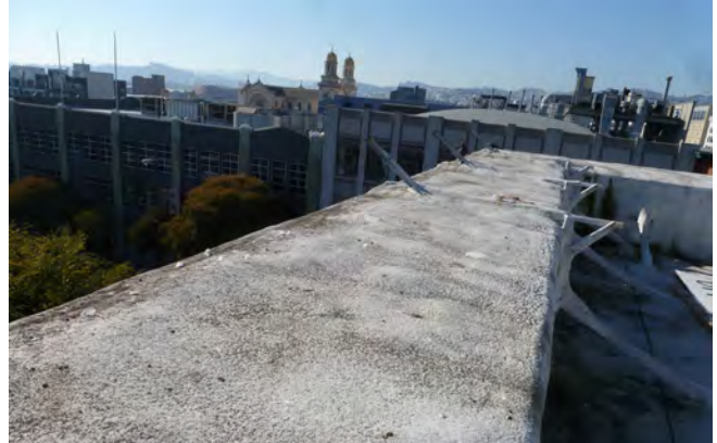
Figure 1. Parapet at southwest corner; note roofing membrane conditions at parapet cap.
