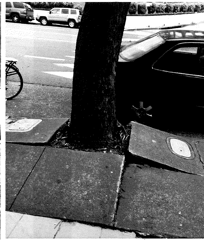
Sidewalk repair needs
