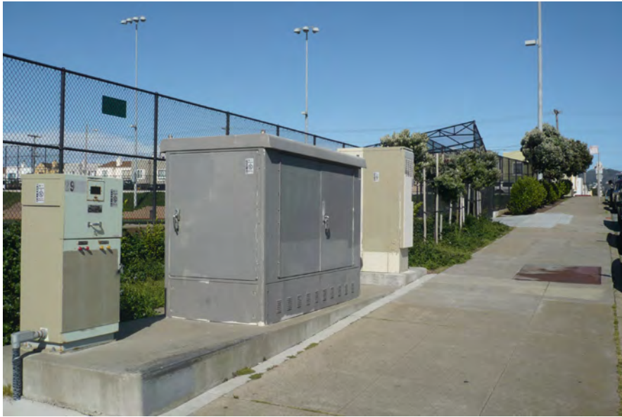
Photo 5 - East-facing View along Wawona Street of South Sunset Playground and Utility Boxes
